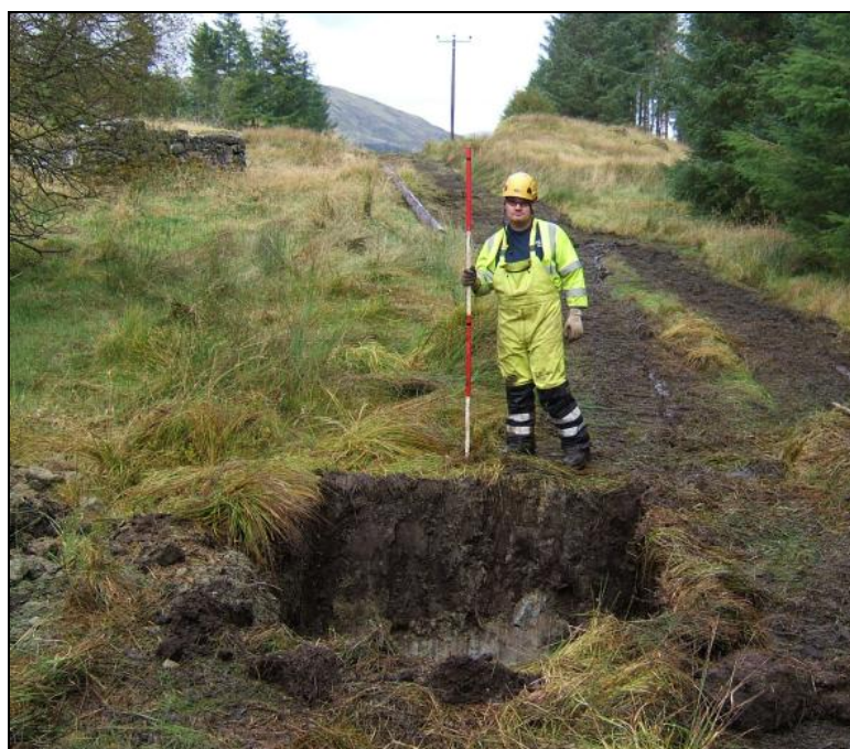
Pole 12 trench with new Pole 13 in the distance, viewed from the south-west
