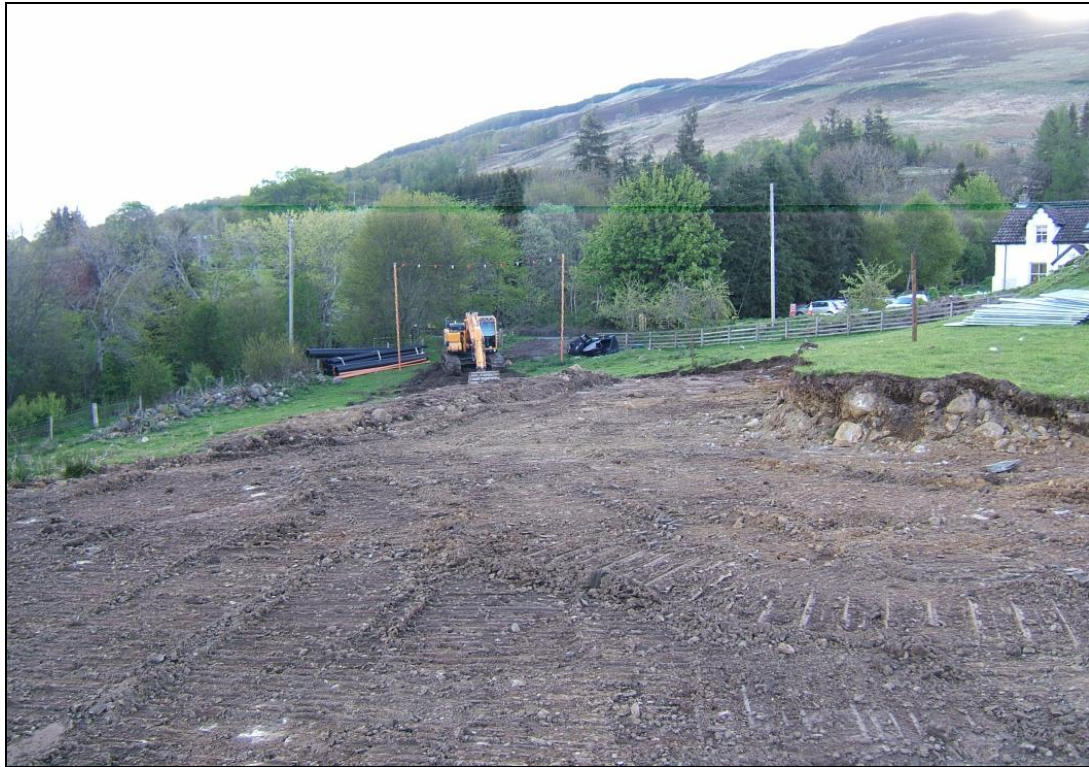
Excavations for the access road from the compound to the public road
