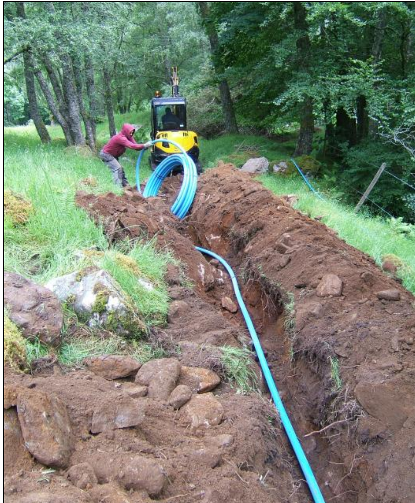
Laying the new pipe midway along the trench, viewed from the north. The edge of the Invervar Burn ravine is on the right
