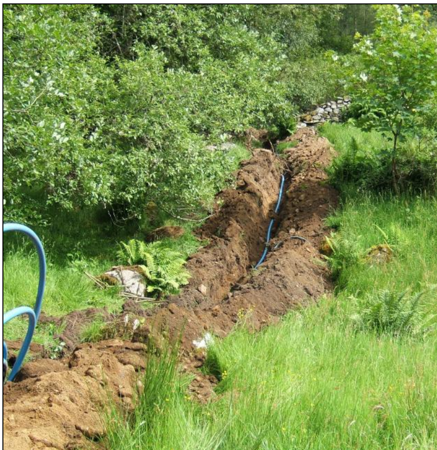
The north end of the pipe trench showing the north boundary wall in the distance
