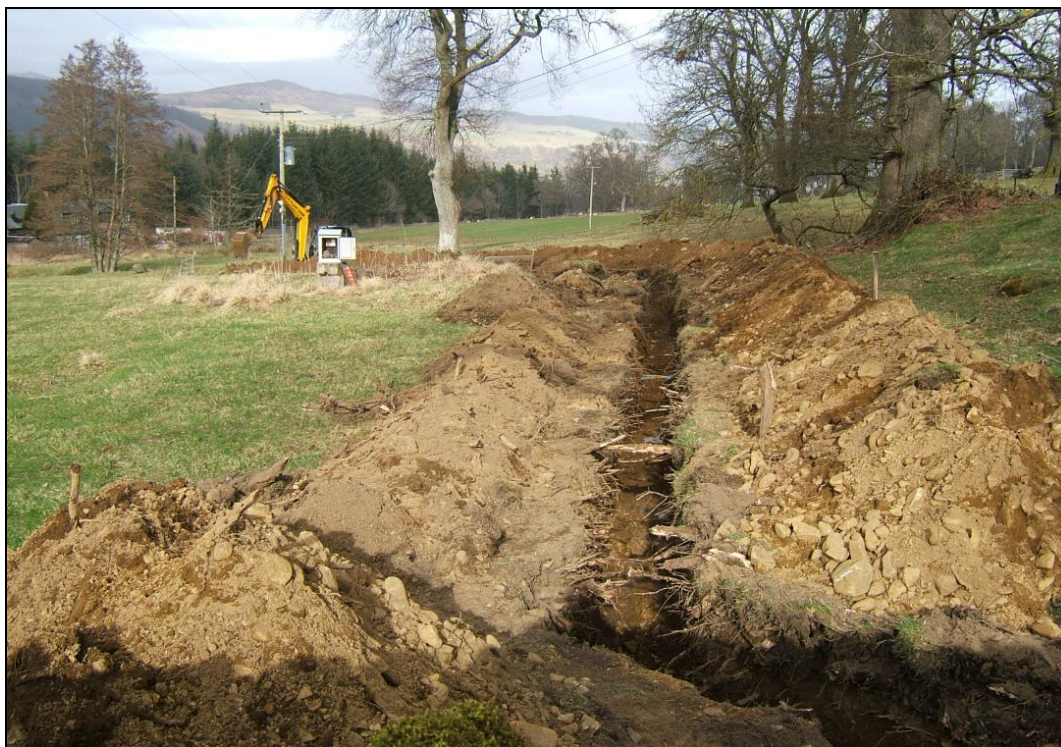
The north-east section of the cable trench with excavation approaching the burn and Pole 38
