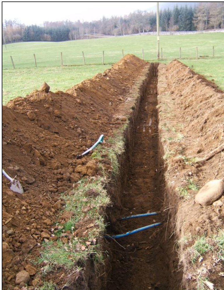
The south-west end of the cable trench, viewed from the north-east. The original Pole 36 is in the distance
