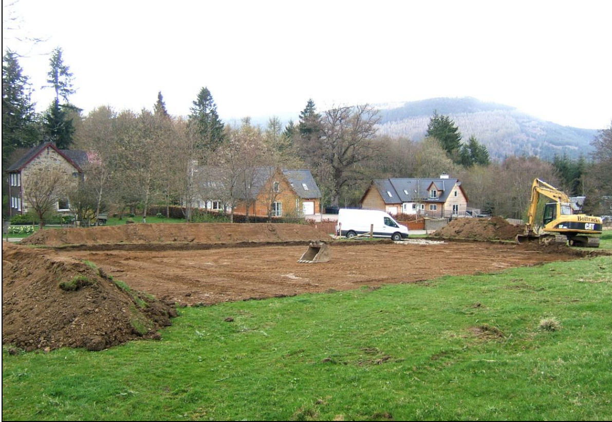
The site stripped of topsoil, viewed from the south. In the background can be seen, left to right, Croftmoraig farmhouse and houses on Plots 1 and 2
