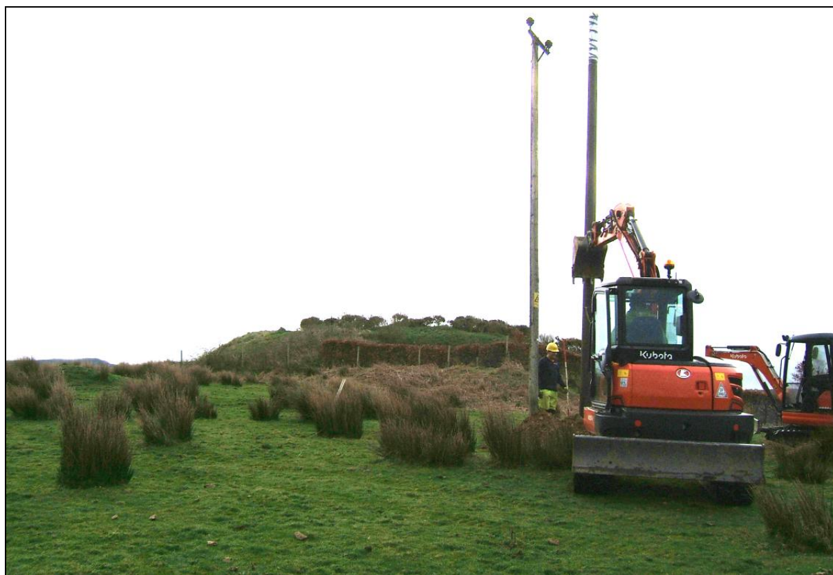
New Pole 72 being inserted. The fort or dun is visible on higher ground beyond. Viewed from the north-west
