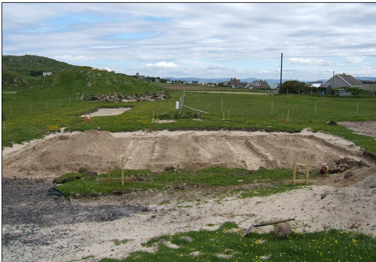
View, from the south-west, of the site following the excavation of the wall trenches
