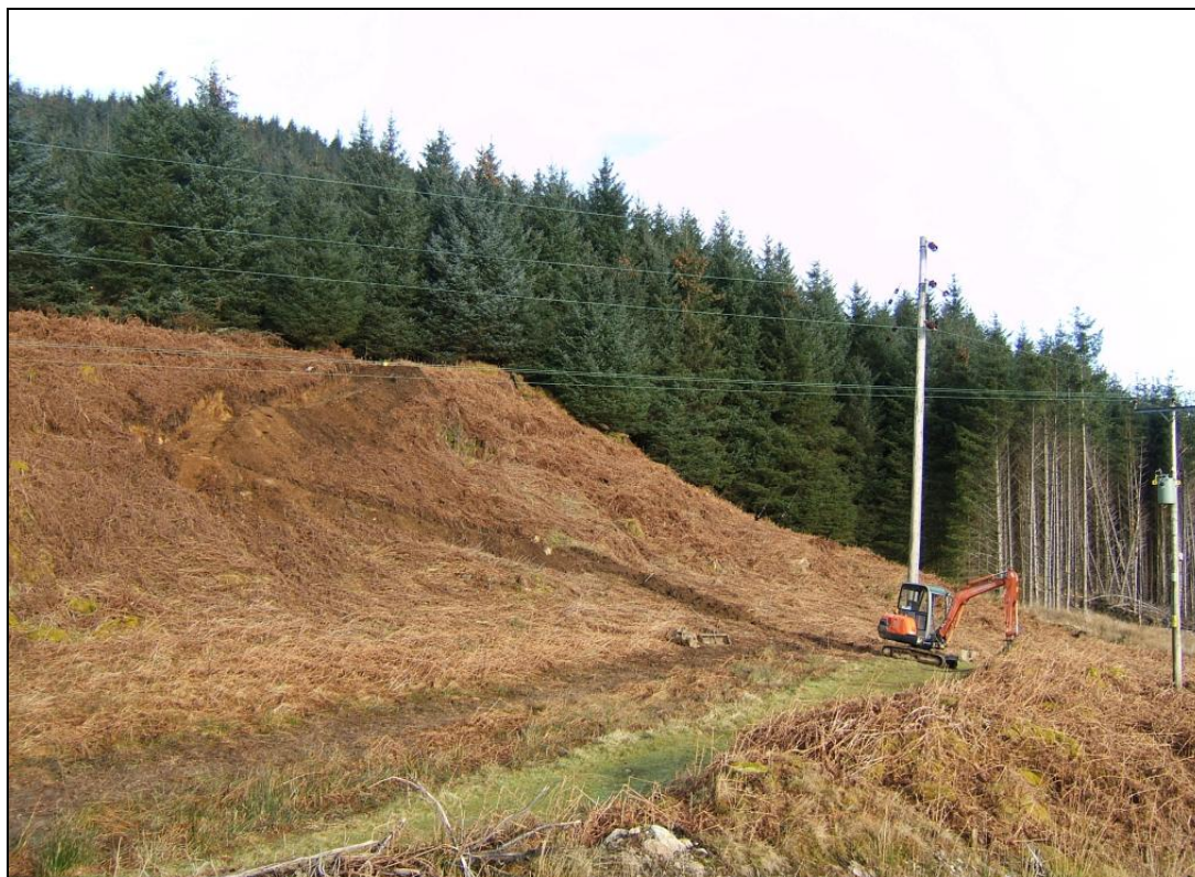
The access track and cable trench on the slope. Pole 27, on the 11kv line, is on the extreme right of the photograph; the 33kv line is adjacent to it
