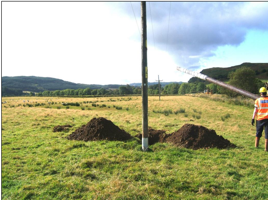
View southwards down Kilmichael glen showing old Pole 36 and the trench for the new one just beyond
