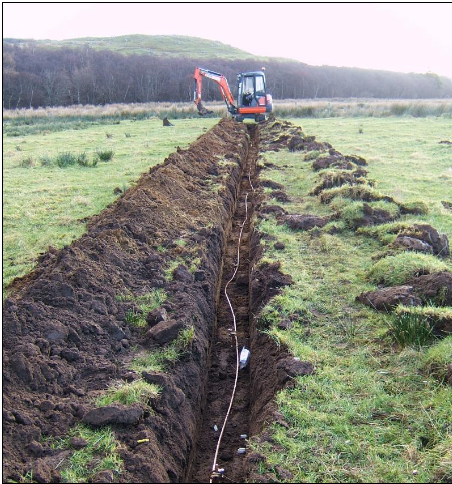
Trench at Pole 85 showing copper earth wire and attached copper rods, viewed from the west
