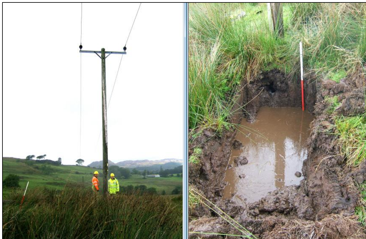
Old Pole 1 showing the result of lightning strike, viewed from the south
