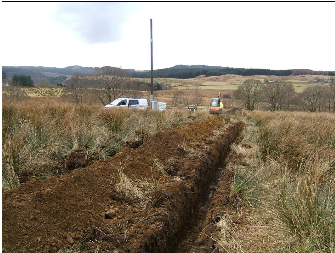
The south-west end of the trench with the new mast in the middle distance
