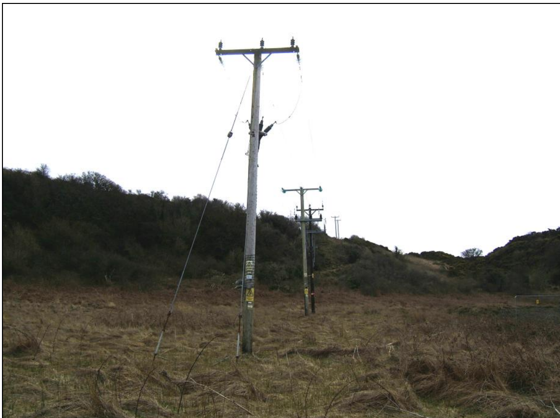
View to the south-east of the overhead line as it climbs the old cliff. Pole 13 is in the foreground
