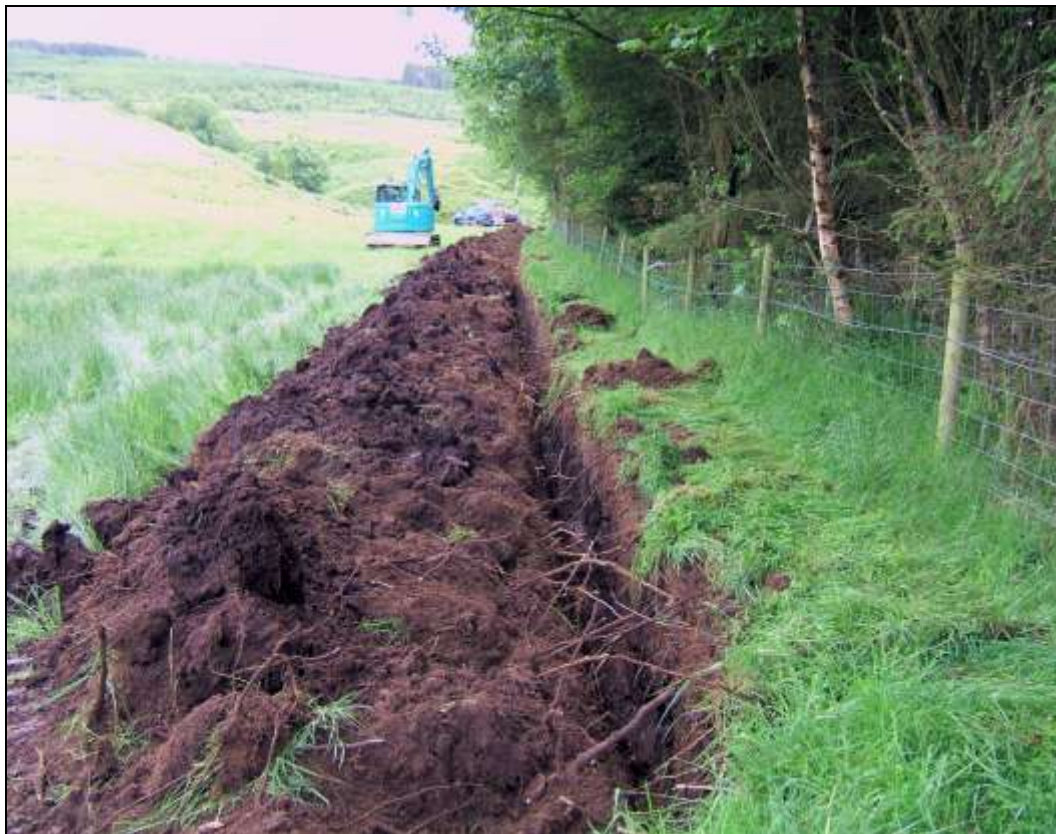
Cable trench from the north-west
