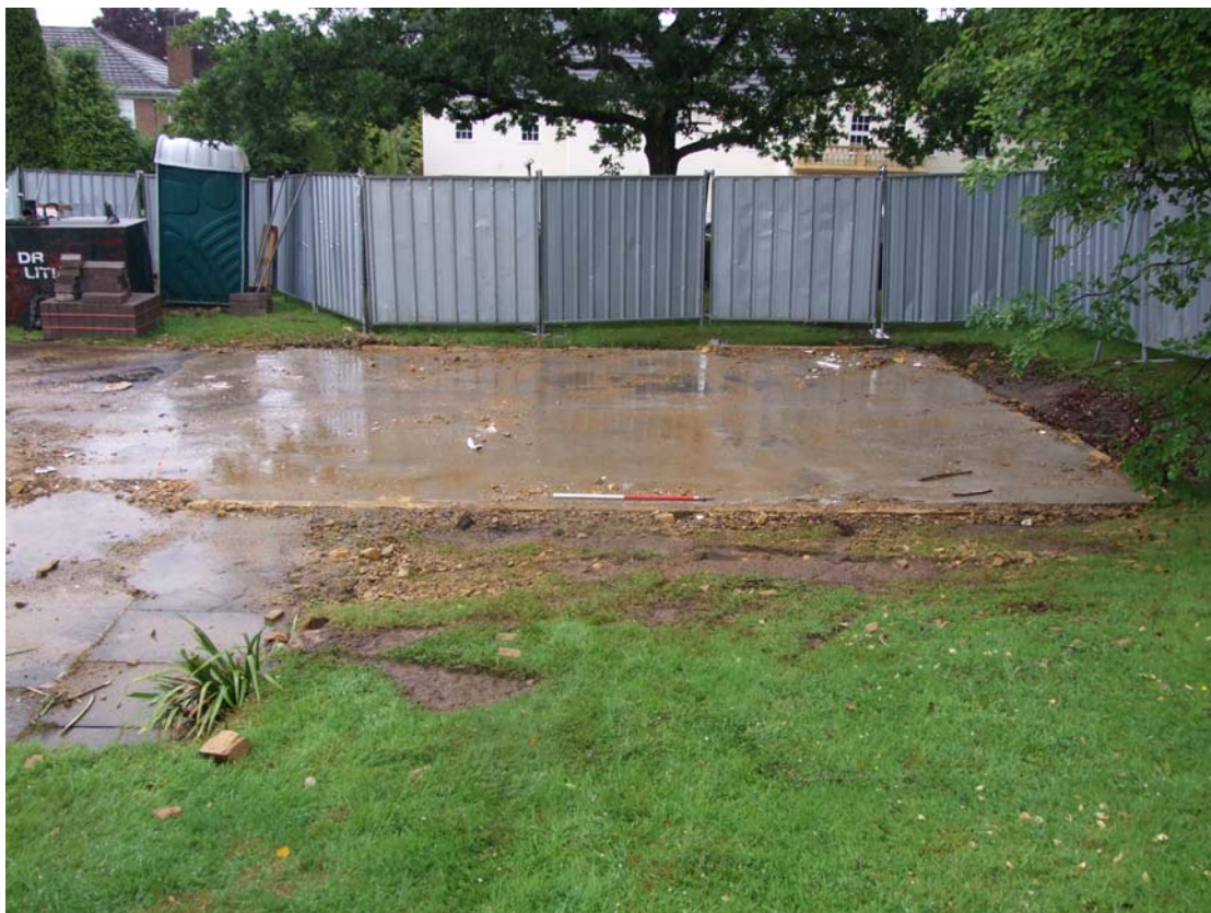
Fig 6 Timberlee: view to the east showing the ground slab of the garage prior to its removal (Area C)
