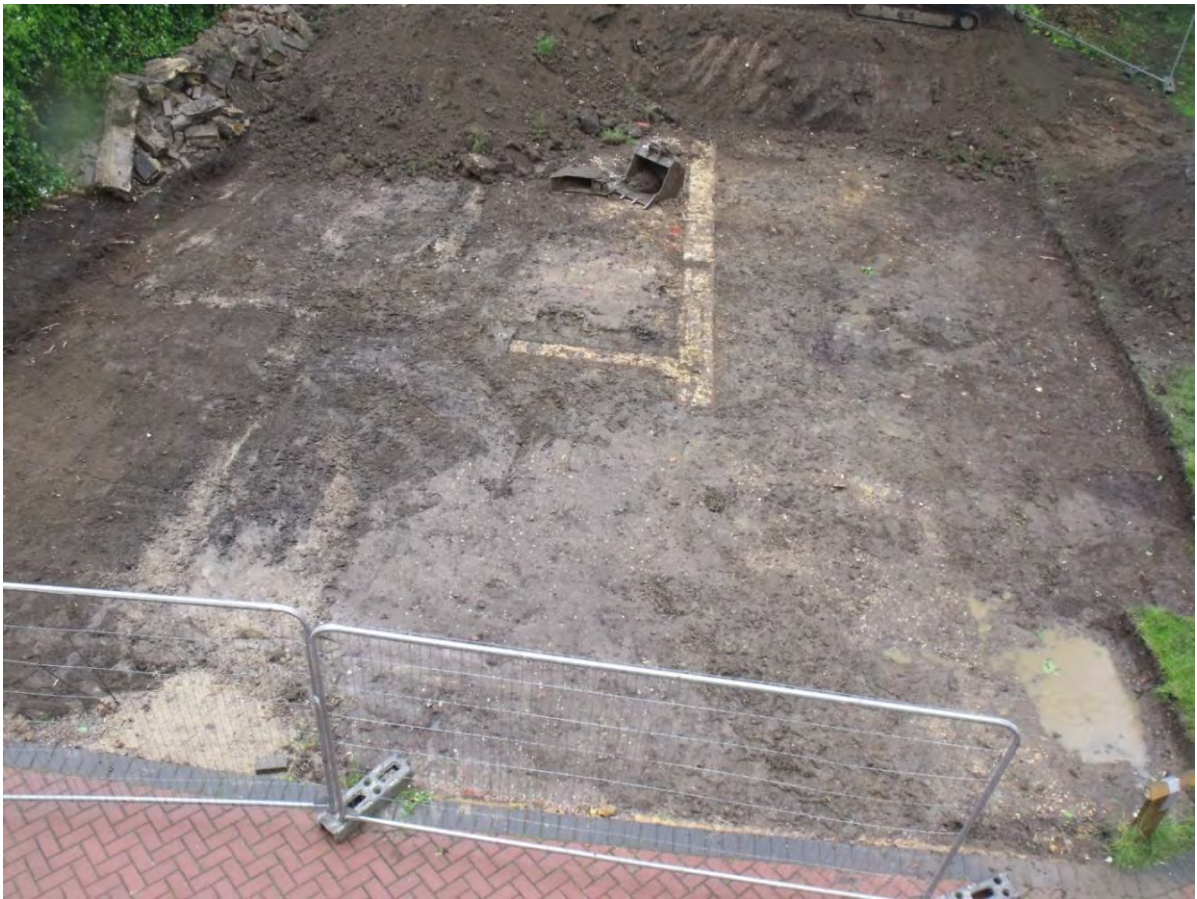
Fig 14 Reigate Priory Junior School, Reigate; progress shot of area strip, view to the west.
