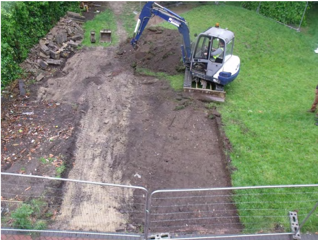
Fig 6 Reigate Priory Junior School, Reigate; removing topsoil, sand delineates line of modern pathway. View to west.
