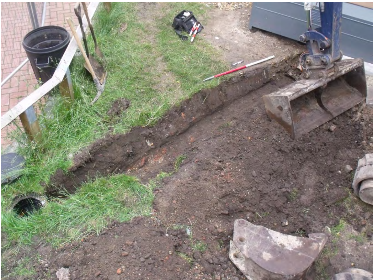
Fig 15 Reigate Priory Junior School, Reigate; drainage pipe spur trench, view to the southeast.
