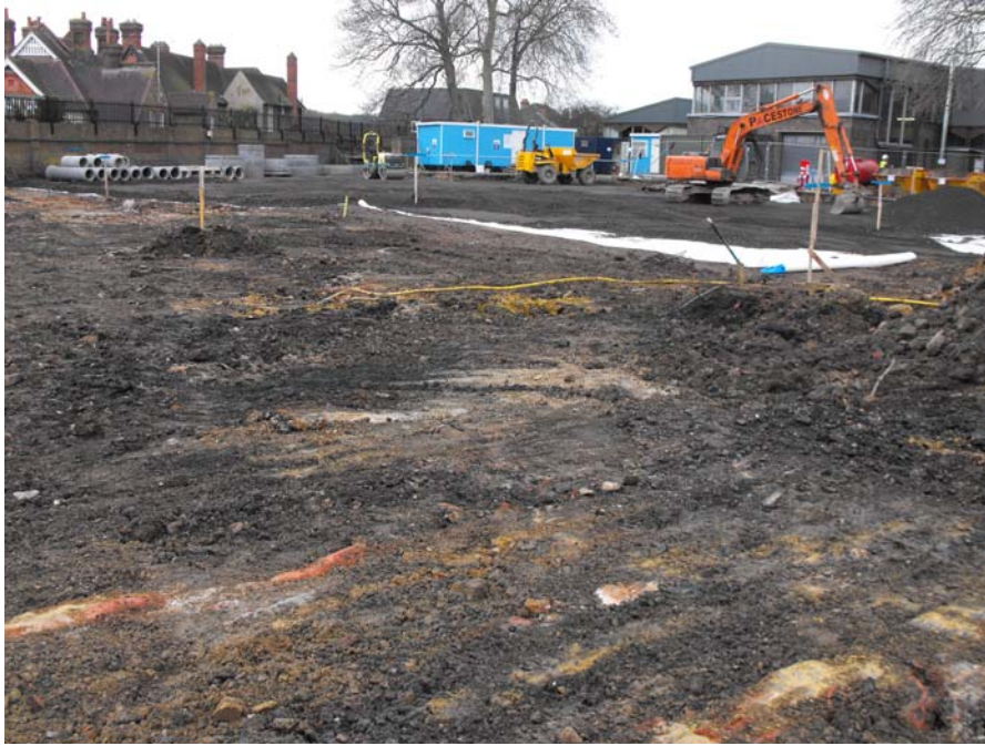
Fig 10: Area B looking south west, showing exposed foundations of building and area re-covered with membrane and crush
