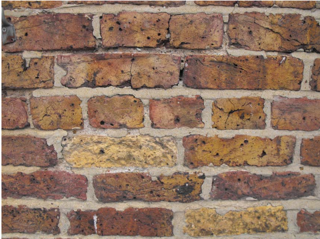
Fig 32: Detail of brickwork on the exterior of the covered riding arena, showing marbled colouring, uneven sizing and large voids.
