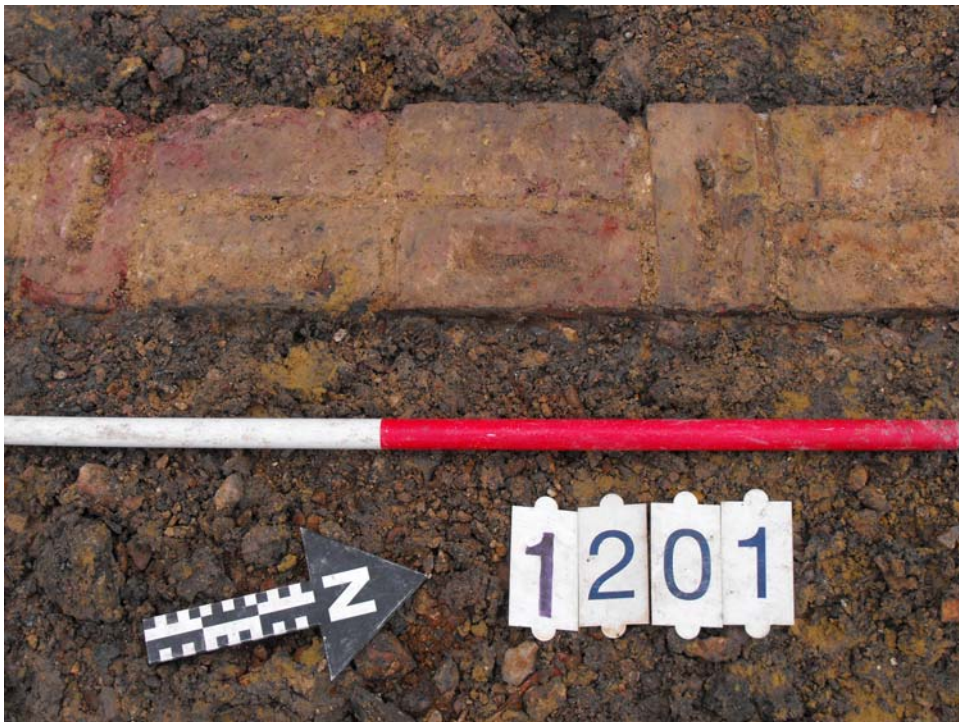
Fig 31: Detail of wall at south end of veranda, showing alternating header/stretcher pattern
