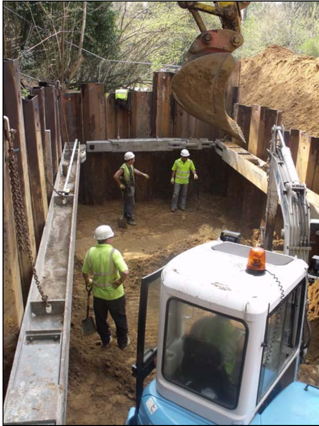
Fig 9 Klargester sewage pit
