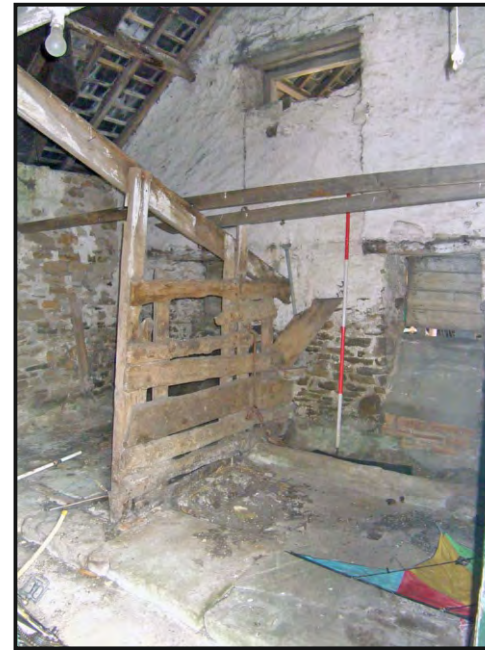
Photo. 34: View towards the internal south wall of the central compartment of the east range, with openings to entrance corridor, byre division and part-flagged floor.
