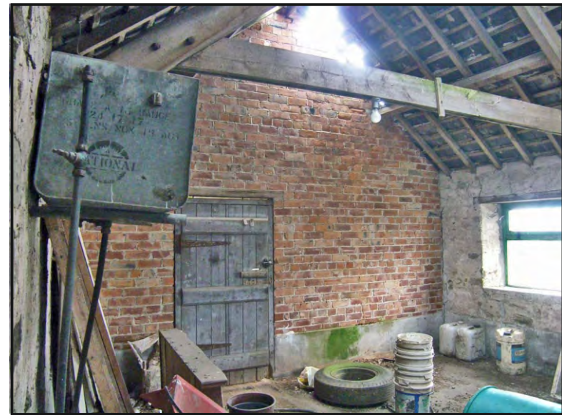
Photo. 30: View from the south-east of the internal west wall of the south range, first floor.
