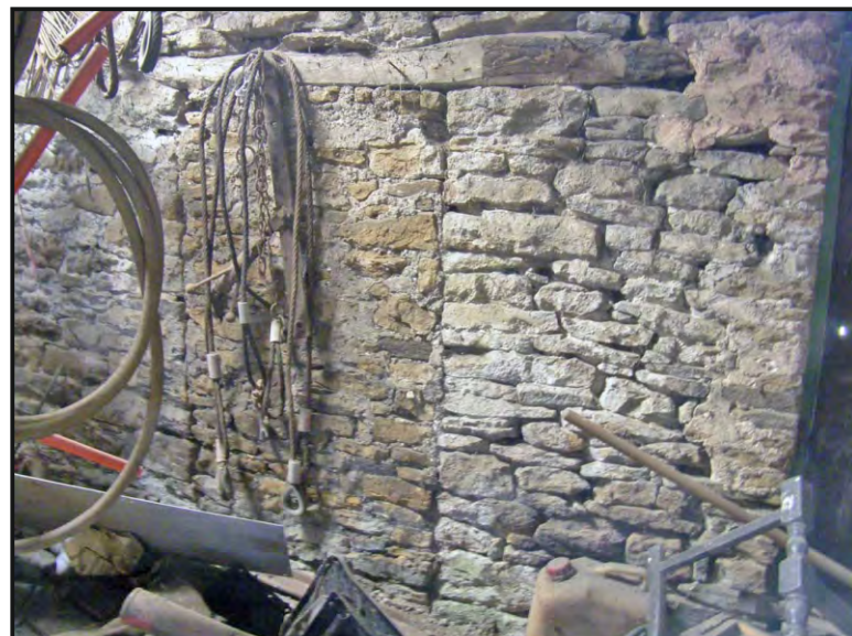
Photo. 39: Detailed view of a blocked opening at the north end of the west wall of the south-east building interior.
