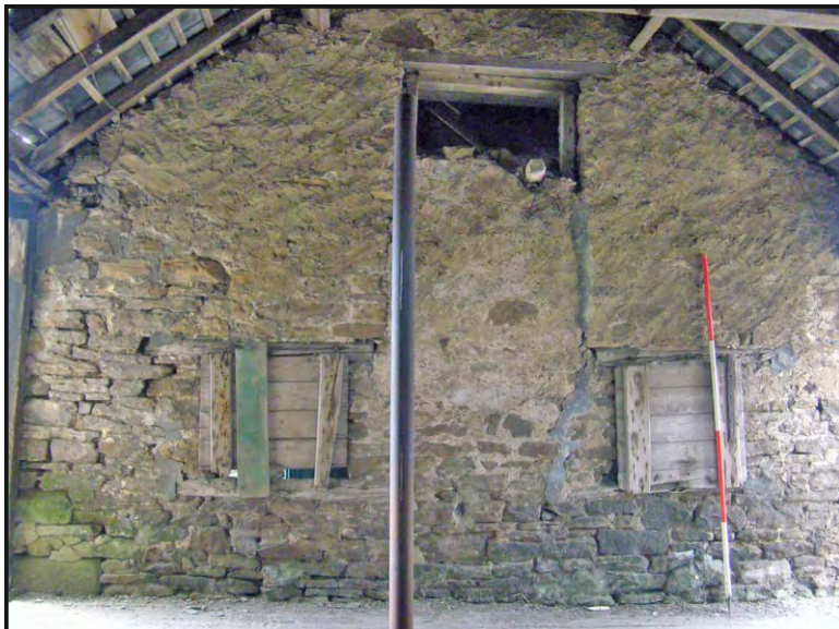
Photo. 35: View from the south side of the south compartment of the east range, showing openings in an internal dividing wall which forms the north side of an entrance between opposed doorways in the east and west sides of the range.
