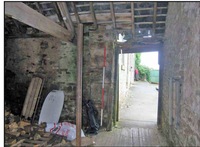
Photo. 36: View westwards from within the south compartment of the east range towards the west doorway into the range.
