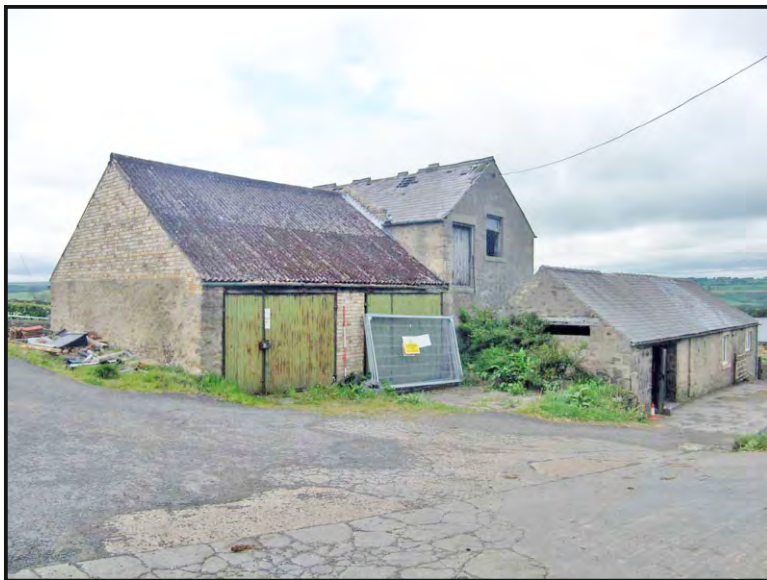
Photo 11: View from the south-east of the farm-buildings complex, with the south-east building, the probable engine house with its early 20th century brick gable in the foreground, and the south gable end of the East Range to the right.
