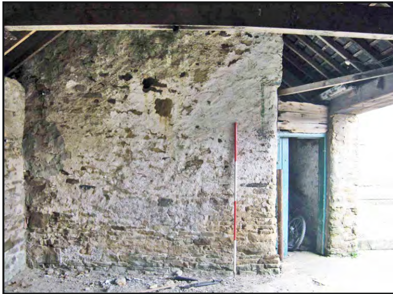
Photo. 33: The internal south wall of the north compartment of the east range.
