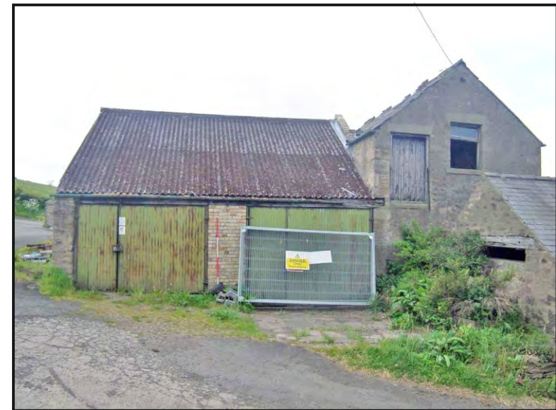
Photo 12: The east elevations of the south-east building (left of view) and south range.
