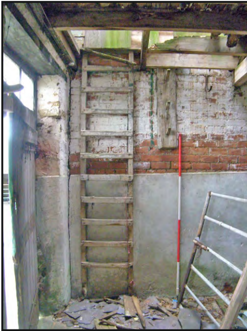
Photo. 25: View to the east wall of the west-central compartment of the south range.
