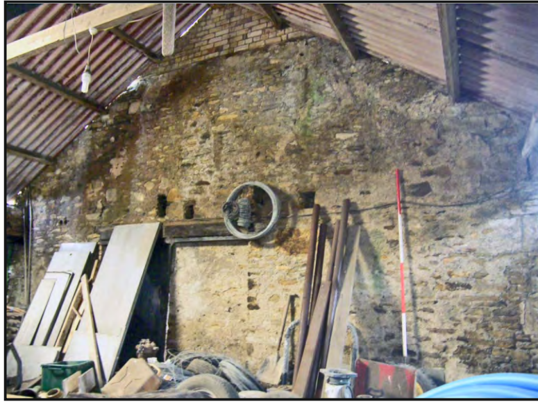
Photo. 37: View from the south-east within the south-east building of the south elevation of the east range.
