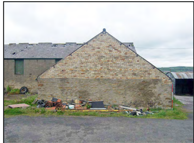
Photo 10: South elevation of the south-east building, attached at the east end of the south range.
