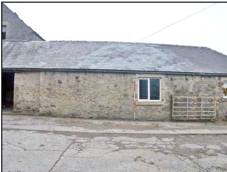
Photo 15: The middle and north parts of the east elevation of the east range.
