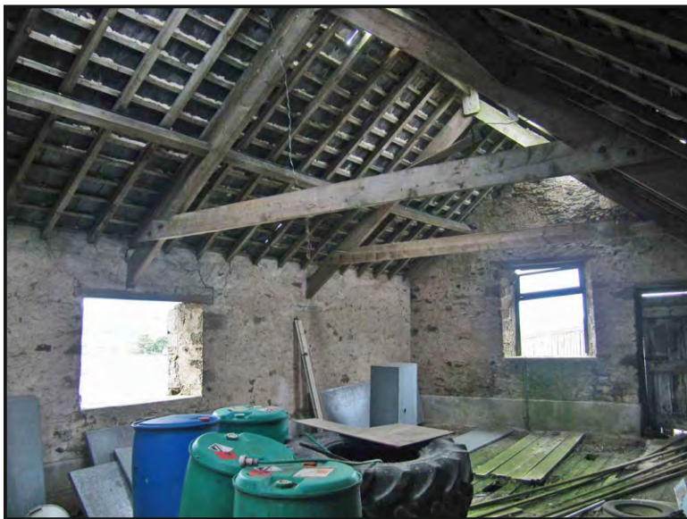
Photo. 31: View from the south-west of the internal east wall and east end of the north wall of the south range, first floor.
