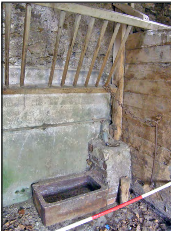
Photo 23: Close-up view of water trough and other fittings against the south wall of the west compartment of the south range.
