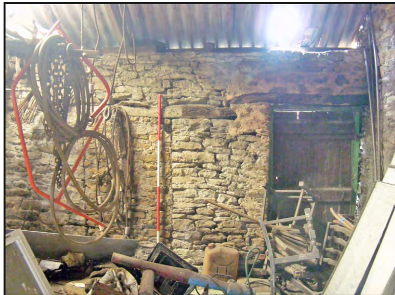
Photo. 38: Doorway and adjacent blocked opening at the north end of the west wall of the south-east building interior.
