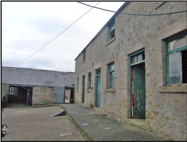
Photo 21: View eastwards from the west end of the south elevation of the south range, towards the east range.
