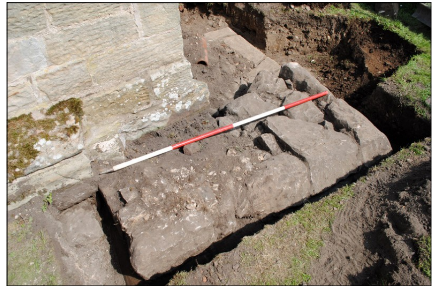
Illus. 44: View looking southeast across completed excavation of Tower foundations adjacent to the southwest corner of the Nave.
