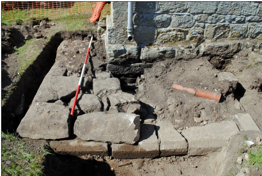
Illus. 40: View looking north across completed excavation of Tower foundations adjacent to the southwest corner of the Nave.
