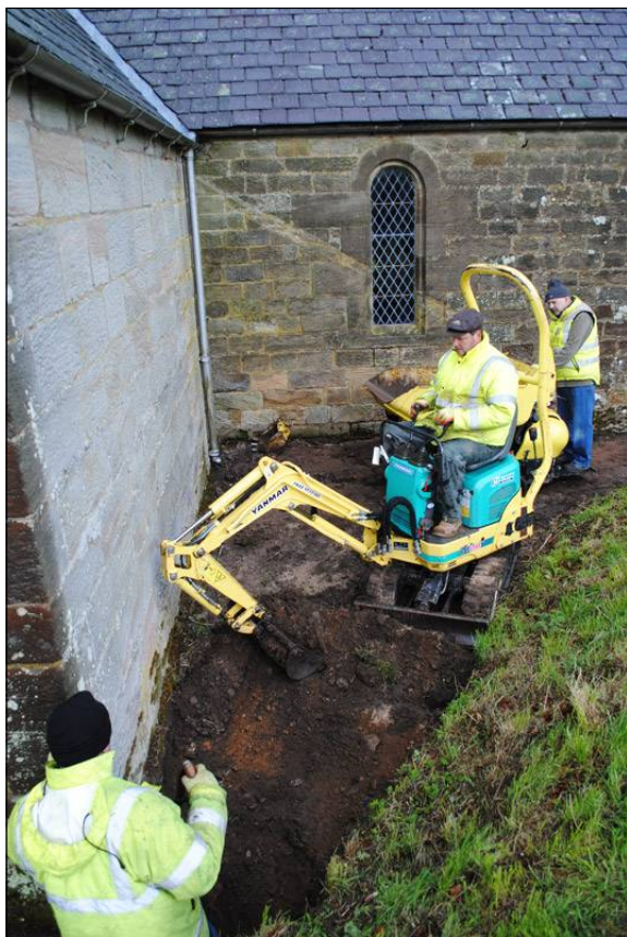
Illus. 21: View looking south along services trench between north transept and north nave wall.
