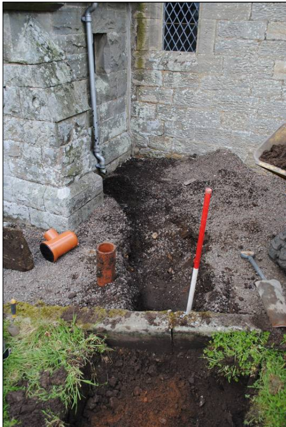
Illus. 31: View looking northwest at services trench, running from the northeast corner of the porch across the footpath.
