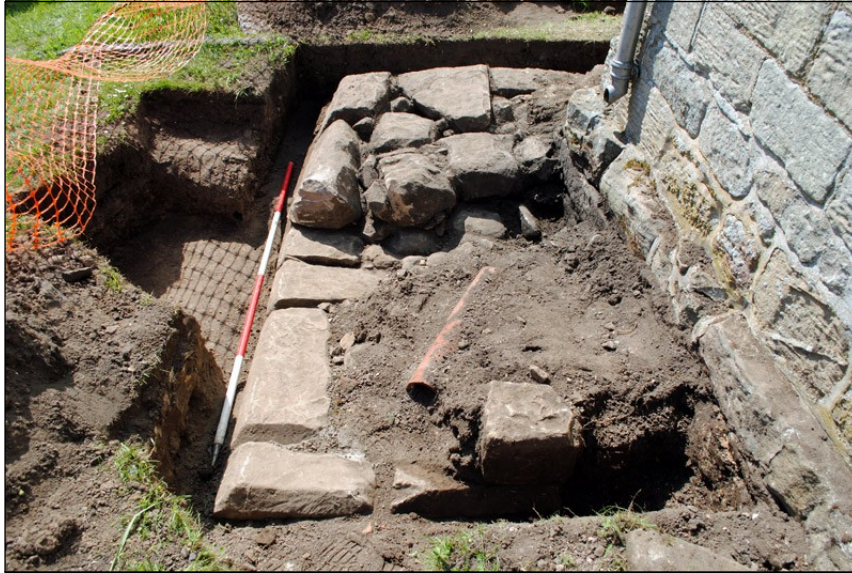
Illus. 42: View looking west across completed excavation of Tower foundations adjacent to the southwest corner of the Nave.
