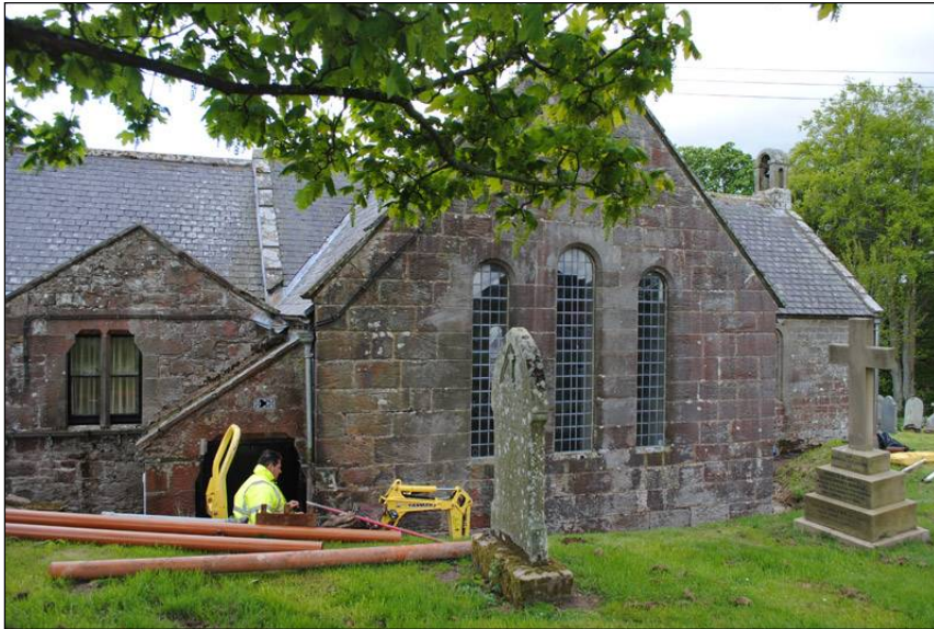
Illus. 16: View of Bolton Chapel, looking south at the start of works.
