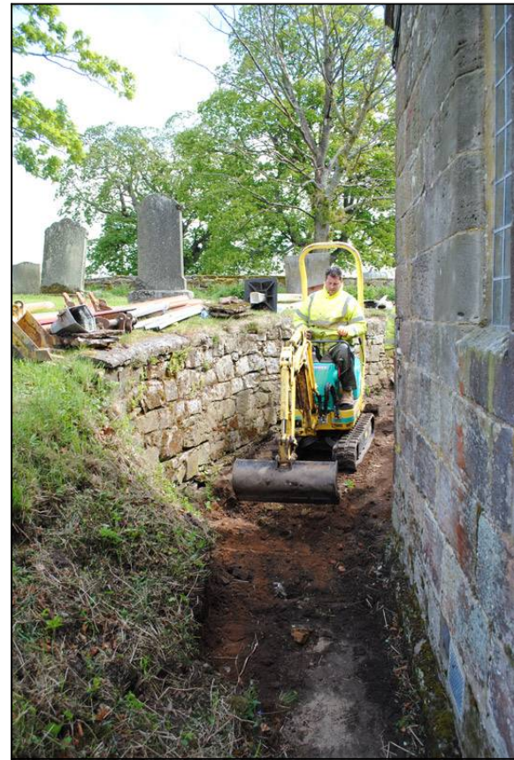
Illus. 17: View looking east along the north side of the chapel during initial clearance of vegetation and turf for services trench.
