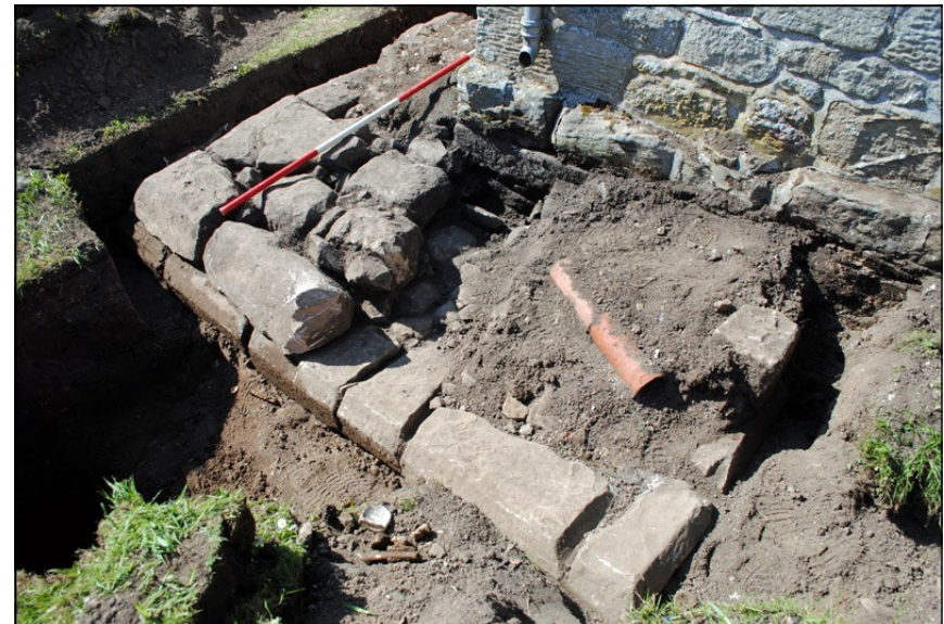
Illus. 41: View looking northwest across completed excavation of Tower foundations adjacent to the southwest corner of the Nave.
