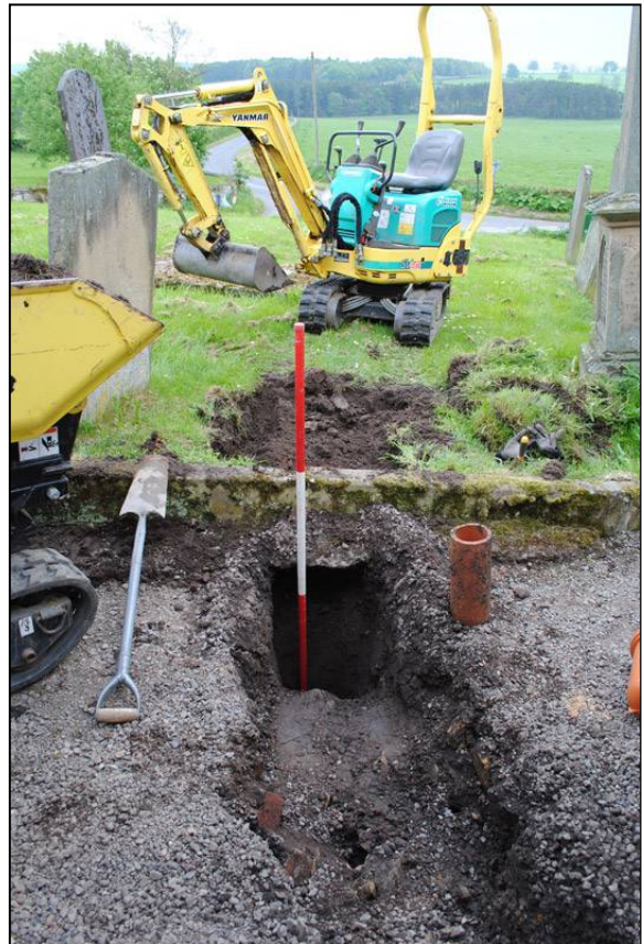
Illus. 32: View looking south at services trench, running from the northeast corner of the porch across the footpath.
