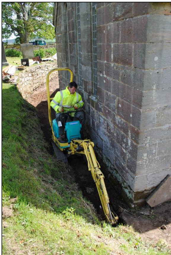
Illus. 18: View looking east along the north side of Bolton Chapel during excavation of services trench.
