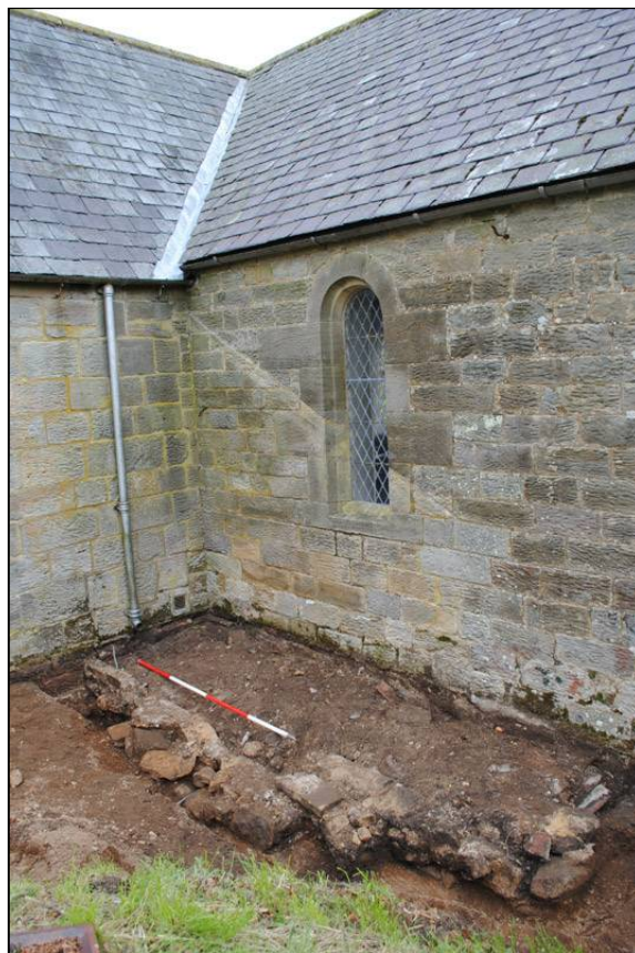
Illus. 22: View looking southeast at structural remains at intersection of the north transept and north nave wall.
