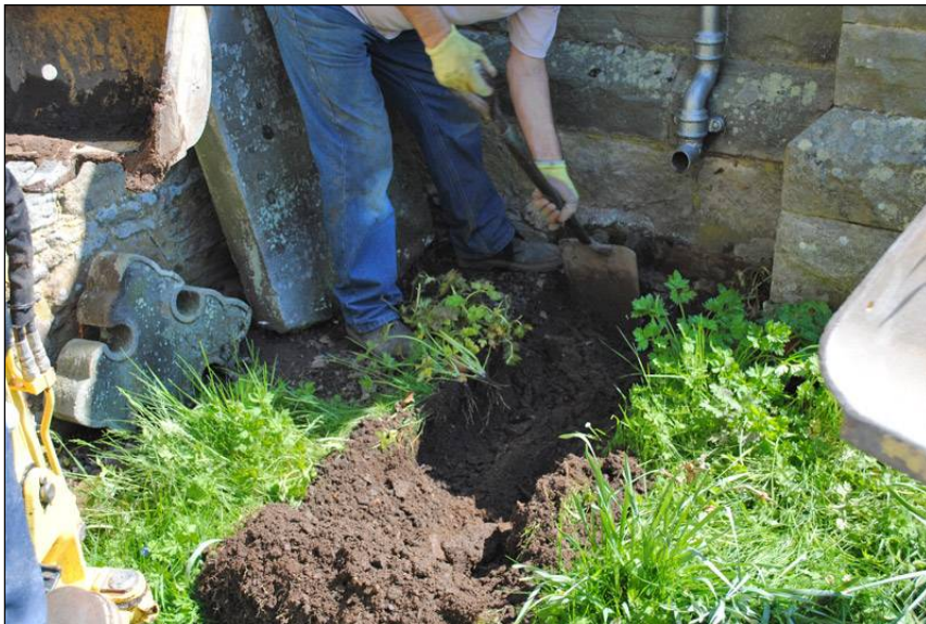
Illus. 34: View looking east at detail of services trench running from the west wall of the porch.
