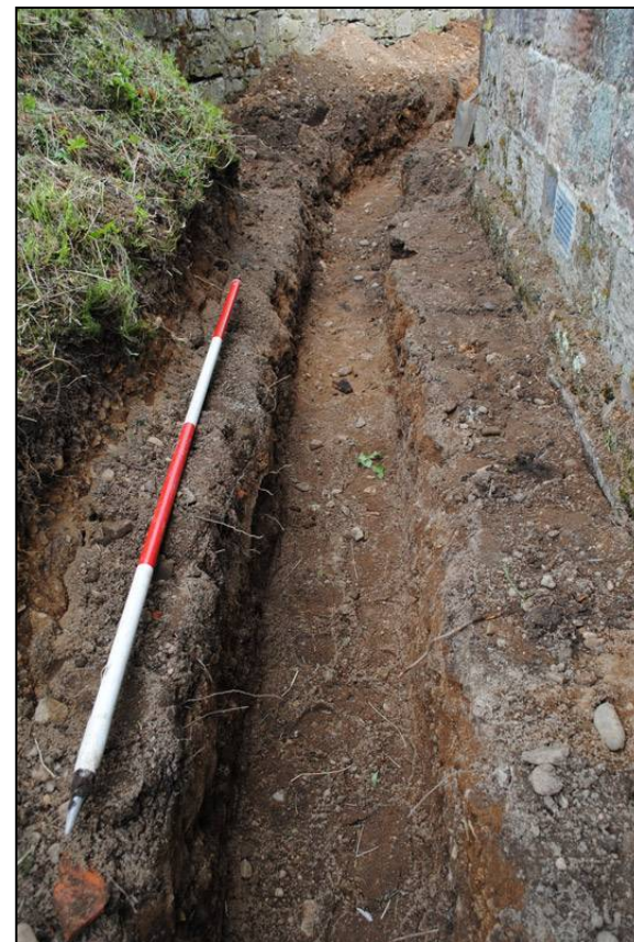
Illus. 20: View looking east along the services trench on the north side of Bolton Chapel.
