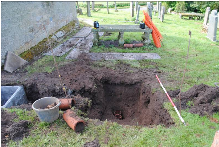
Illus. 28: View looking south at excavated soak-away pit, adjacent to the northwest corner of the nave.
