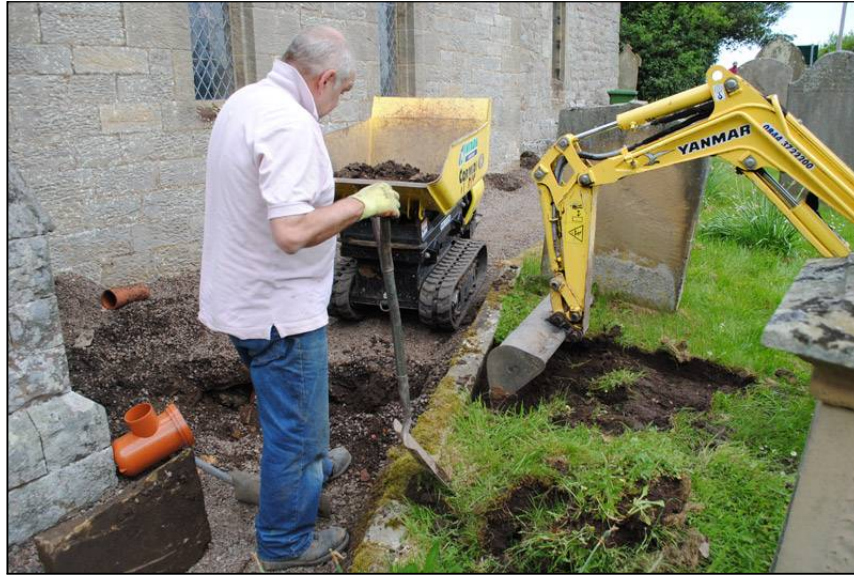
Illus. 30: View looking east during excavation of services trench and soak-away pit, running from the northeast corner of the porch turning southwards and bisecting the footpath.
