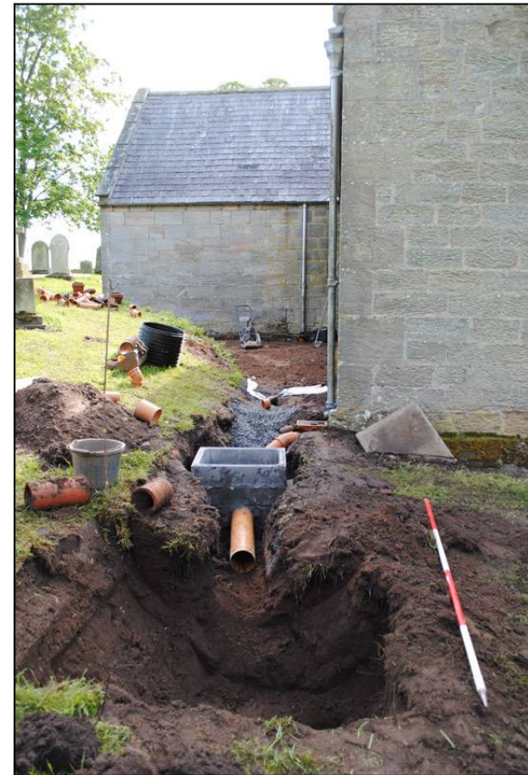
Illus. 29: View looking east at excavated soak-away pit, adjacent to the northwest corner of the nave.
