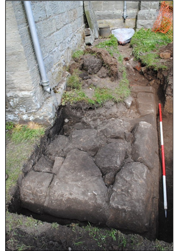
Illus. 38: View looking east along Tower foundations adjacent to the southwest corner of the Nave.
