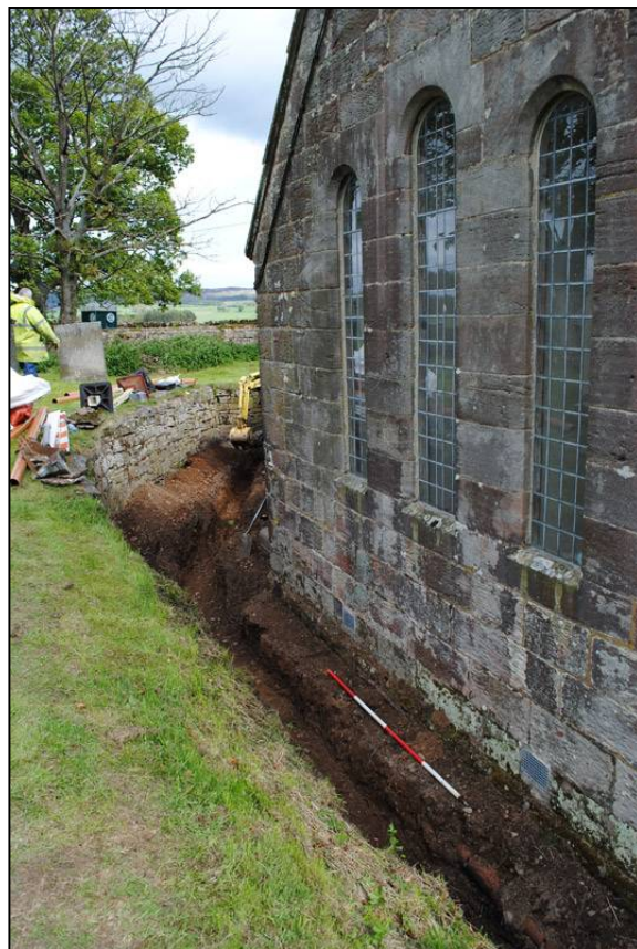
Illus. 19: View looking southeast along the services trench on the north side of Bolton Chapel.
