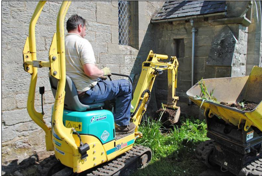
Illus. 33: View looking northeast during excavation of services trench from the west wall of the porch.
