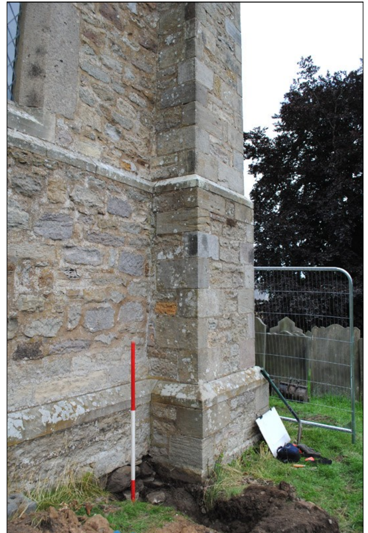
Illus. 13: View looking north-east towards Trench 1 and the south-east corner of the Chancel.
