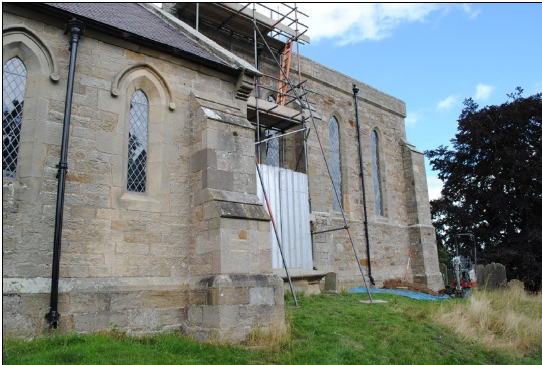
Illus. 12: Wide view looking north-east towards Trench 1 and the south-east corner of the Chancel.
