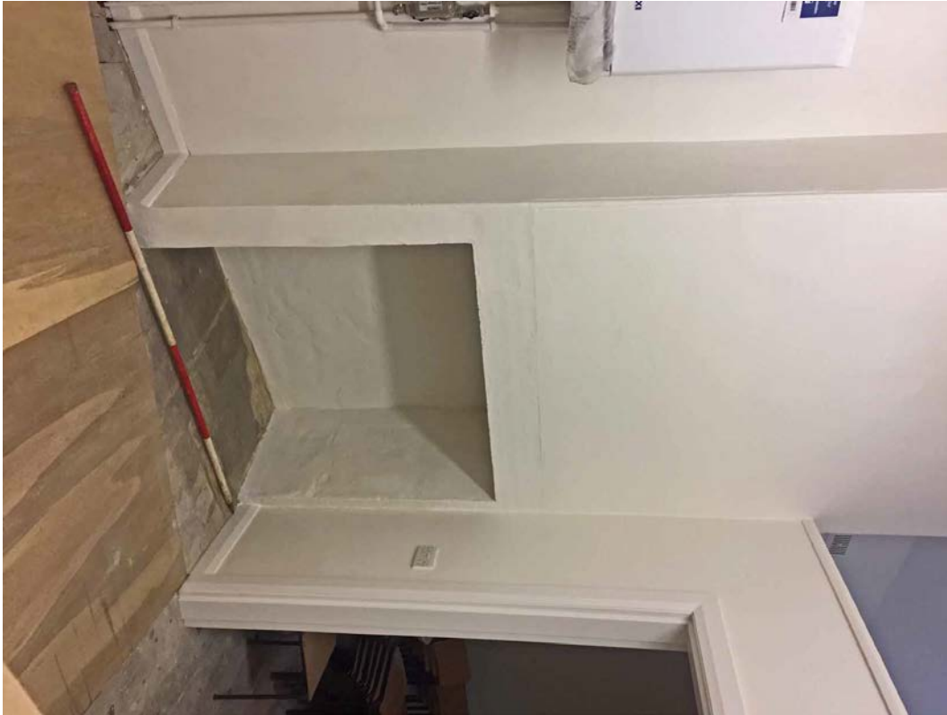
13 (Bottom to left of view): Redundant chimney breast on the east side of the Porch Block (kitchen area), viewed from the north-west.
