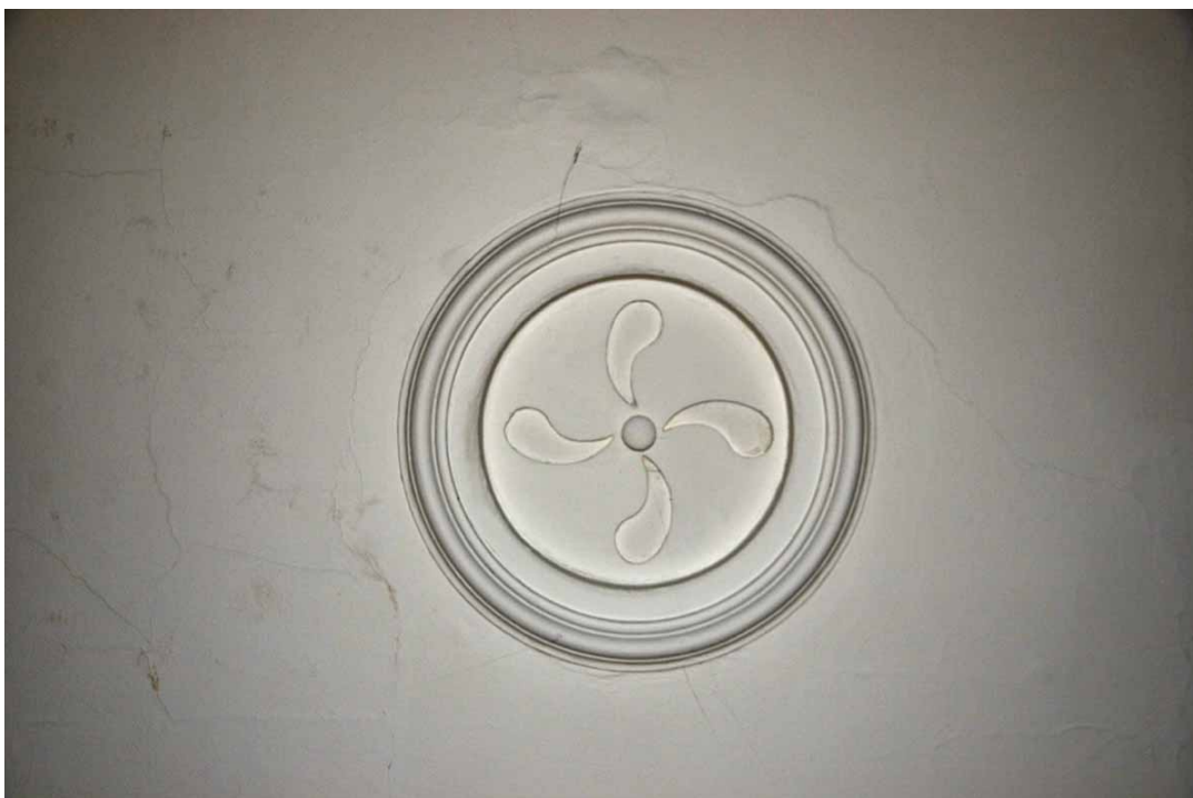
07: Ceiling ventilator In main chapel
