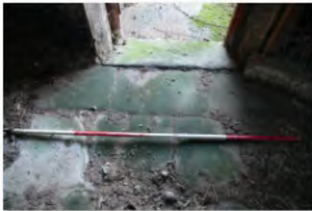
76 SE Range N compartment door threshold
