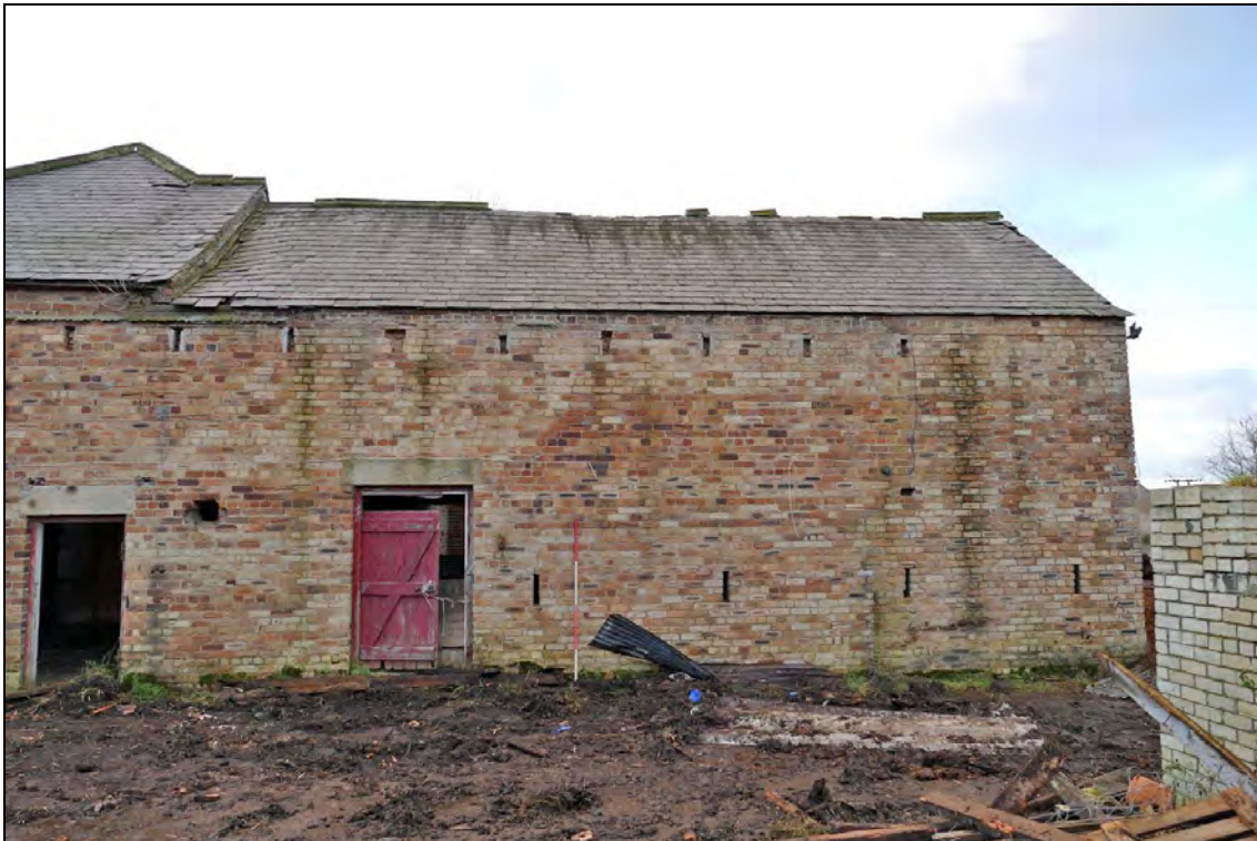
Illus. 20: The Northern Part of the West Range, view of the east side.
