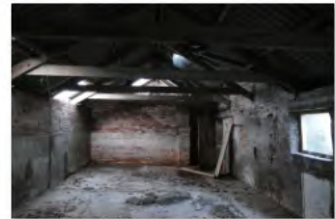
90 W Range S part S compartment looking N
