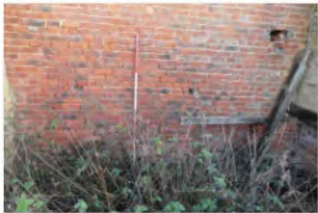
106 Engine House blocked door on W
