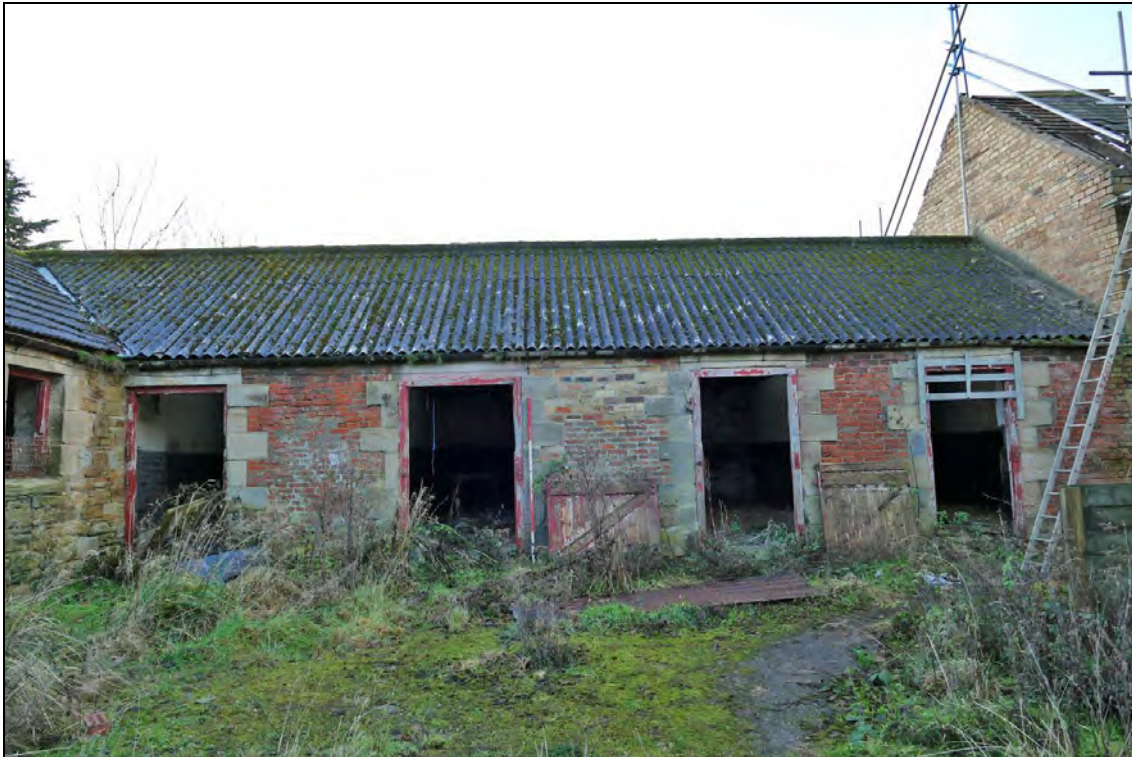
Illus. 19: The Southern Part of the West Range, viewed from the south yard.
