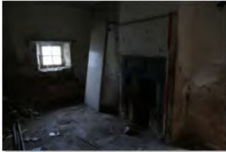
73 SE Range centre compartment fireplace
