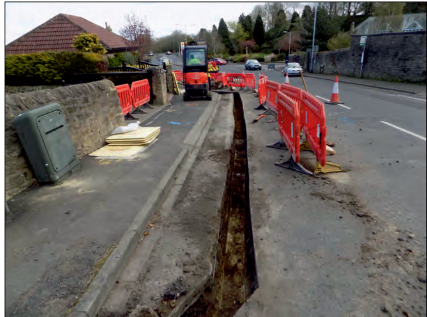
Photo 8. General working shot during cable trenching, view looking east along Hexham Road.
