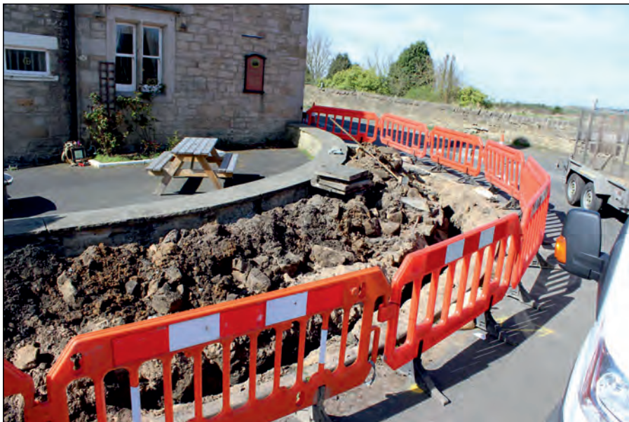
Photo 3. View looking northwest across cable trenching located towards the northeast corner of the Three Tuns Inn.
