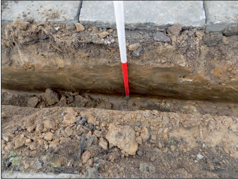
Photo 5. South facing section of cable trench, located approx 5m from start of trench.
