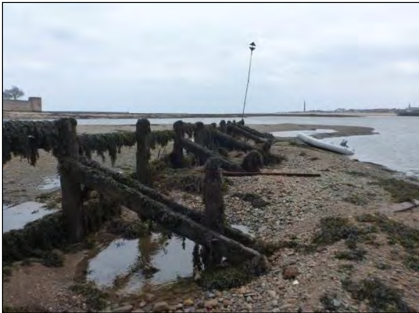
Frontispiece: Part of the groyne structure on the south side of the dock entrance
