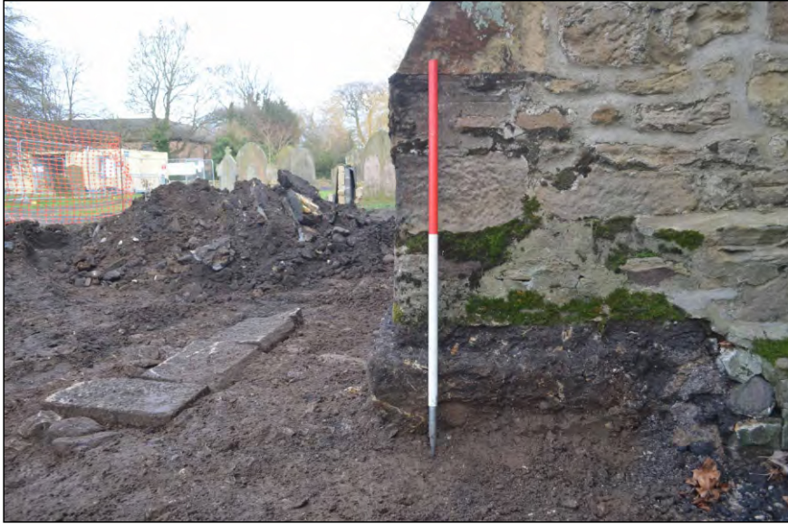
Photo 39. Exposed foundation of western buttress along the north wall of the church. View looking east.
