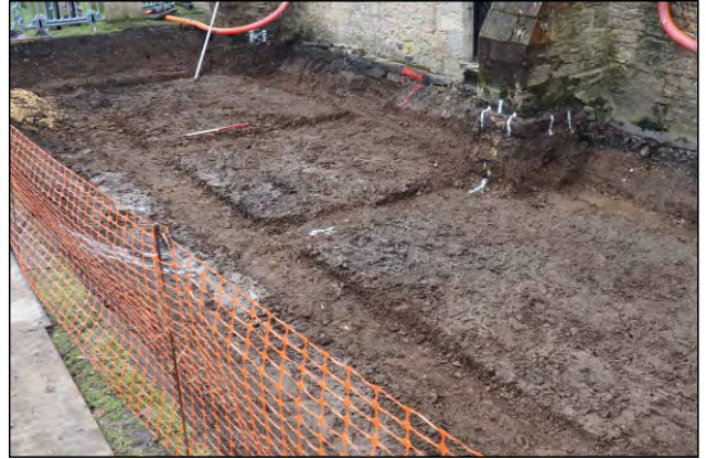
Photo 48. Completed trenching for the foundation pad of the new extension. View looking SE.
