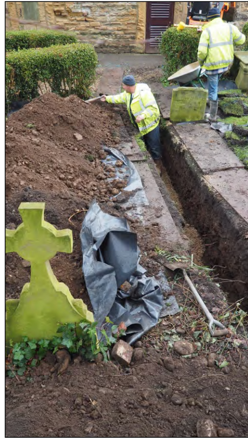
Photo 77. View looking east along services trench excavated from Vicarage garden to Church east end.
