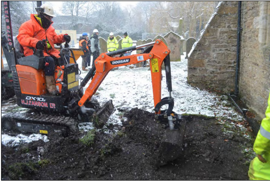
Photo 31. View looking east at the beginning of excavations for the foundation pad of the new extension.
