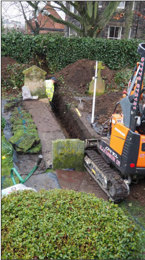
Photo 76. View looking west along services trench excavated from Vicarage garden to Church east end.
