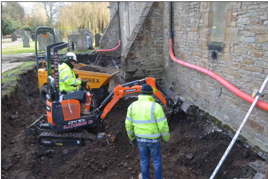
Photo 45. Further ground reduction to the west of the western buttress along the church north wall. View looking east.
