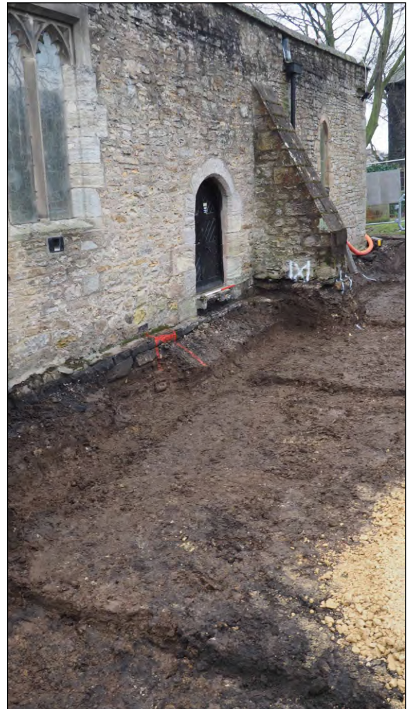
Photo 50. Completed trenching for the foundation pad of the new extension. View looking SW.
