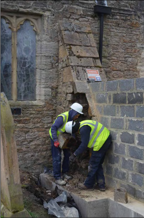
Photo 82. The eastern buttress during removal of facing stones on east side of front elevation.
