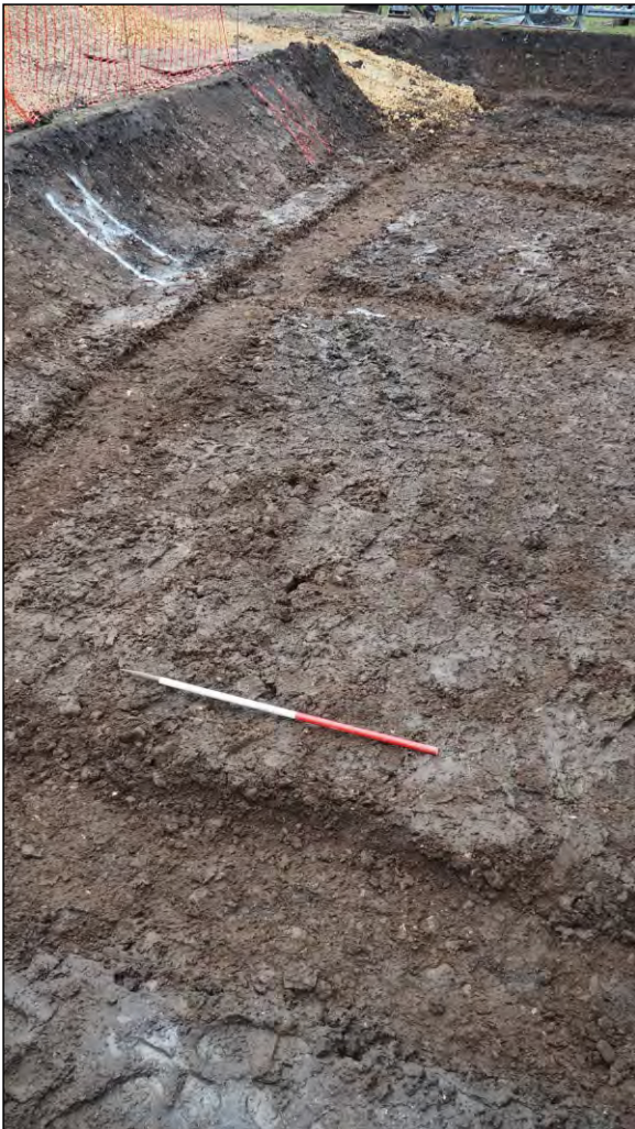
Photo 49. Completed trenching, with detail of graded ramp, for the foundation pad of the new extension. View looking ENE.
