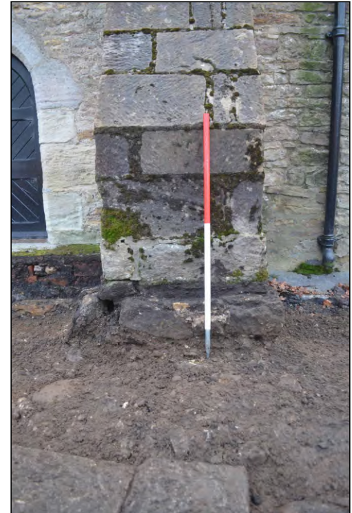
Photo 40. Exposed foundation of western buttress along the north wall of the church. View looking south.
