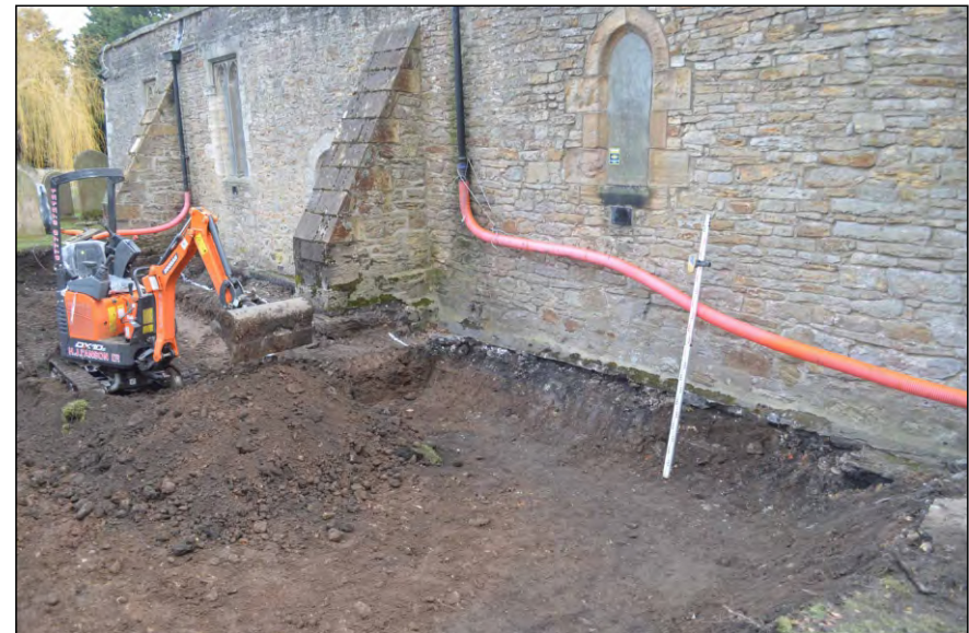
Photo 46. Further ground reduction to the west of the western buttress along the church north wall. View looking south-east.
