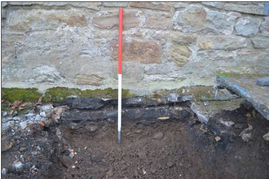
Photo 41. Depth of Church north wall foundations revealed during excavations at the west end of the extension area.
