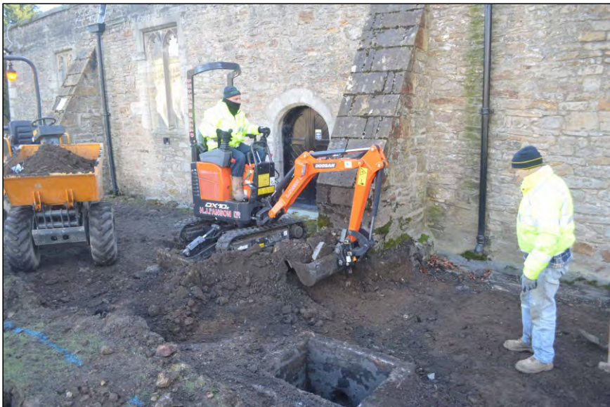
Photo 33. Clearing turf from the extension area revealed a brick soak-away drainage tank [03]. View looking south-east.
