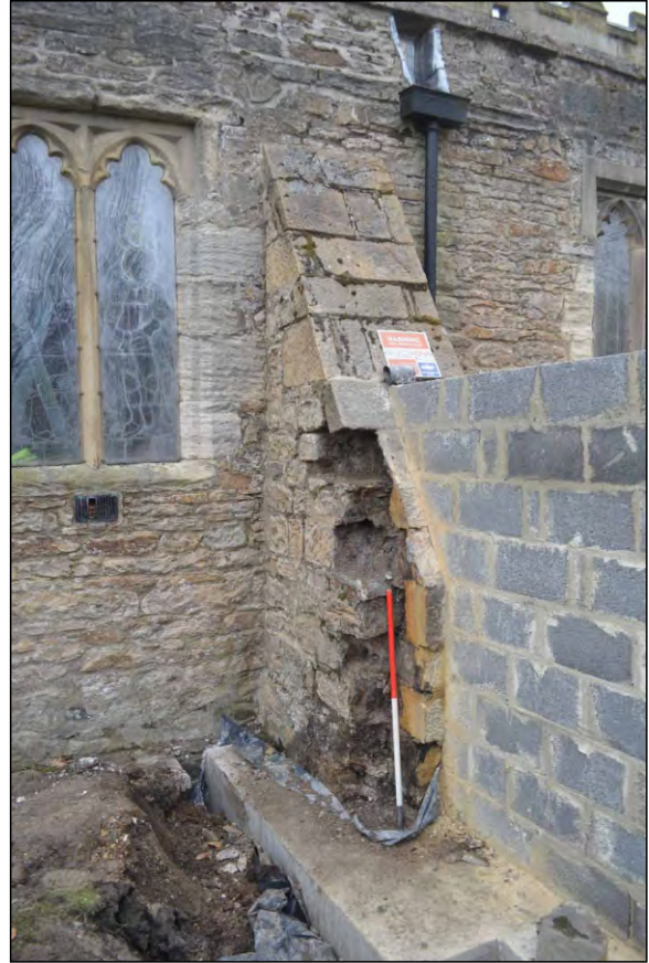
Photo 83. The eastern buttress after removal of facing stones on east side of front elevation.
