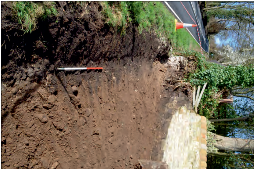
Photo 3. View looking west after demolition and removal of southern boundary wall and shallow grading of the surface for new driveway in.
