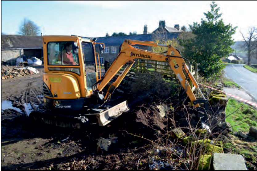
Photo 1. View looking east during demolition of the southern boundary wall, fronting on to the Military Road verge.
