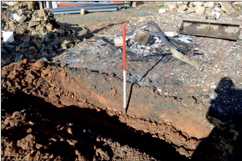
Photo 15. South-southeast facing section of portion of property boundary fenceline trench and driveway area.
