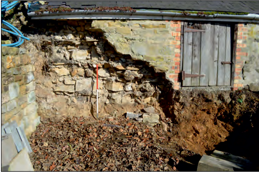
Photo 17. SSW facing elevation of damaged walling at west end of barn, to be demolished.
