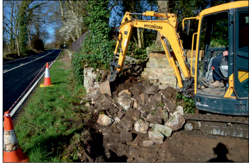
Photo 2. View looking west during demolition of the southern boundary wall, fronting on to the Military Road verge.
