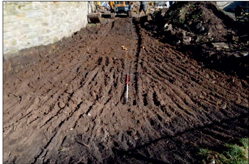
Photo 4. View looking north after demolition and removal of southern boundary wall and shallow grading of the surface for new driveway in.
