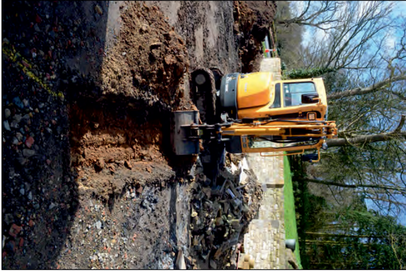
Photo 13. View looking west-southwest during excavation of portion of property boundary fenceline trench and driveway area.
