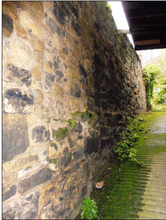
Photo 10: View of the eastern section of the burgage plot boundary wall, looking W up the slope.
