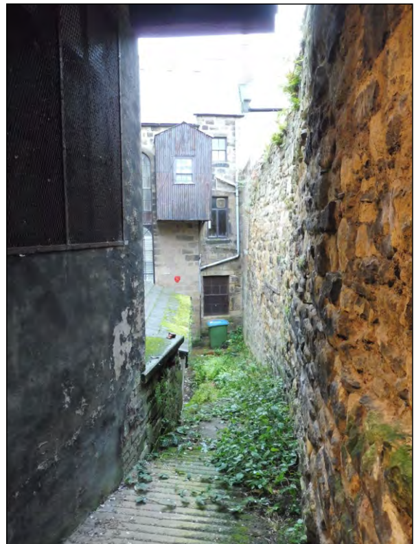
Photo 8: View of the rear yard looking E towards the front building from the narrow passage on the S side of rear wing building 3.
