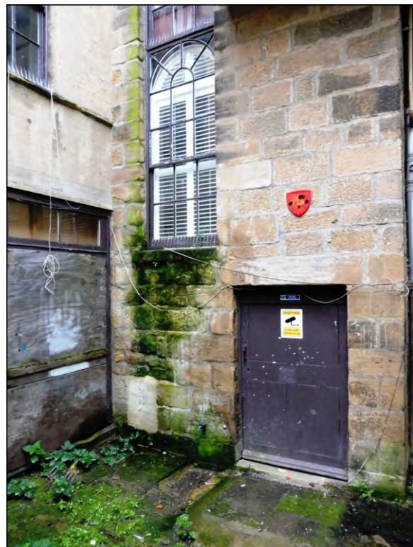
Photo 4: View of the NE corner of the rear yard showing the junction of the S wall of link building 1 and the W wall of the front building.
