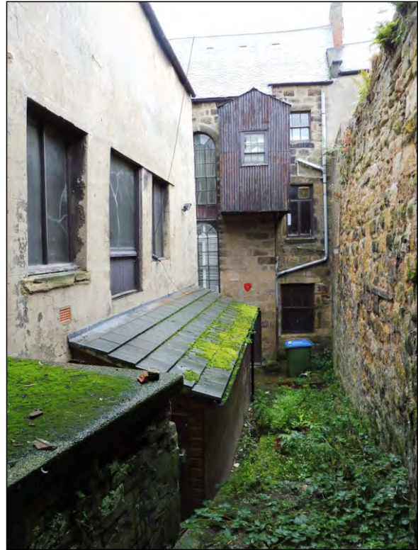
Photo 6: View of the rear yard looking E towards the front building from the S side of rear wing building 2.
