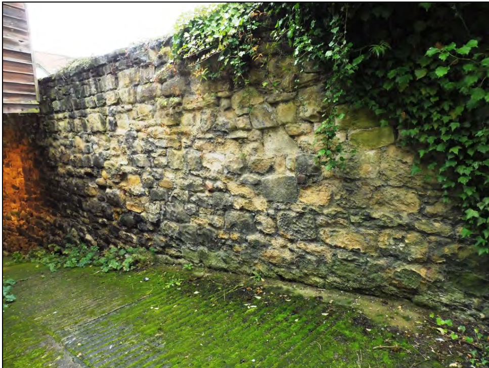
Frontispiece: Part of the boundary wall along the south side of the development site, delimiting the ancient burgage plot
