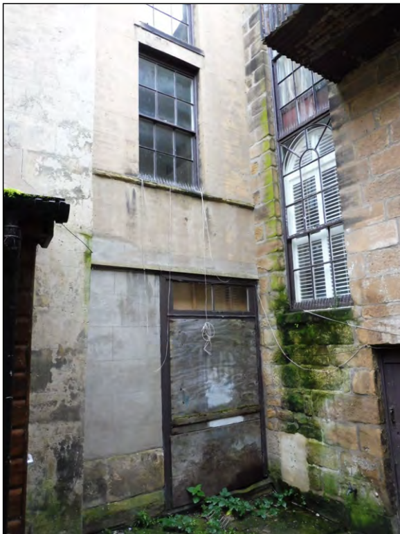
Photo 3: Lower view of the NE corner of the rear yard showing the S wall of the link building (rear wing 1).
