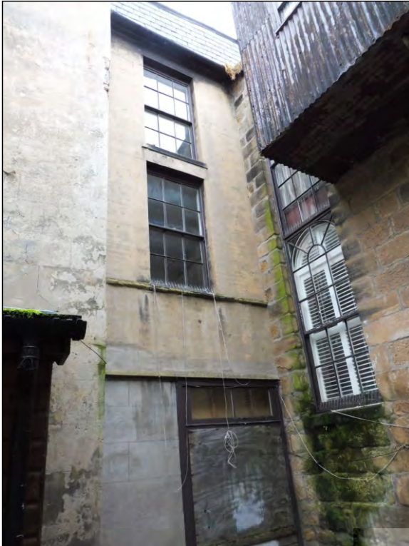
Photo 1: View of the NE corner of the rear yard showing the S wall of the link building (rear wing part 1).
