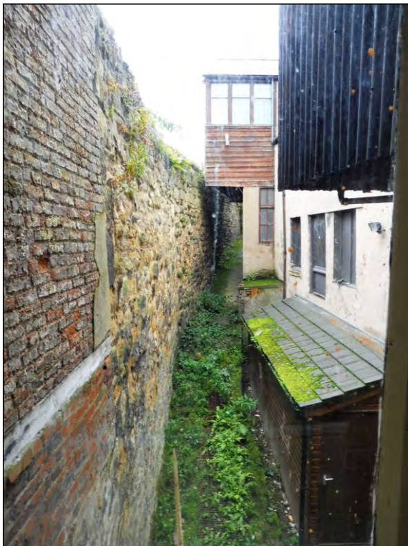
Photo 7: View of the rear yard looking W from the first floor of the front building.
