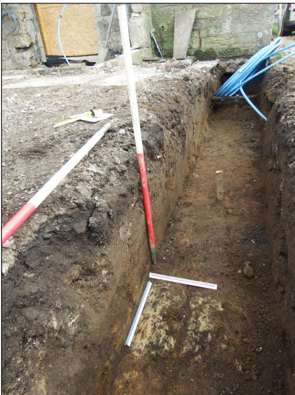
Photo 7: View looking east along south foundation trench with clay patch [06] visible in the foreground.
