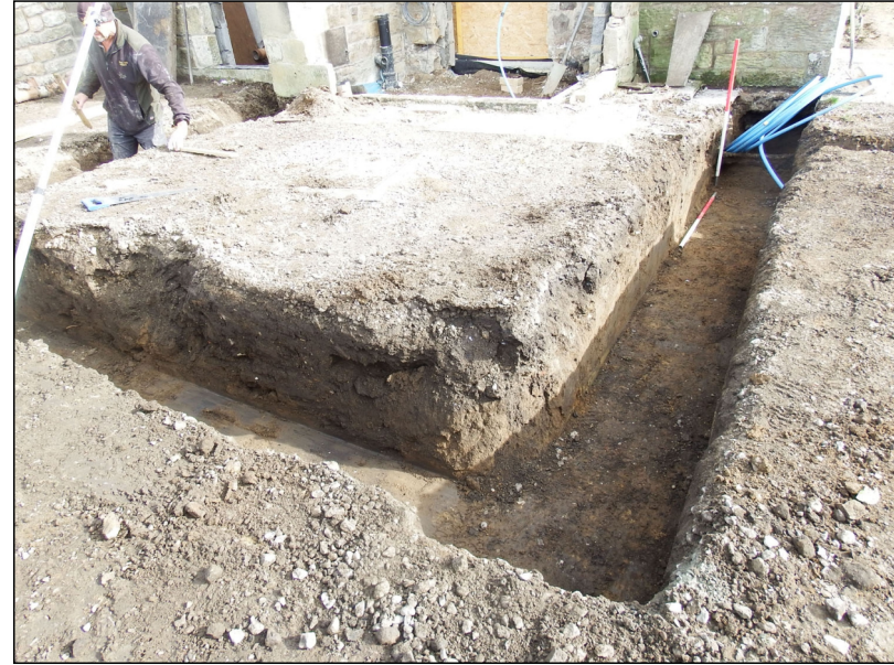
Photo 2: View looking east at foundation trenches abutting the west end of Townhead.
