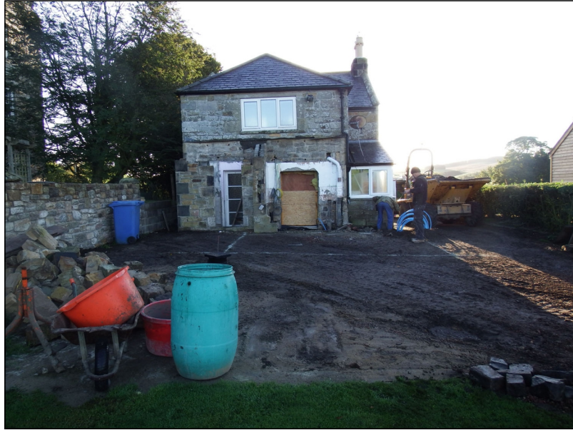
Photo 1: View looking ESE across the watching brief site prior to the excavation of foundation trenches.
