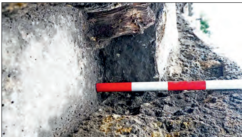
Photo 51. Area C2 view looking SSW at detail of timber post and masonry [13].
