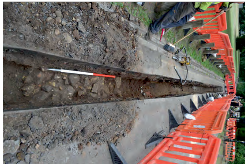
Photo 14. Area B2, broad view looking WNW at detail of sandstone rubble surface [08].
