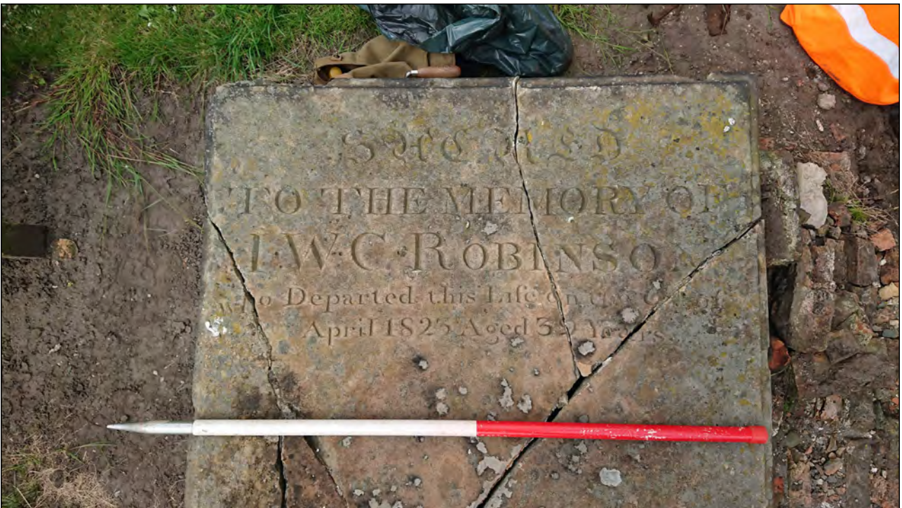
Photo 10. Dedicatory inscription on Tomb Chest 'A', with recently vandalised brick vault beneath.
