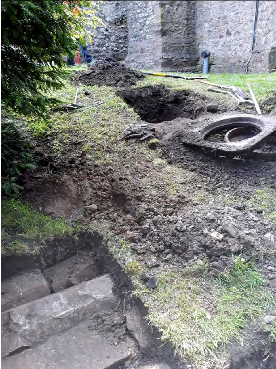
Photo 18. Broad view looking approximately east at second (successful) excavation attempt to find MH1.
