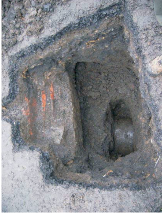
Illus. 31: Test pit within the area of the proposed new development, showing water pipe at c.2m depth.
