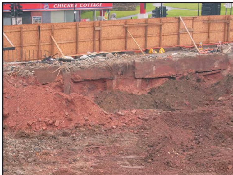
Illus. 10: The foundations of Gallowgate street frontage and the red shale levelling dump, looking south-west.
