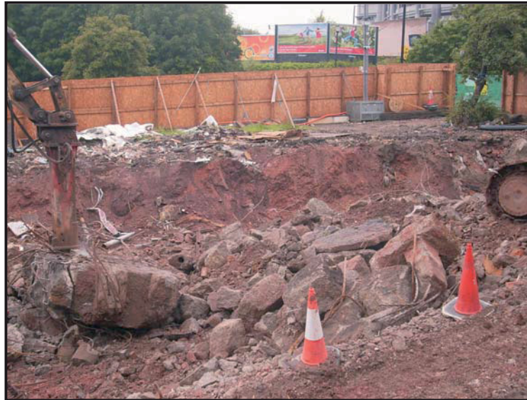
Illus. 09: The removal of rubble after the demolition of Wellbar House, looking north-west.
