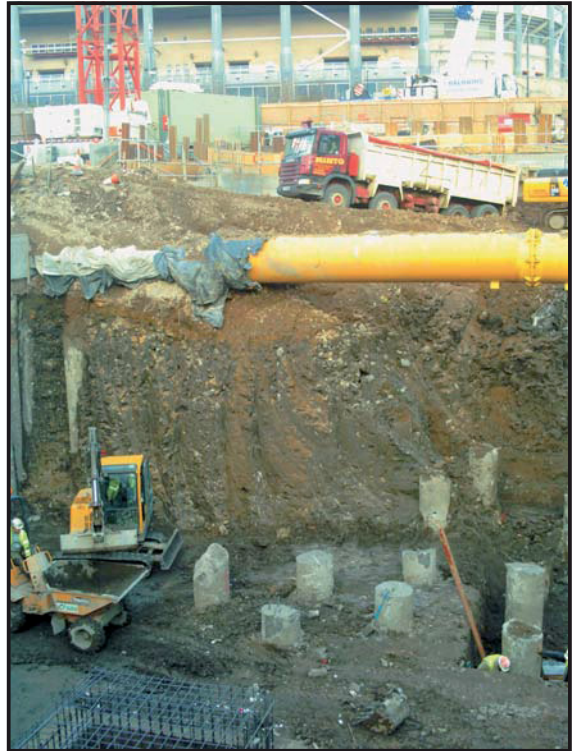
Illus. 16: The development site facing north showing the 1960s pile foundations of Wellbar House in-situ.
