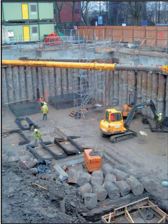
Illus. 15: A view of the development site showing the removed 1960s pile foundations in the foreground with the foundations for the new build in the background, facing south-east.
