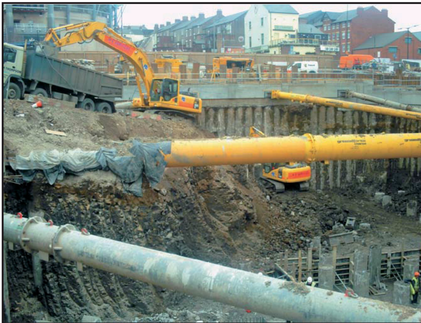
Illus. 20: The removal of the clay in the north-eastern area of the site, taken from the south-west.
