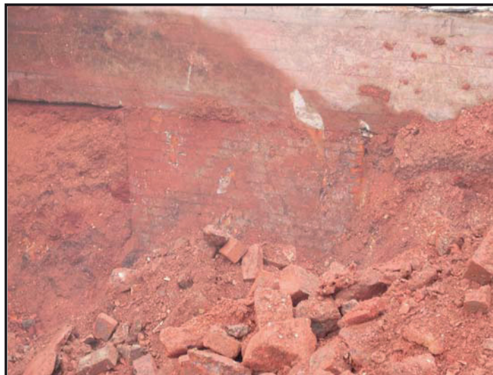
Illus. 13: Brick and concrete wall exposed at the southern end of the development site, forming part of the substructure of the Gallowgate street frontage.
