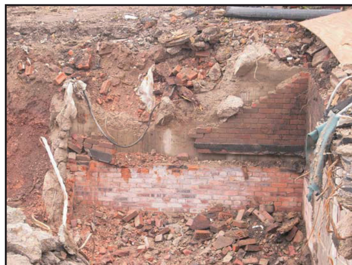
Illus. 14: A brick clad concrete, wall forming part of the substructure of Wellbar House along the eastern side of the development site.
