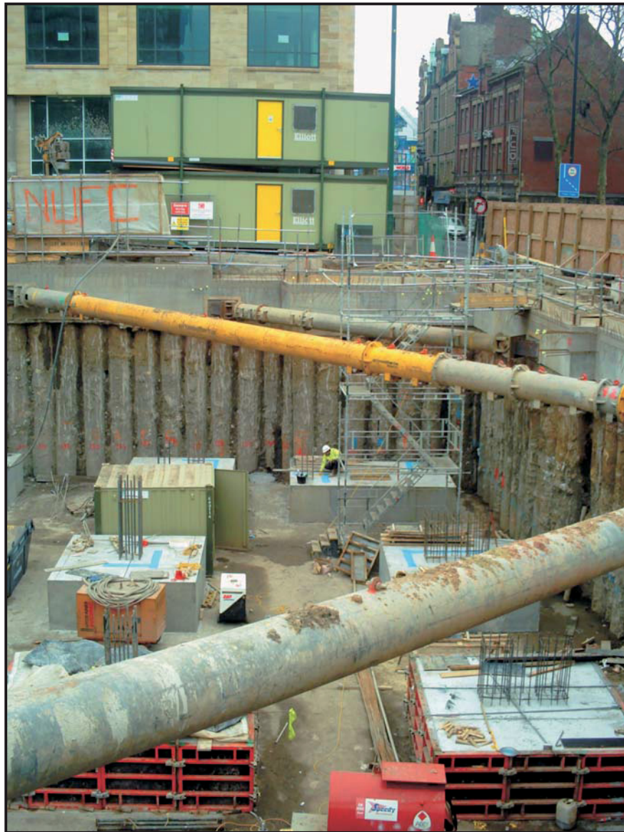
Illus. 21: A general view of the development site facing south-east showing the level down to which deposits have been excavated with the modern foundations in place.
