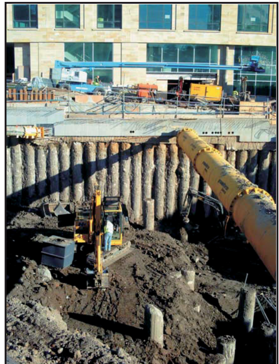
Illus. 18: The removal of the clay surrounding the 1960s pile foundations, facing east.
