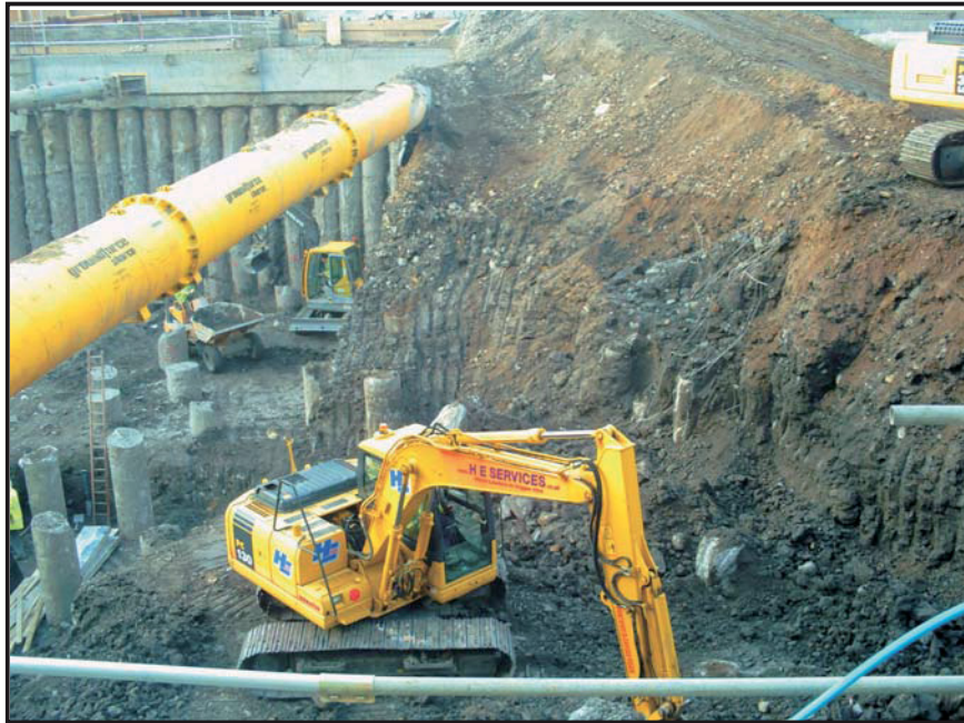
Illus. 19: The removal of the clay in the western area of the site, with the Wellbar House piles exposed in the background, taken from the east.
