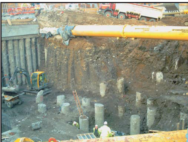
Illus. 17: The development site looking north-west during removal of clay to exposing the 1960s pile foundations of Wellbar House in-situ.
