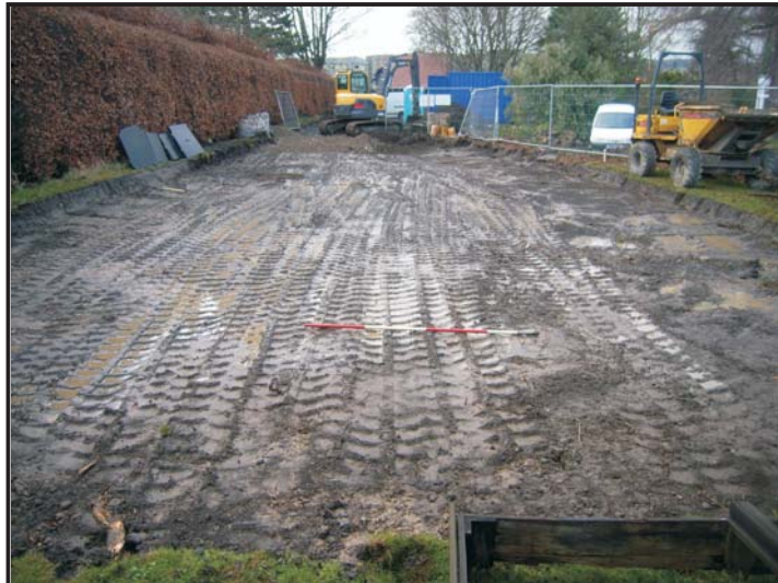
Illus. 14: View from the north of the Ingleboro site during the second phase of construction work, January 31st 2008.
