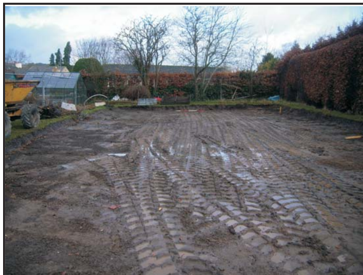
Illus. 15: View of Ingleboro site from the south during the second phase of construction work, February 4th 2008.
