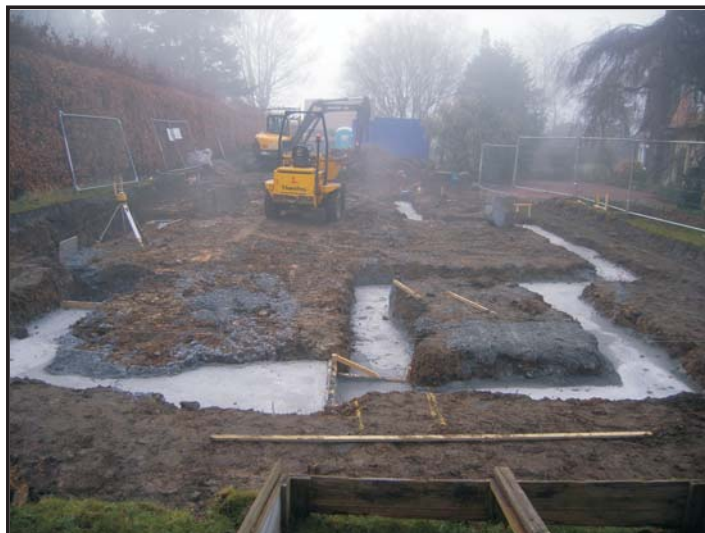
Illus. 21: View of Ingleboro site from the north during the second phase of construction work, February 6th 2008.
