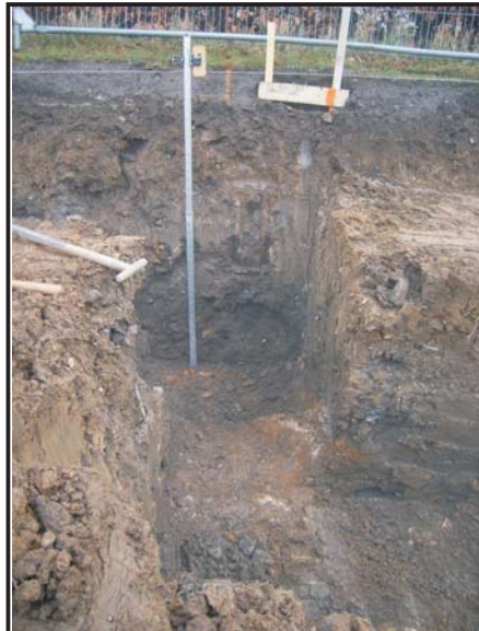
Illus. 20: View from the west of the Ingleboro site during the excavation of foundations on February 6th, 2008.
