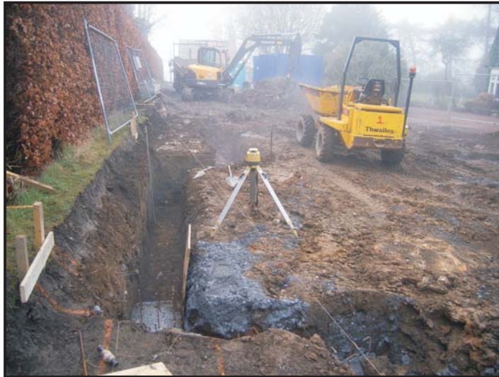
Illus. 19: View from the north of the Ingleboro site during the excavation of foundations on February 6th, 2008.
