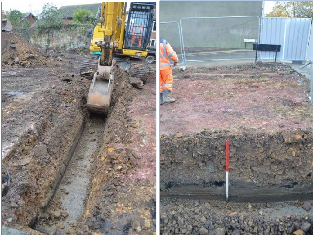
(above left) Photo. 01: The excavation of Trench 4 in Phase 1 of the watching brief)
