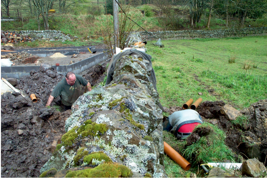
Plate 3: Excavating an ancillary service trench through the southern boundary of the site
