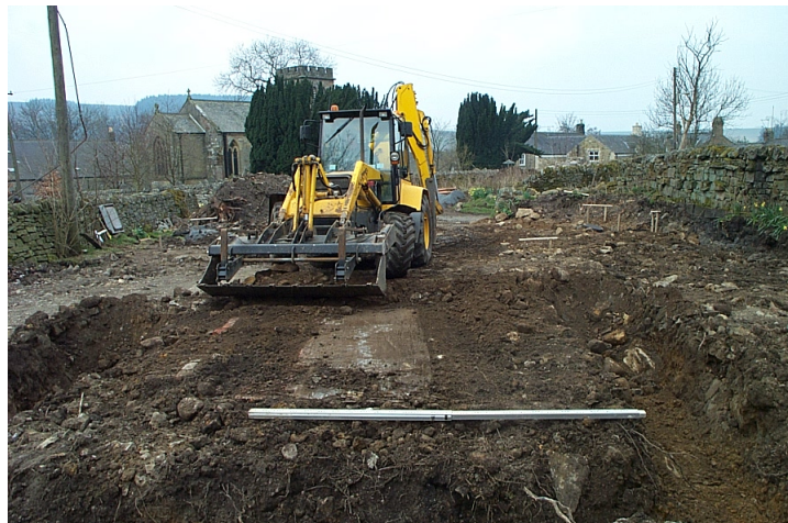
Frontispiece: The Old Garage site, Falstone – view from the east during machine excavation of foundation trenches
