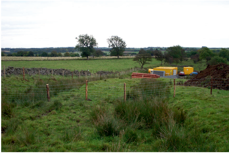
Plate 9: Holloways running S-E into works compound area, with soil dump to right
