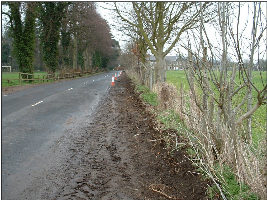
Plate 2: General view of the strip of land excavated to make way for the new footpath (facing east towards Corbridge)
