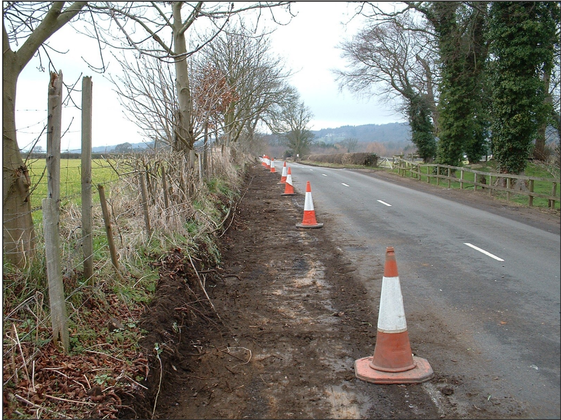
Plate 1: General view of the strip of land excavated to make way for the new footpath (facing west towards the English Heritage Visitors Centre)
