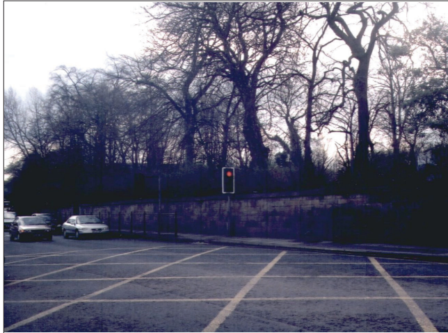
Illustration 21: View of the retaining wall along the west side of North Road
