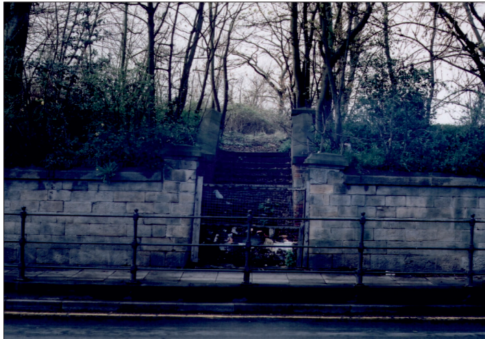
Illustration 22: View of the steps in the retaining wall showing difference between the original and later levels of North Road
