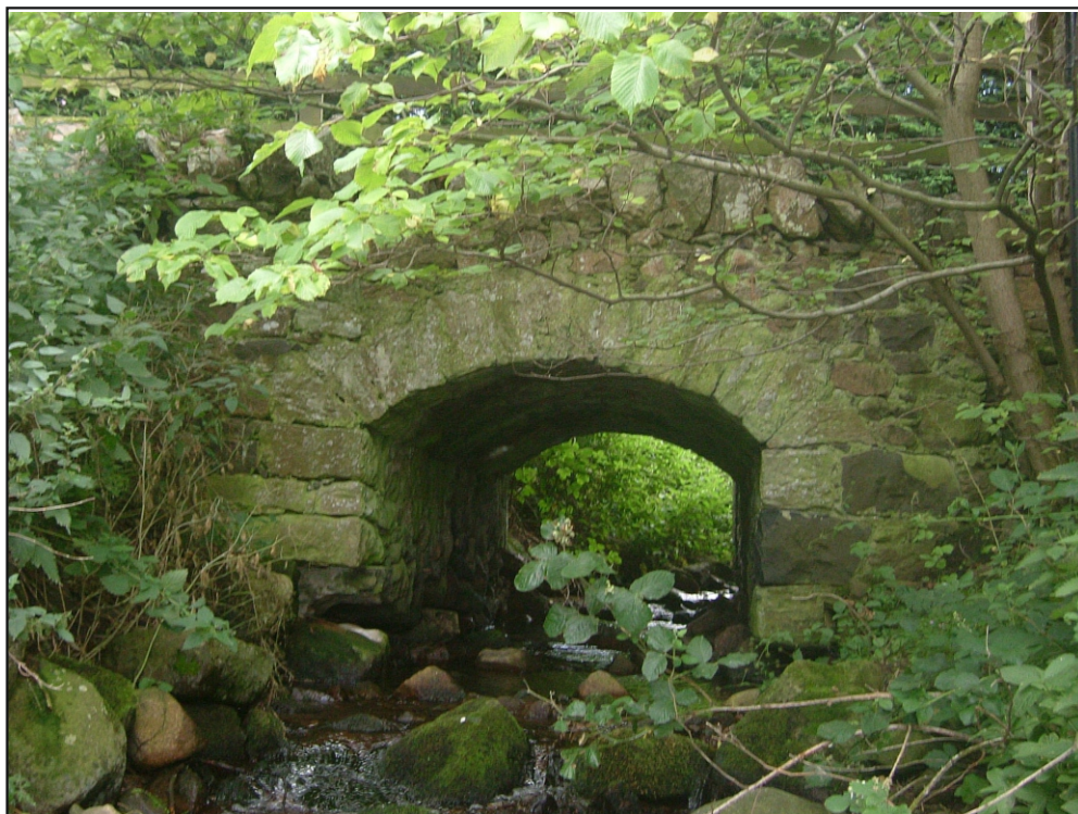
Fig. 43: Bridge over the Akeld Burn, next to site of Akeld mill (AK_MP 074)
