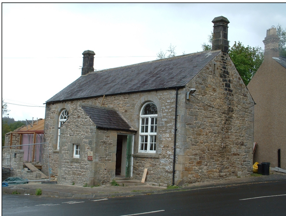
Fig. 55: Falstone schoolhouse during restoration and conversion to a Northumberland National Parks Authority café and visitors centre, Summer 2004(Fal_MP 021)
