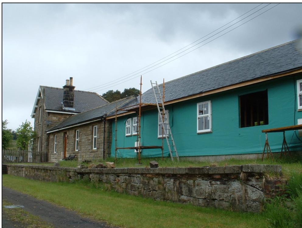
Fig. 61: Falstone Station (Fal_MP 063)
