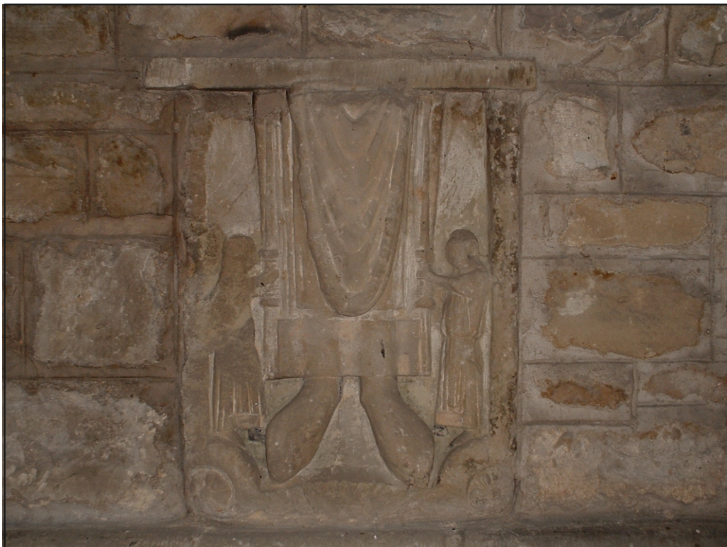
Fig. 48: Lower part of a medieval tomb effigy, probably of a churchman, re-used in the north wall of St Michael's Church, Ingram (Igm_MP 004)
