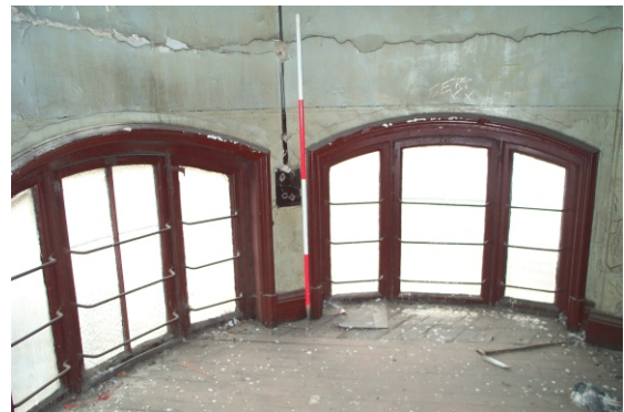
Illus. 25: Third floor NW corner (windows look out over the High Level Bridge towards Newcastle Castle Keep).
