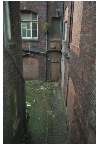
Illus. 29: View from north-east stair well towards lower part of the south wing, north elevation facing courtyard
