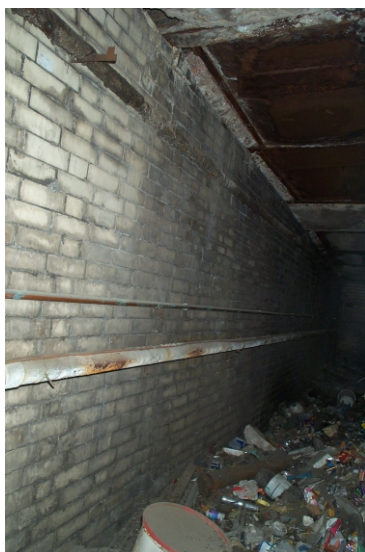
Illus. 18: Sunken area between front of basement and road (footpath above)
