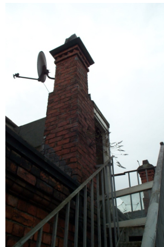
Illus. 31: Chimney stack on roof of the south wing, viewed from fire escape
