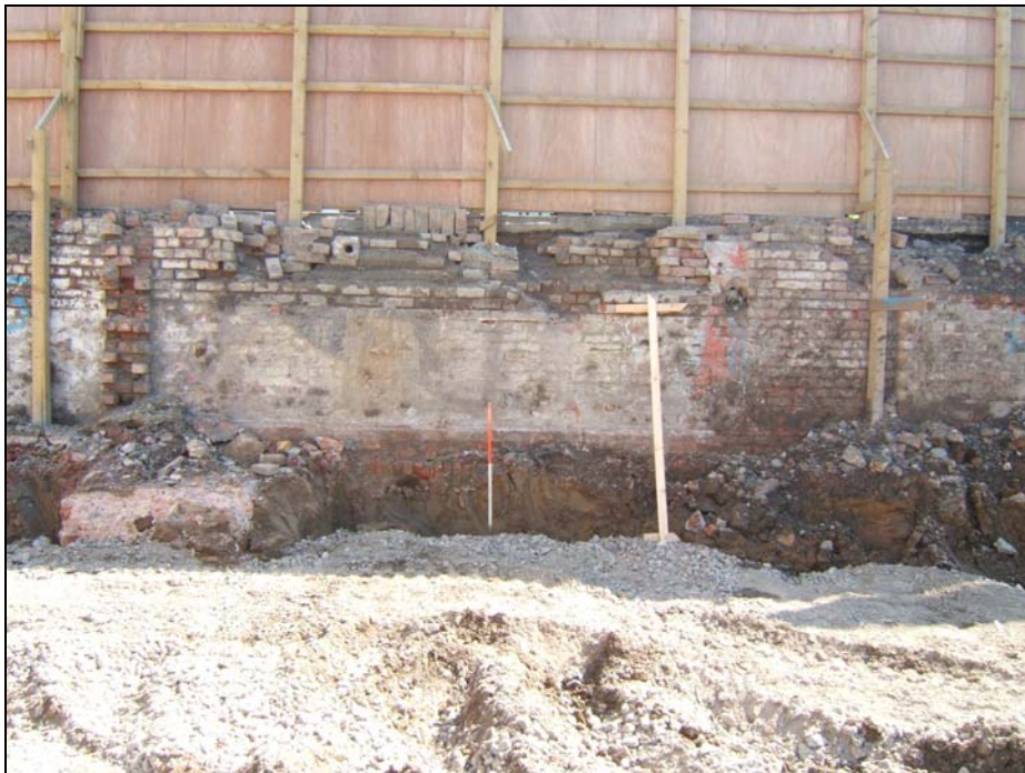
Frontispiece: Front wall of the cellaring for 30-34 Gallowgate and underlying clay deposits
