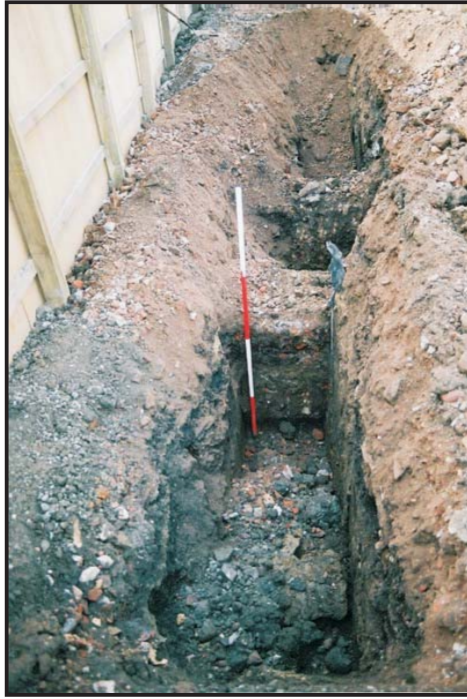
7. Piling trench along the S edge of the development site showing brick walls probably associated with Corporation Baths (looking W)
