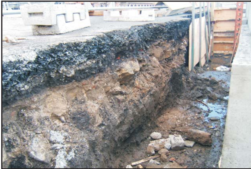
1. The trench for the revetment wall of the access ramp viewed from the west. The section shows layers of demolition rubble and redeposited material
