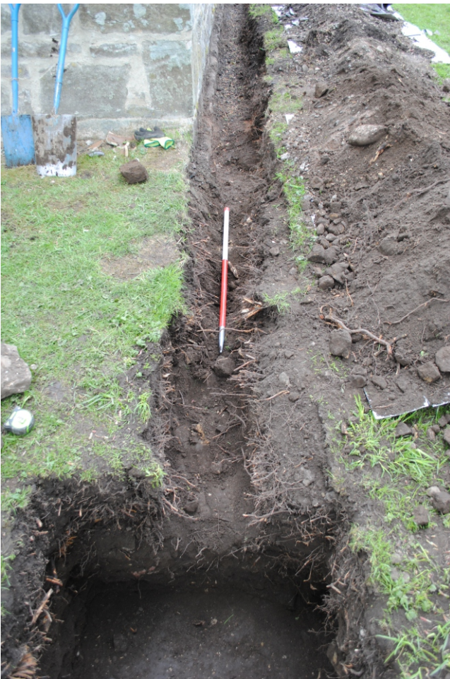
Photo 02. View looking west from soakaway pit 1 towards the excavations for the drain.
