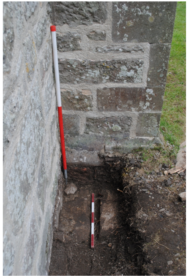
Photo 06. The foundations adjacent to the north buttress on the west wall. South view..
