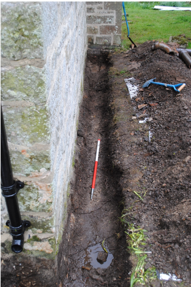
Photo 05. View looking south in the return of the trench for the drain.
