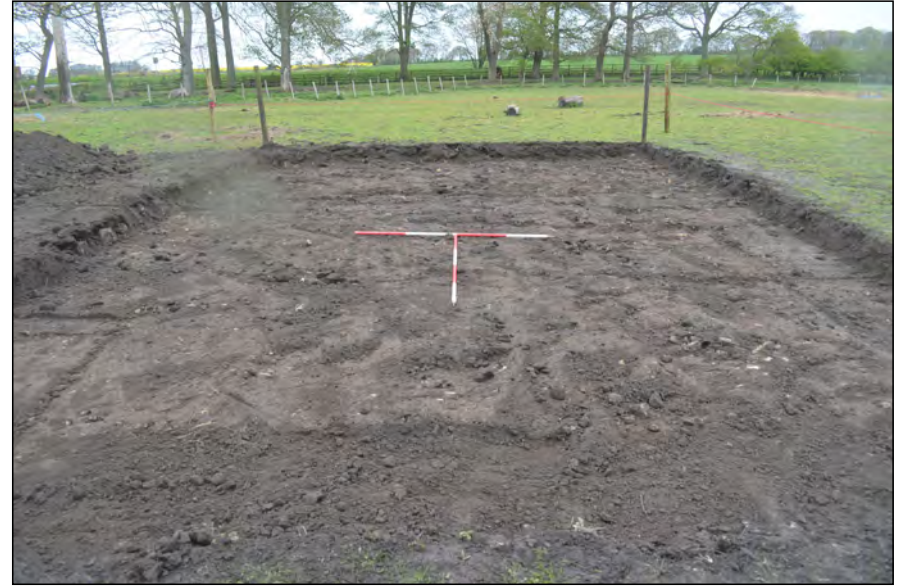
Photo 06. View looking NNE along the finished excavation area subject to watching brief (scales visible = 2 x 2m).
