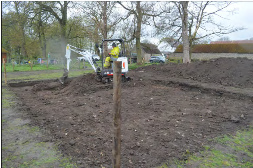
Photo 03. View looking south-west after further excavation progress across the watching brief site.
