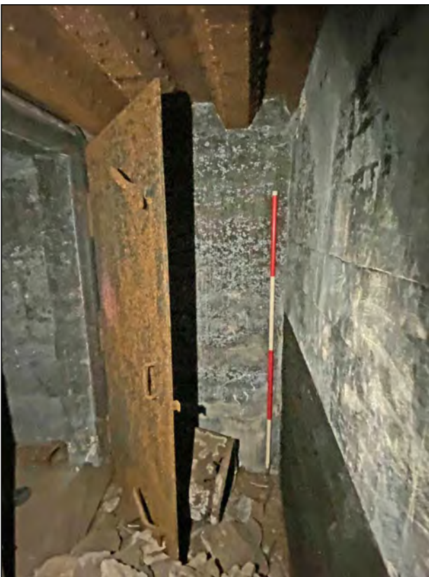
Photo 35. View looking NE at doorway opposite the spiral stairway in short exit corridor return.
