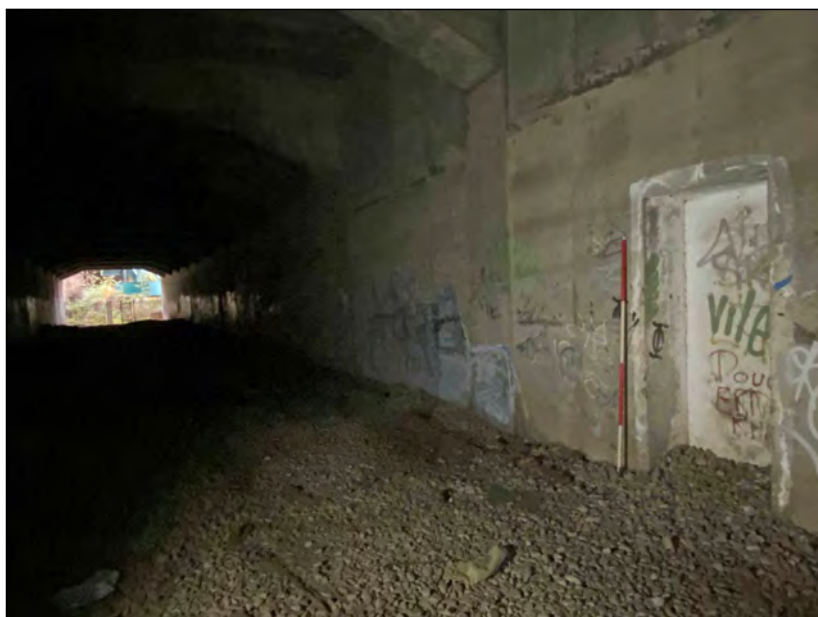
Photo 15. View looking north-west along the tunnel, with Retreat Alcove 05 in the foreground.
