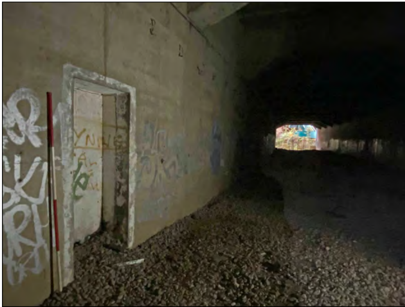
Photo 17. View looking south-west along the tunnel, with Retreat Alcove 06 visible in the foreground.
