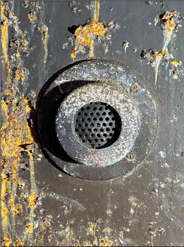
Photo 10. View of air vent grill.
