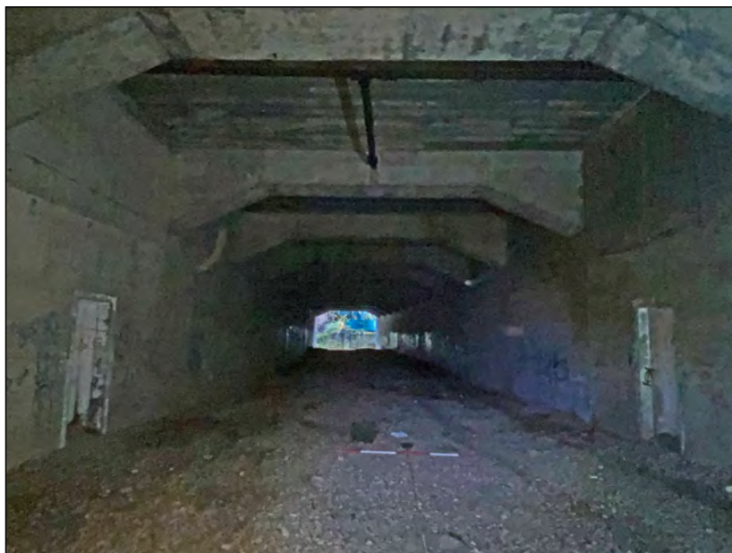
Photo 14. View looking west along the tunnel, with Retreat Alcoves 05-06 visible in the foreground.
