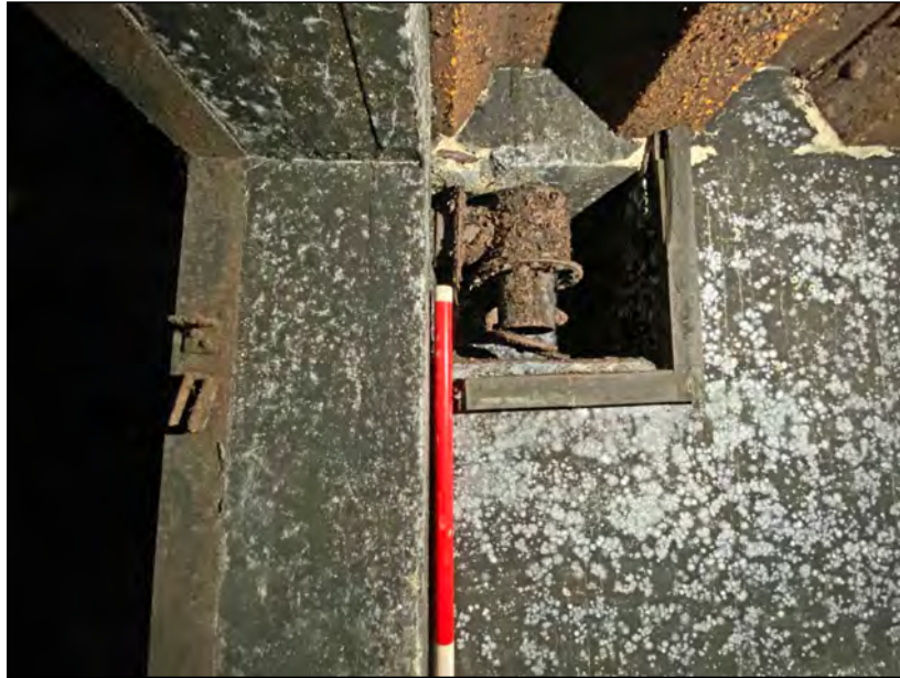
Photo 34. View of service vent at SE end of exit corridor.
