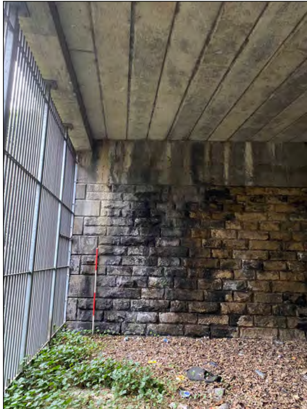
Photo 01. View of the east end of / entrance to the railway tunnel, looking south.
