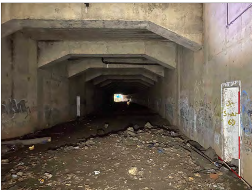
Photo 05. View looking west from near the east end of the tunnel, with Retreat Alcove 01 visible (foreground right).
