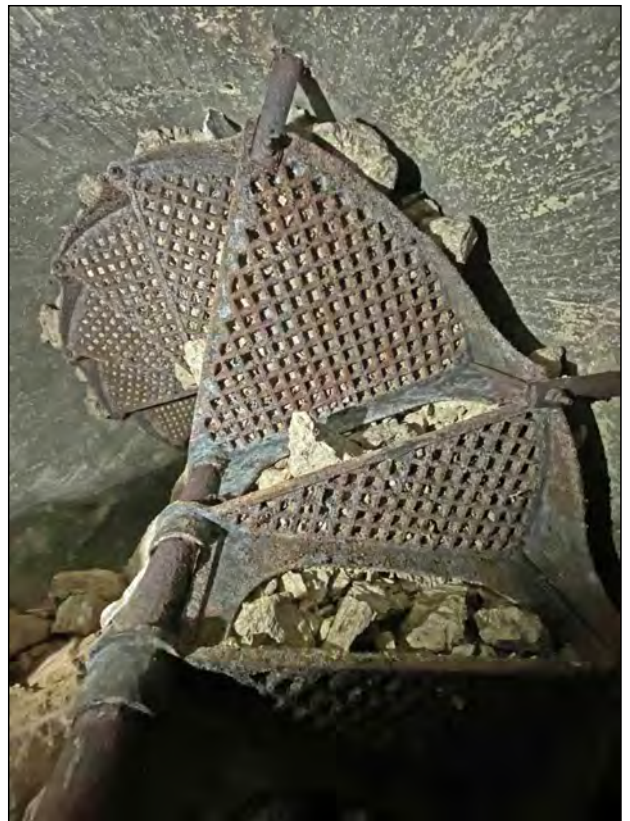
Photo 39. Alternative view looking upwards at blocked spiral stair exit.
