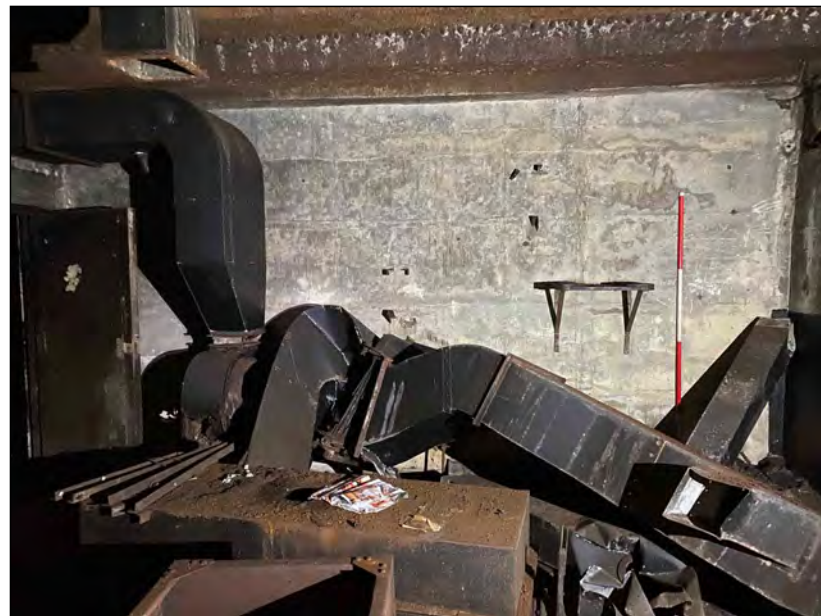
Photo 16. View of collapsed air filtration ducts against the north wall in Room 1.
