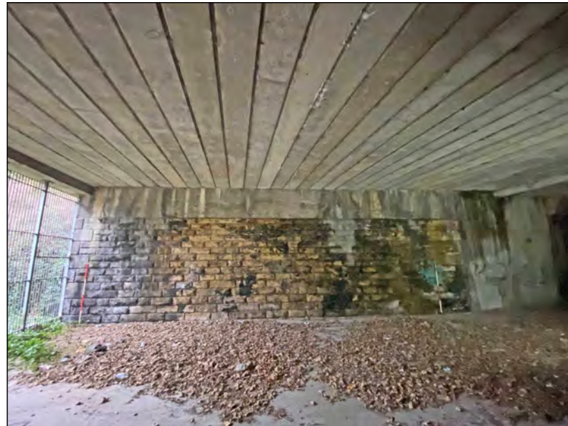
Photo 02. Broad view of the east end of / entrance to the railway tunnel, looking south.
