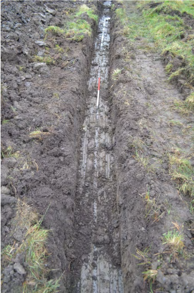
Photo 06. View looking west at the pipe trench to the west of the water treatment tank.
