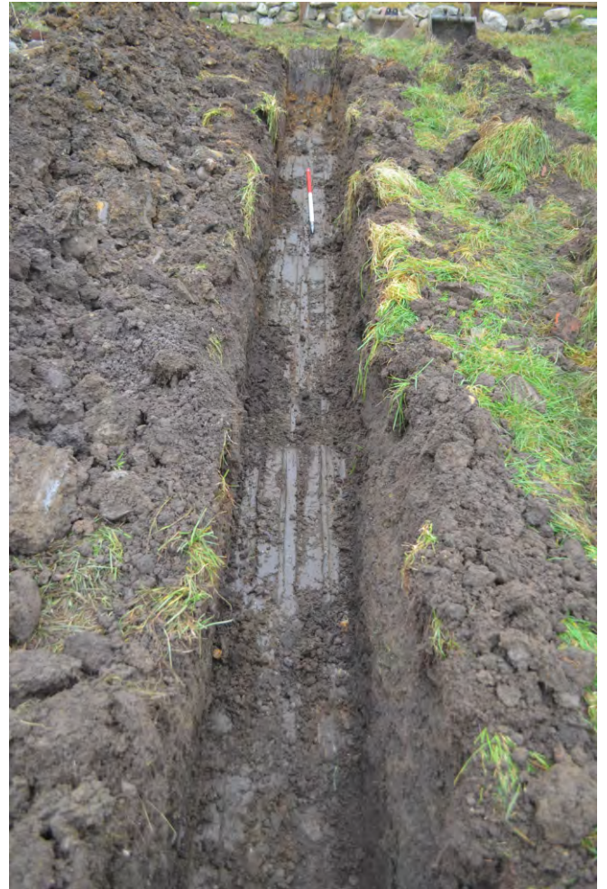
Photo 10. View looking north at the north-south section of trench to the west of the water treatment tank, N of Photo 09.
