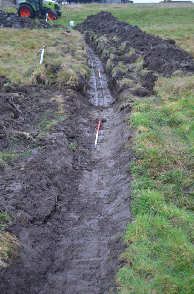
Photo 03. View looking north at the pipe trench to the east of the water treatment tank.
