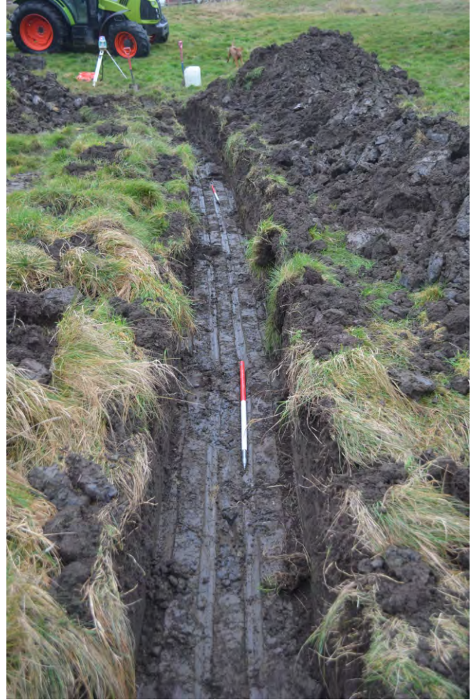
Photo 04. View looking north at the pipe trench to the east of the water treatment tank, N of photo 03.
