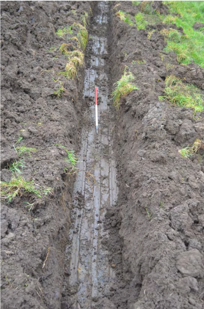
Photo 09. View looking north at the north-south section of trench to the west of the water treatment tank.
