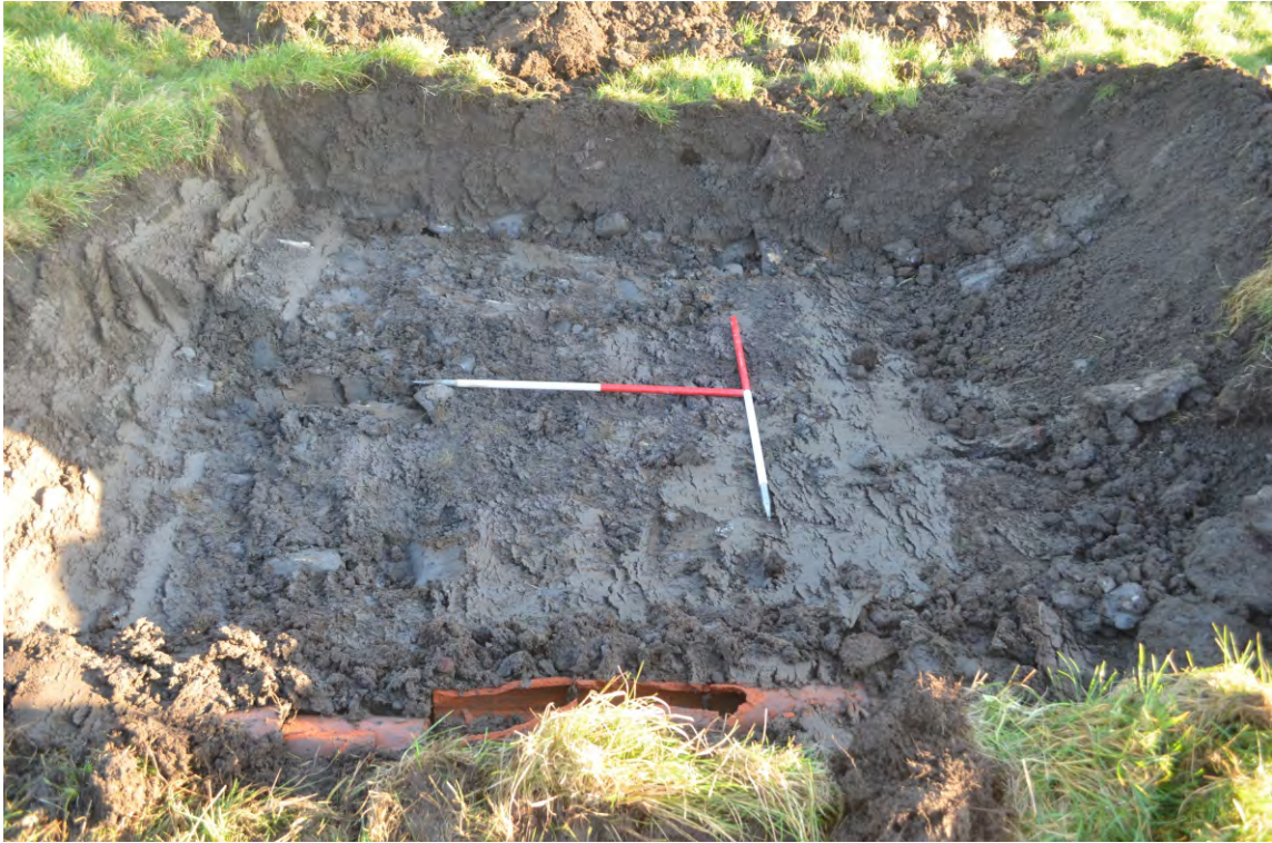
Photo 01. The pit for the water treatment tank, photographed partially excavated at the horizon of the boulder clay.
