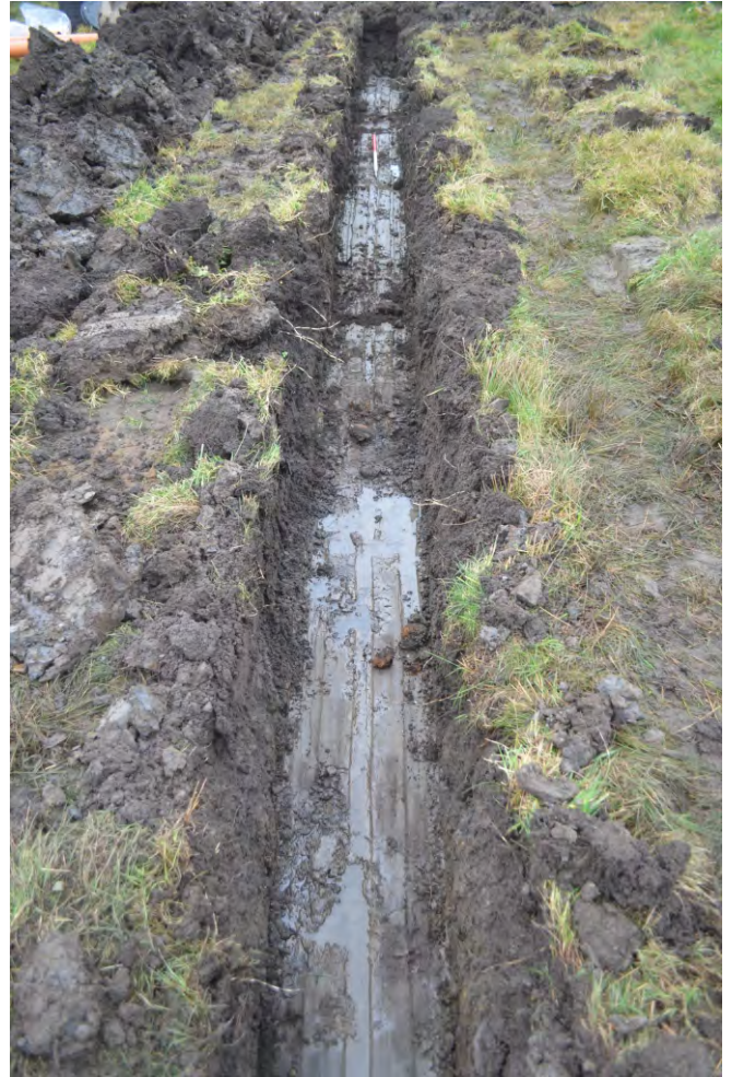
Photo 07. View looking west at the pipe trench to the west of the water treatment tank, W of photo 06.
