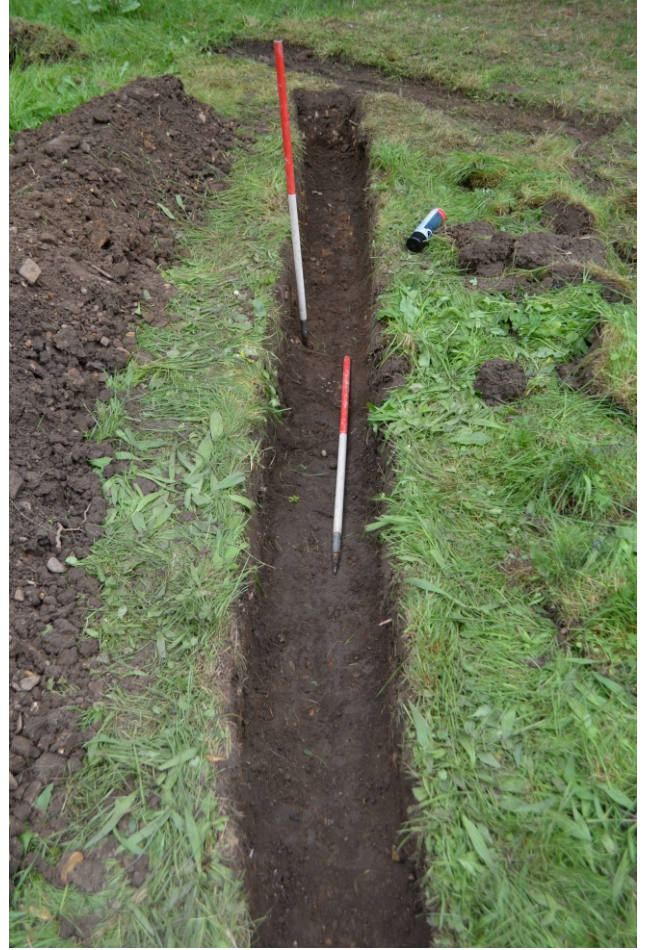
Photo 14. South-east view of pipe trench and the beginnings of the soakaway pit.
