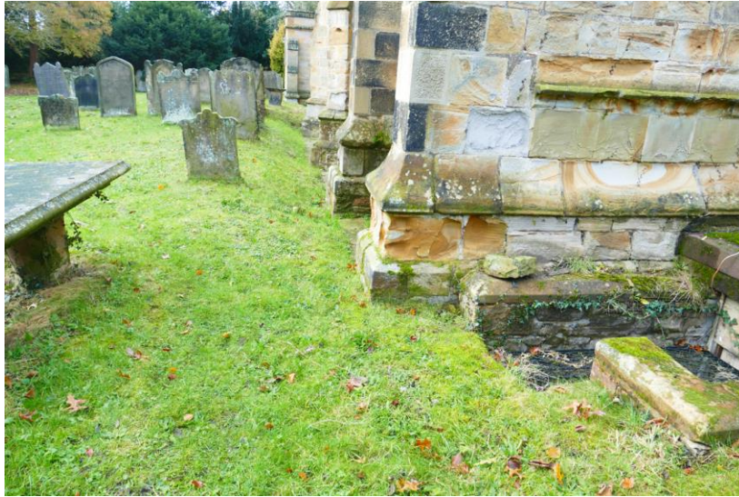
Photo. 01: View from the east of southern buttresses to the nave, showing a rise in ground level onto the cemetery area to the south.
