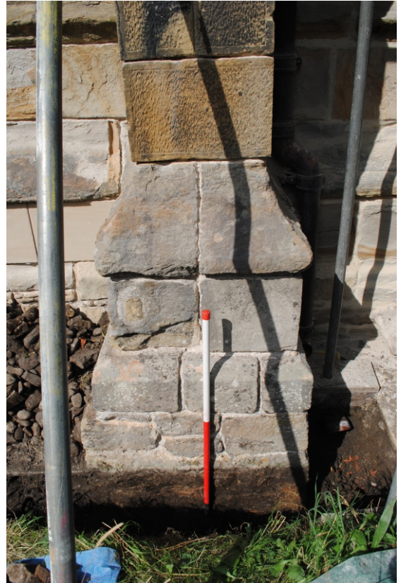
Photo 10. Excavations expose the base of the central buttress of the 'Lady Chapel'. North view.
