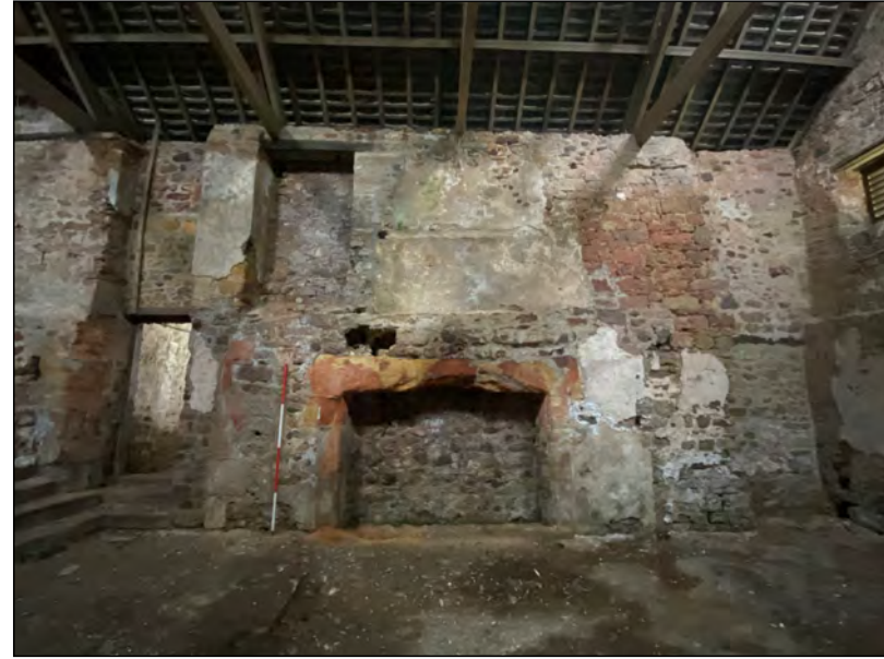
Photo 62. The north part of the internal (E-facing) west wall of the 'Old Hall', with fireplace prominent.
