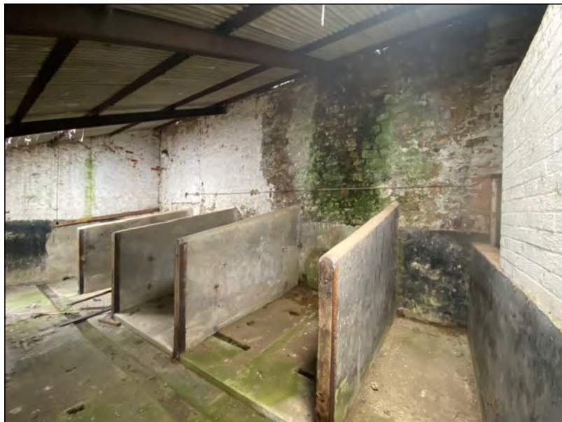
Photo 47. View NE over stalls within the southern lean-to extension of the east range, north part of the west elev of the 'Old Hall' and (left) part of south gable end of original east range.
