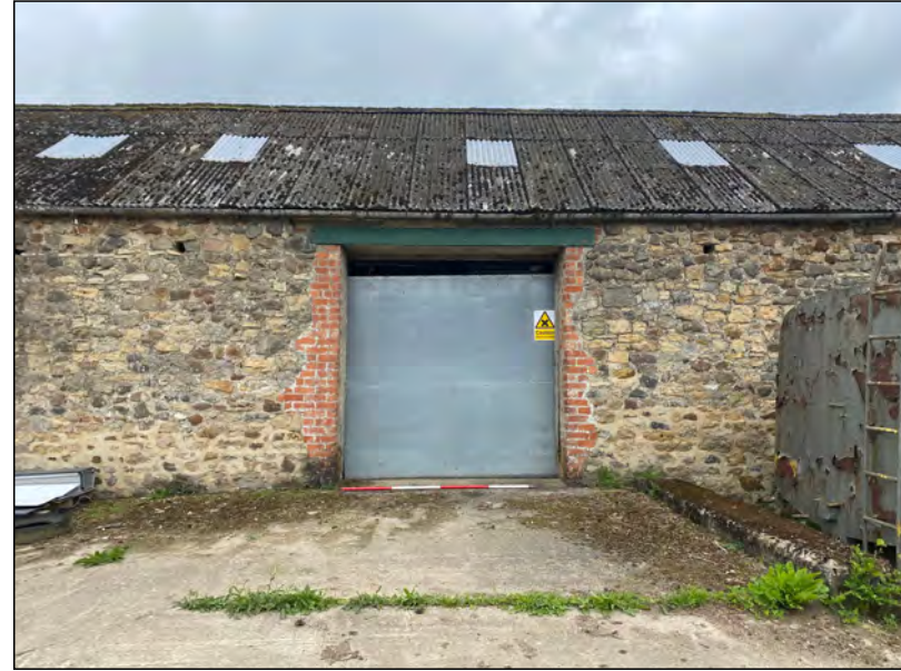
Photo 10. Doorway in the middle part of the north elevation to the north range
