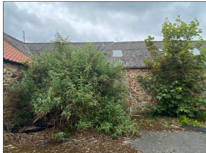
Photo 32. The west part of the south elevation to the north range of farm-buildings (partly obscured by vegetation).
