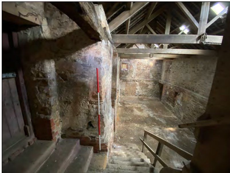
Photo 83. View NNE from the internal south-west corner of the internal first-floor space.
