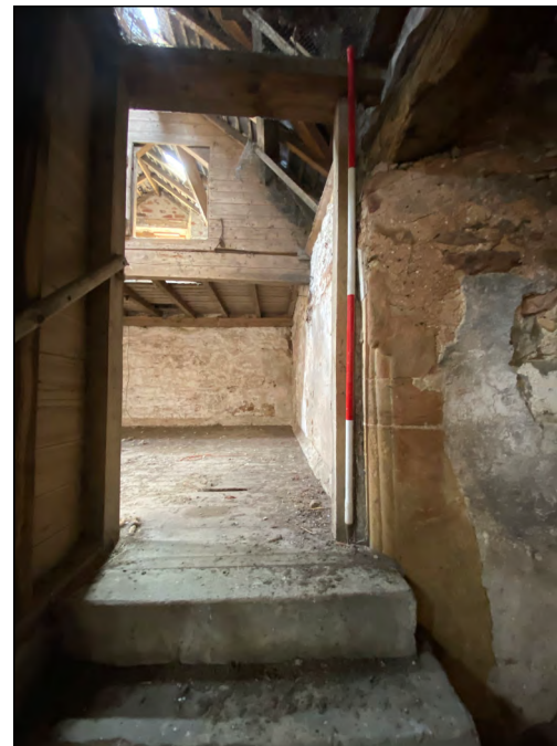
Photo 72. View from the north of top of stairs at first-floor level, showing the surviving, decorated south jamb of former first-floor fireplace.
