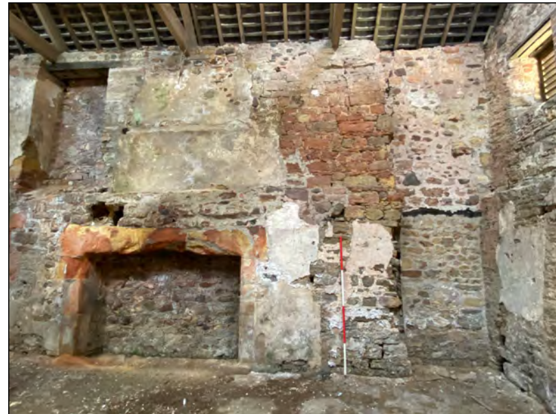
Photo 64. The N end of the internal (E-facing) W wall of the 'Old Hall', with fireplace to left and blocked opening with timber lintel at extreme right.
