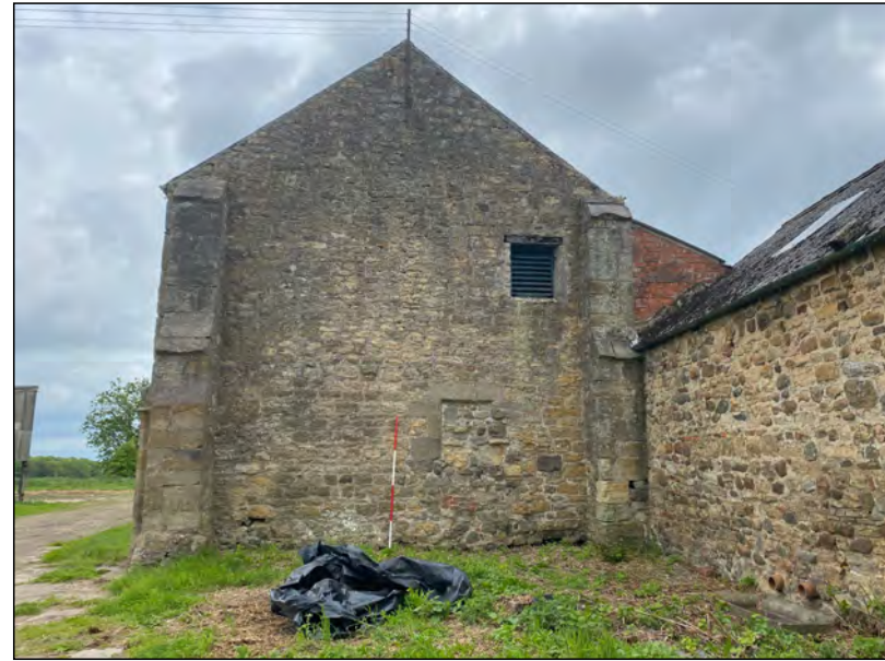
Photo 14. The north elevation of the 'old hall' attached to the east side of the east range.
