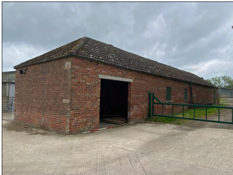
Photo 39. The west and north (left of view) elevations of the detached north-west range seen from the north-west.
