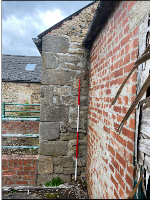
Photo 29. Quoins forming the south-east corner of the original north part of the east range, projecting from a later lean-to addition to the south.
