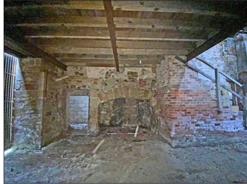
Photo 58. The south part of the internal face of the west wall of the 'Old Hall', with fireplace and modern brick-built stairs to first-floor level.
