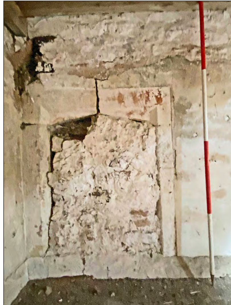
Photo 82. Blocked fireplace in the east-facing internal face of the south end of the west wall at first-floor level.
