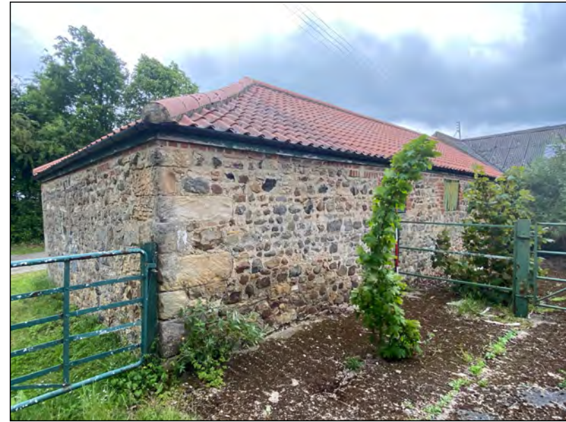
Photo 34. View from the south-east to the west (right of view) and south elevations to the west range of farm-buildings.
