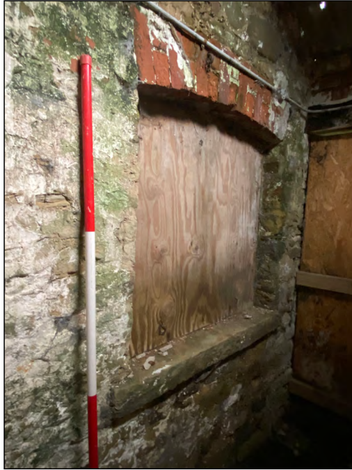
Photo 49. View south-west of window in the north part of the east elevation of the south range of farm-buildings.
