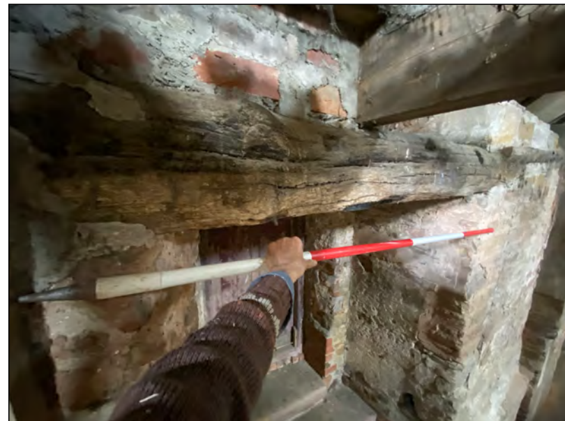
Photo 76. View from SE of worked timber reused as a window lintel in the south part of the west wall at first floor level.
