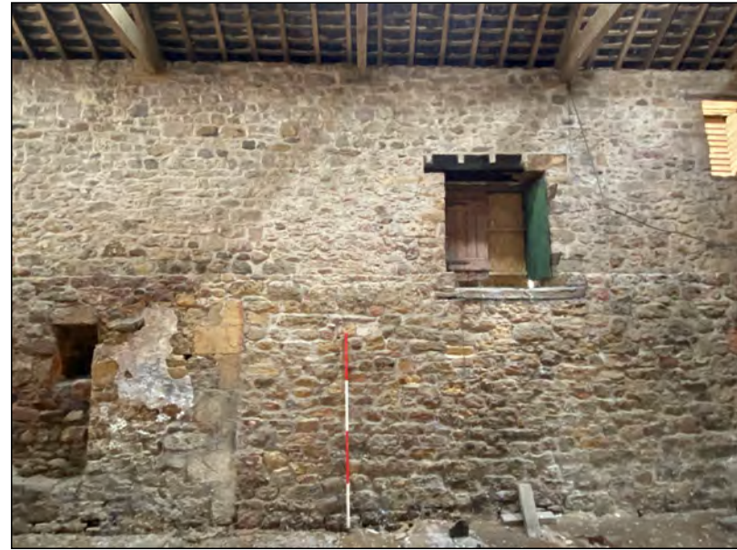
Photo 54. The north-central part of the internal face of the east wall of the 'Old Hall'.
