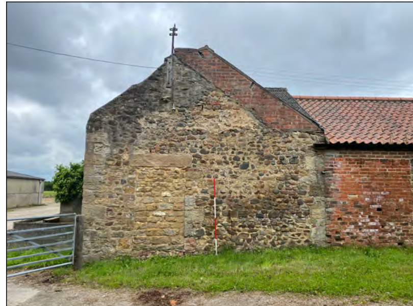
Photo 08. West gable elevation of the single-storey north range of farm-buildings, showing blocked doorway and alterations to the roof structure.
