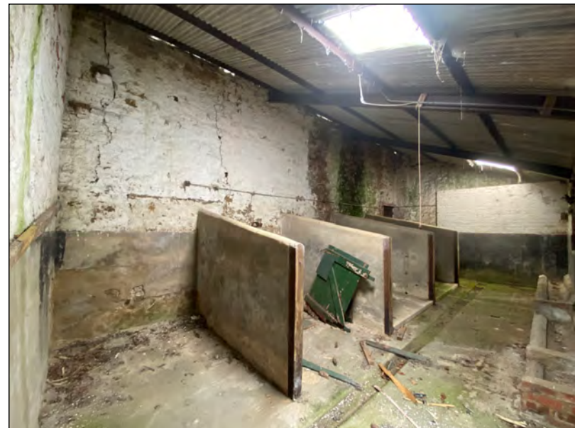
Photo 44. View SE within the southern lean-to extension of the east range over stalls to the north part of the west elevation of the 'Old Hall' and (right of view) the east end of the GF elevation of the south range of farm-buildings.
