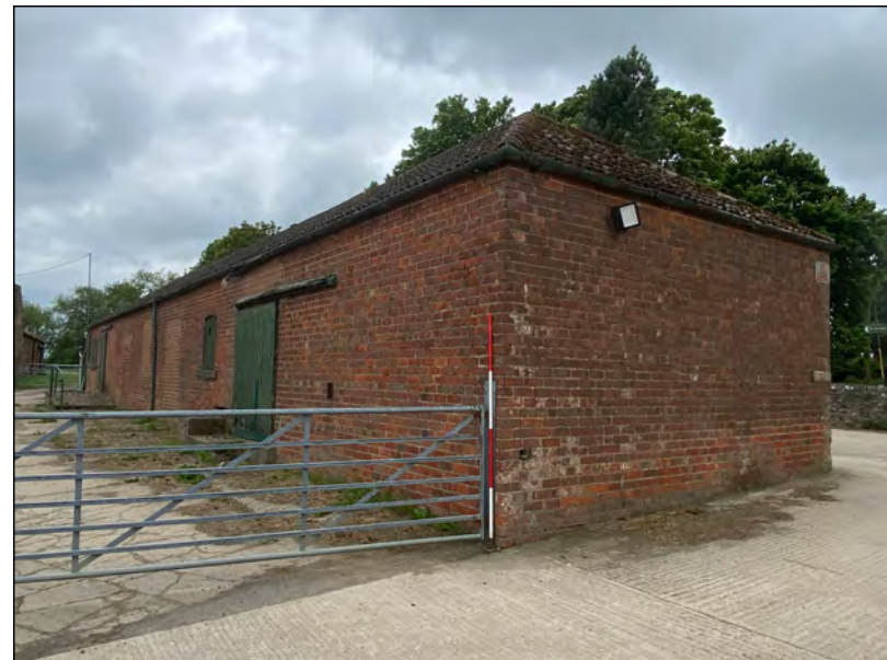
Photo 40. The north (right of view) and east elevations of the detached north-west range seen from the north-east.
