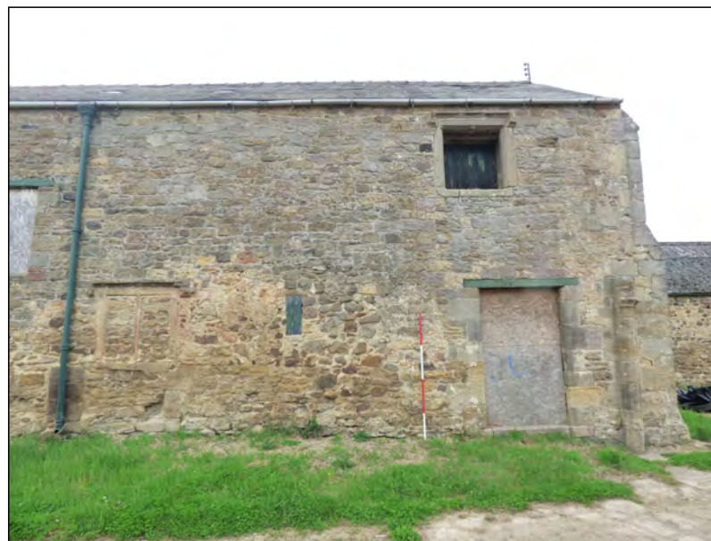
Photo 18. The north part of the east elevation of the 'Old Hall', with remains of the respond of an arch at the north end and blocked ground-floor window set north of centre, with another medieval window suggested at first-floor level by an indistinct patch of rubble (more clearly visible on the internal face).
