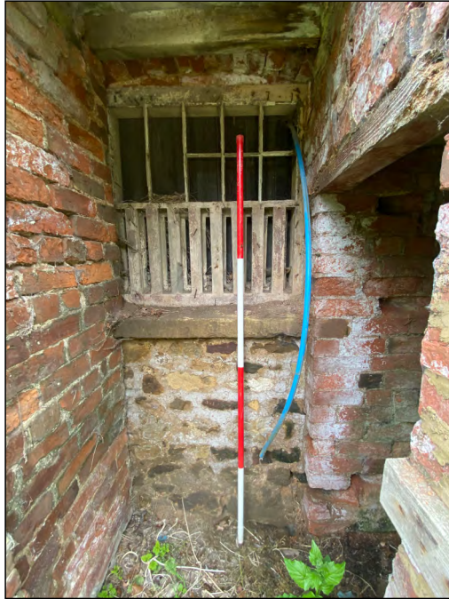
Photo 25. Windowed opening below brick external stair to the first-floor granary at the west end of the south range.
