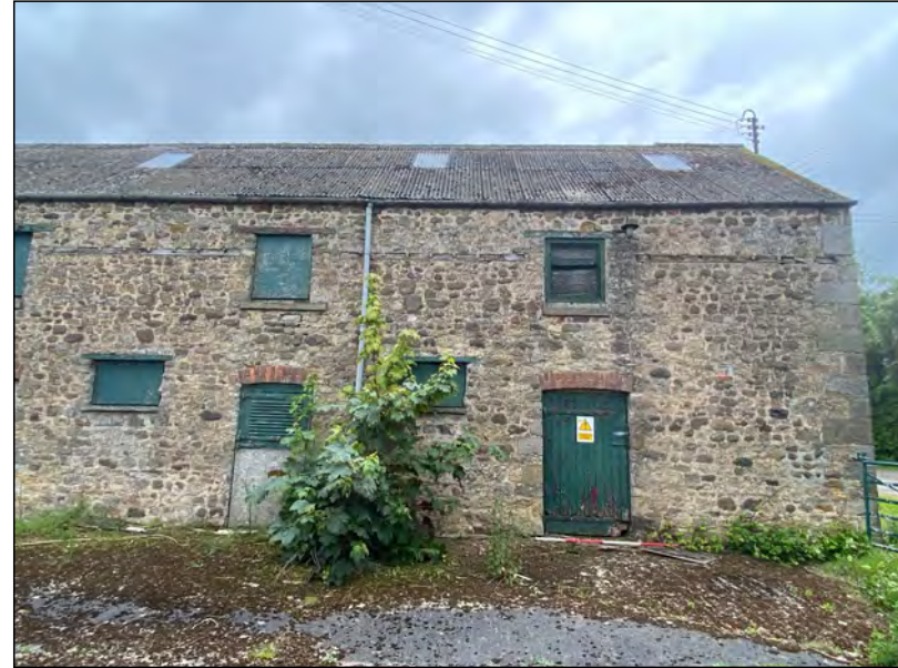
Photo 26. The west part of the north elevation of the south range of farm-buildings.
