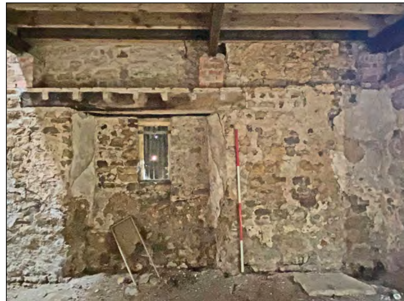
Photo 56. The south part of the internal face of the east wall of the 'Old Hall'.
