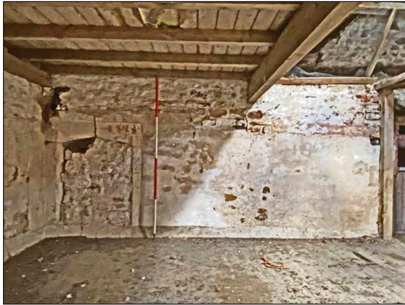
Photo 81. The east-facing internal face of the south end of the west wall at first-floor level.
