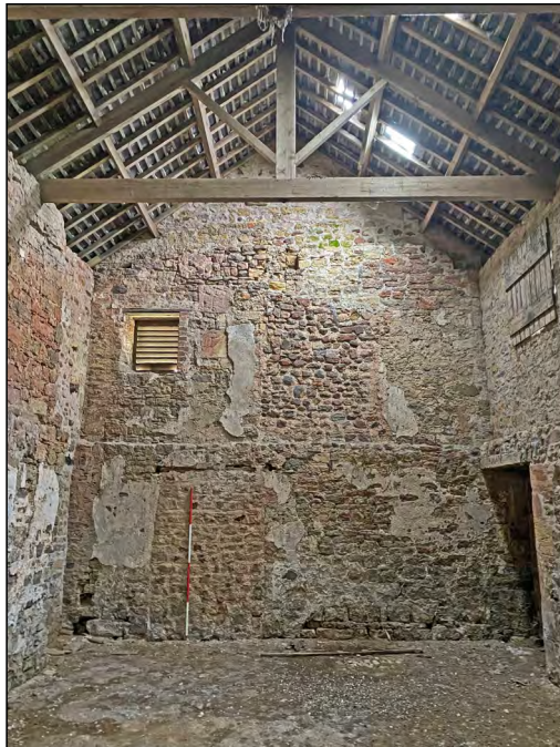
Photo 51. Internal view to the south face of the north wall of the 'Old Hall'.
