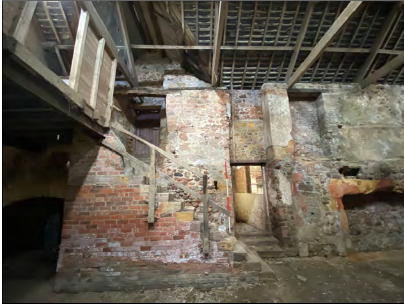
Photo 61. The S-central part of the internal face of the W wall of the 'Old Hall', with GF entrance to the E range, modern brick-built stairs providing access to first-floor level and various blocked openings at first-floor level.
