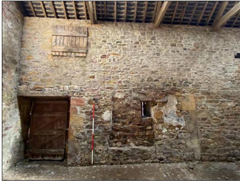
Photo 53. The north part of the internal face of the east wall of the 'Old Hall'.
