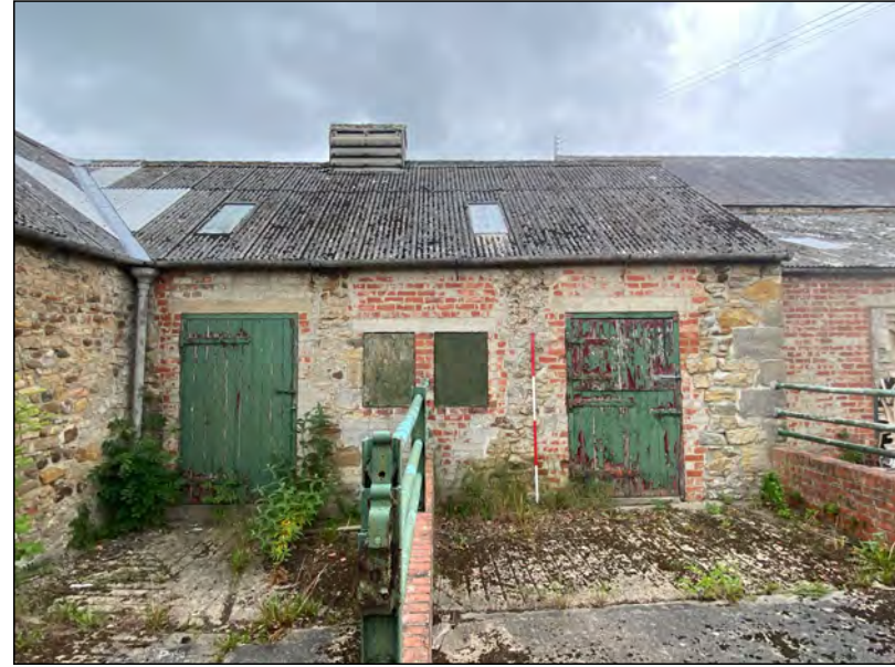
Photo 30. The original north part of the west elevation to the east range of farm-buildings.
