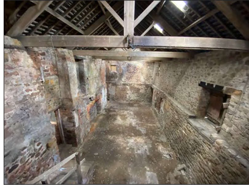
Photo 78. View north into the 'Old Hall' interior from the north end of the first-floor space.
