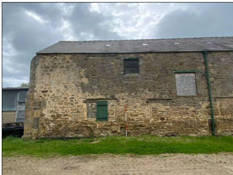
Photo 19. The south part of the east elevation of the 'Old Hall', with remains of the respond of an arch at the south end, two blocked ground-floor windows of medieval origin with another at first floor level.
