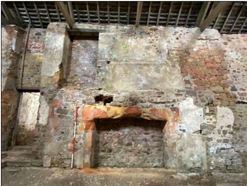
Photo 63. Fireplace in the N part of the internal (E-facing) W wall of the 'Old Hall', with blocked openings at first-floor and GF doorway to the W at right.
