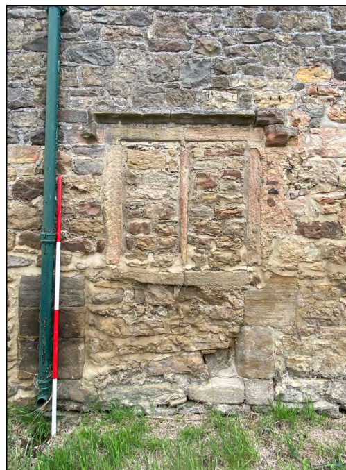
Photo 20. Blocked medieval window at ground floor level set north of centre in the east elevation of the 'Old Hall'.
