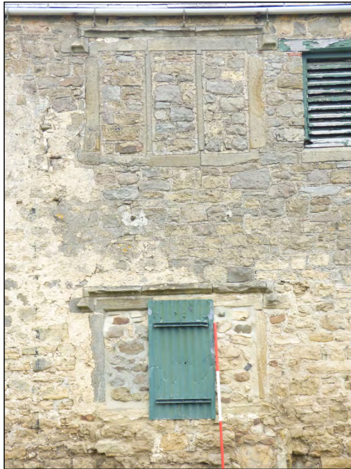
Photo 21. Blocked medieval windows at ground- and first-floor levels in the south part of the east elevation of then 'Old Hall'.
