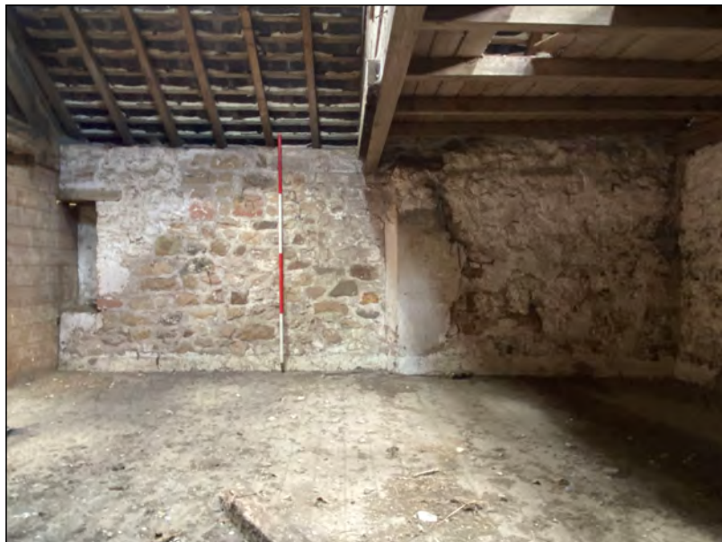
Photo 79. The west-facing internal face of the south end of the east wall at first-floor level.
