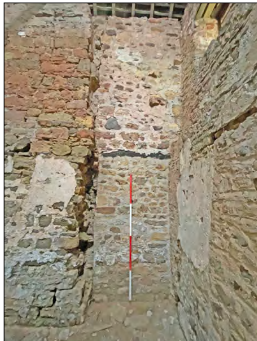
Photo 67. Blocked opening with remains of timber lintel at north end of the internal (E-facing) west wall of the 'Old Hall'.
