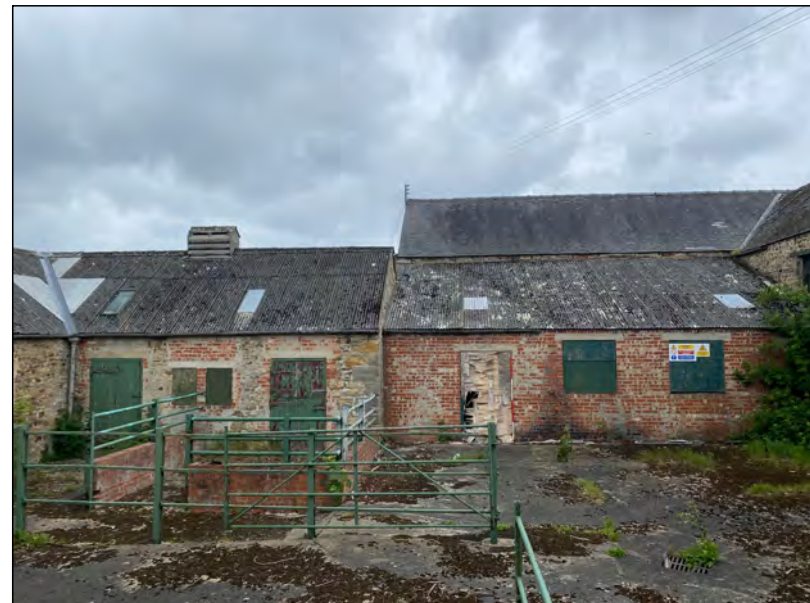
Photo 28. The west elevation of the east range of farm-buildings, comprising an original north part (left of view) and a later, lean-to addition to the north part of the west side of the 'Old Hall'.
