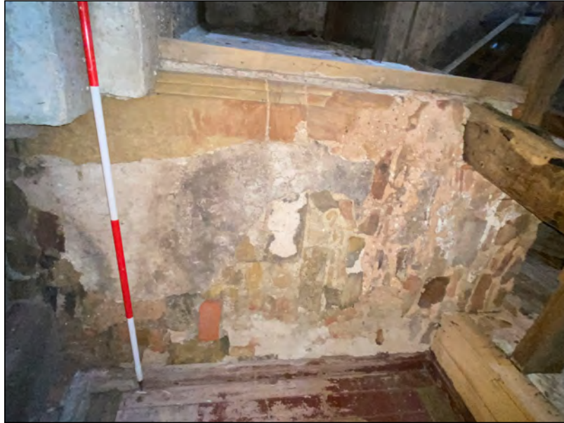
Photo 73. View SW to N-facing wall forming passage to first-floor entrance door (to adjoining the first-floor granary of the S range), formerly a fireplace marked by surviving south jamb.
