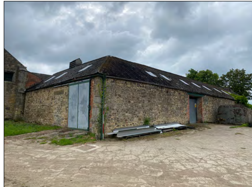
Photo 12. Oblique view from the north-east of the north elevation to the north range (right of view) and east elevation of the east range.
