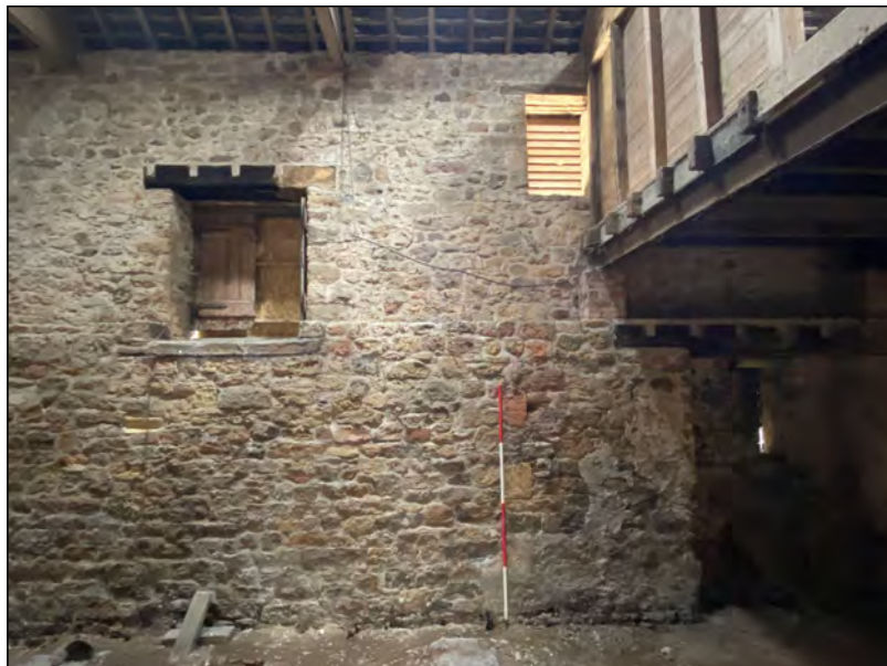
Photo 55. The south-central part of the internal face of the east wall of the 'Old Hall'.
