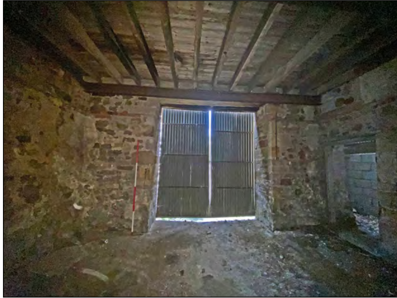
Photo 57. The internal face of the south end wall of the 'Old Hall'.
