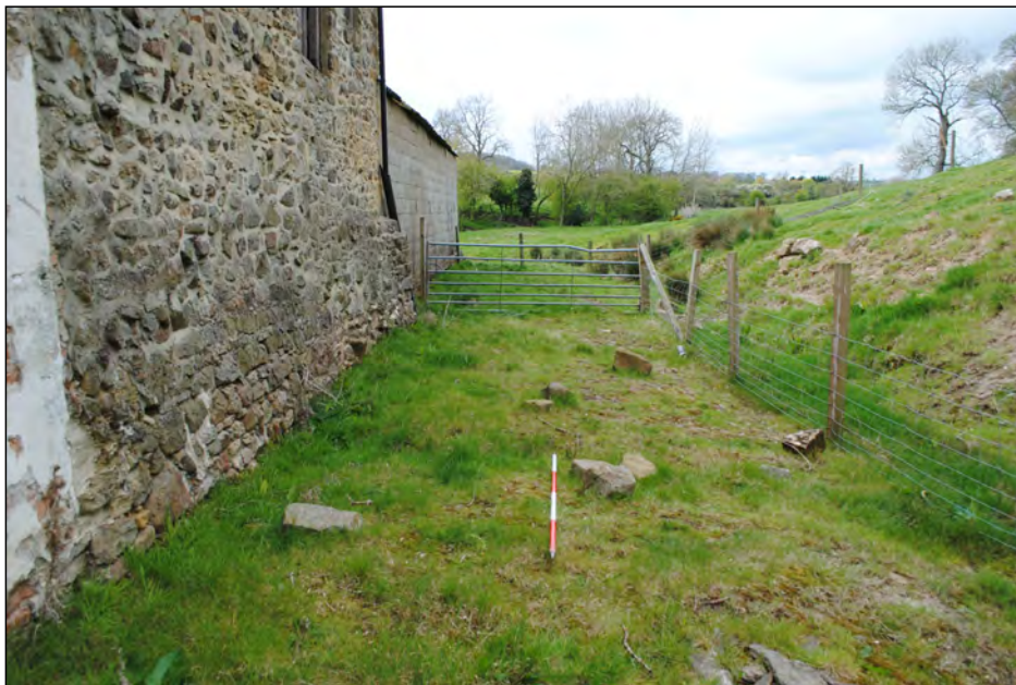
Photo 23. View looking south-west at disturbed masonry pieces alongside the north wall of the mill.
