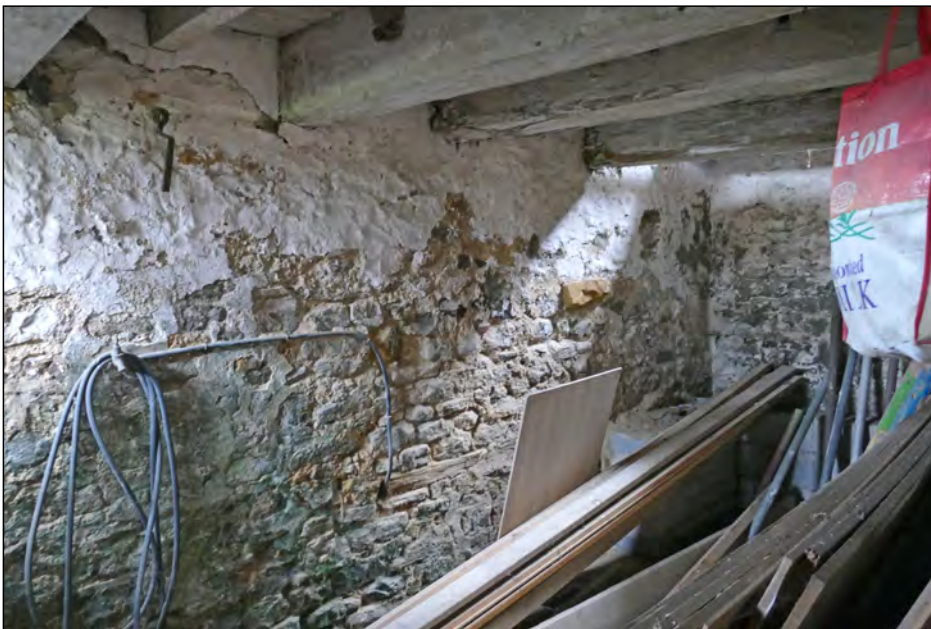
Photo 11. View looking WNW at west wall (interior) of mill, with blocked window towards centre.
