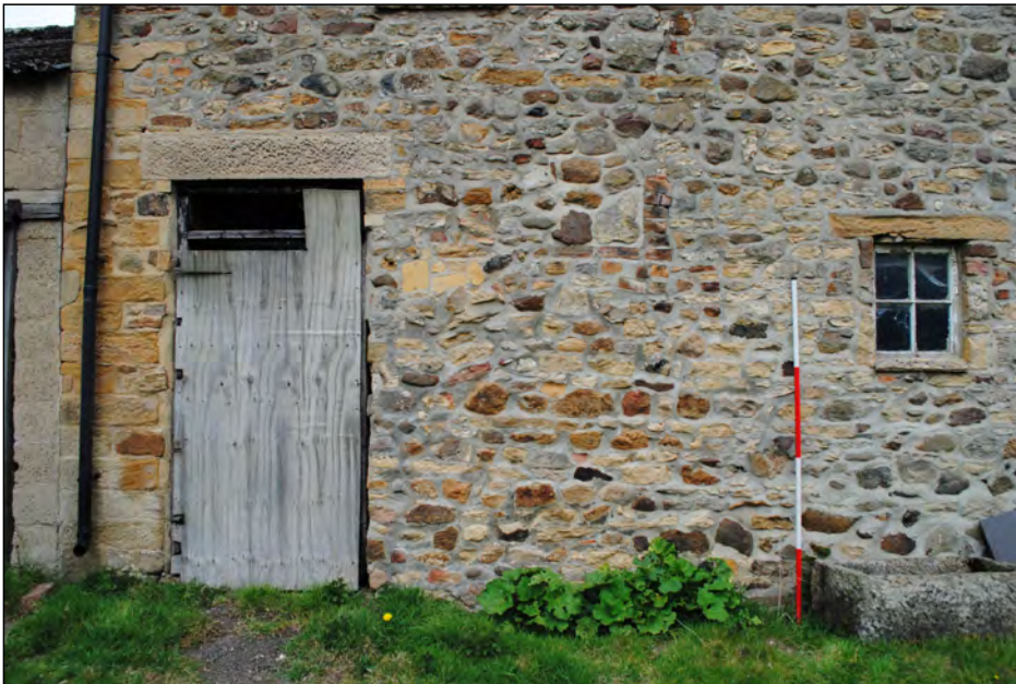
Photo 03. South-east facing elevation (lower-left portion) of the mill building, showing doorway (left) blocked window (centre) and ground floor window (right).
