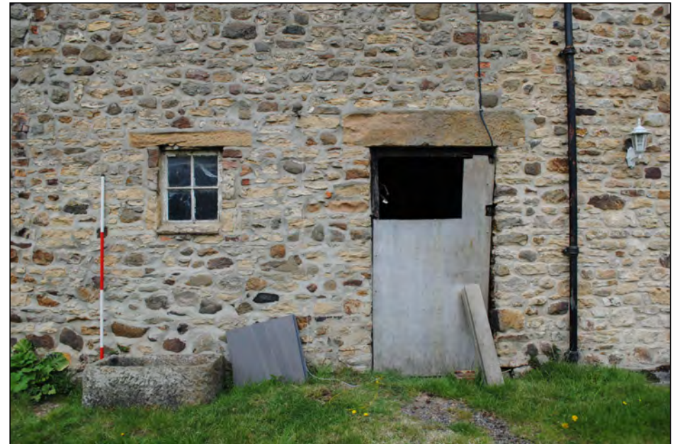
Photo 04. South-east facing elevation (lower-right portion) of the mill building, showing a second doorway (right) and ground floor window (left).
