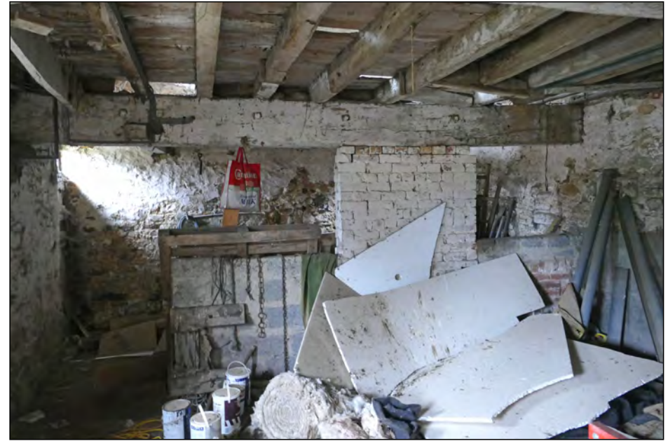
Photo 10. View looking south-west along interior of mill ground floor towards west wall.
