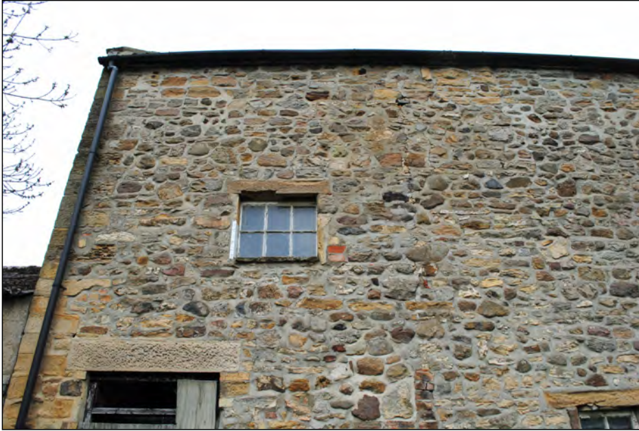
Photo 05. South-east facing elevation (upper left portion) of mill building, showing small first floor window.
