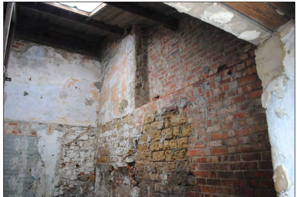
Photo 40. View looking north at interior of stable block SW end, showing significant alterations with a mixture of stone and brick in the partition wall.
