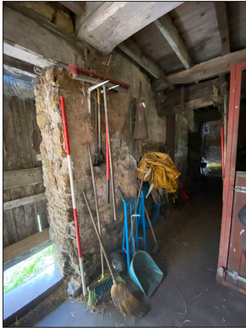
Photo 69. Mill interior view (ground floor), looking south-east towards northernmost entrance through the NE wall.
