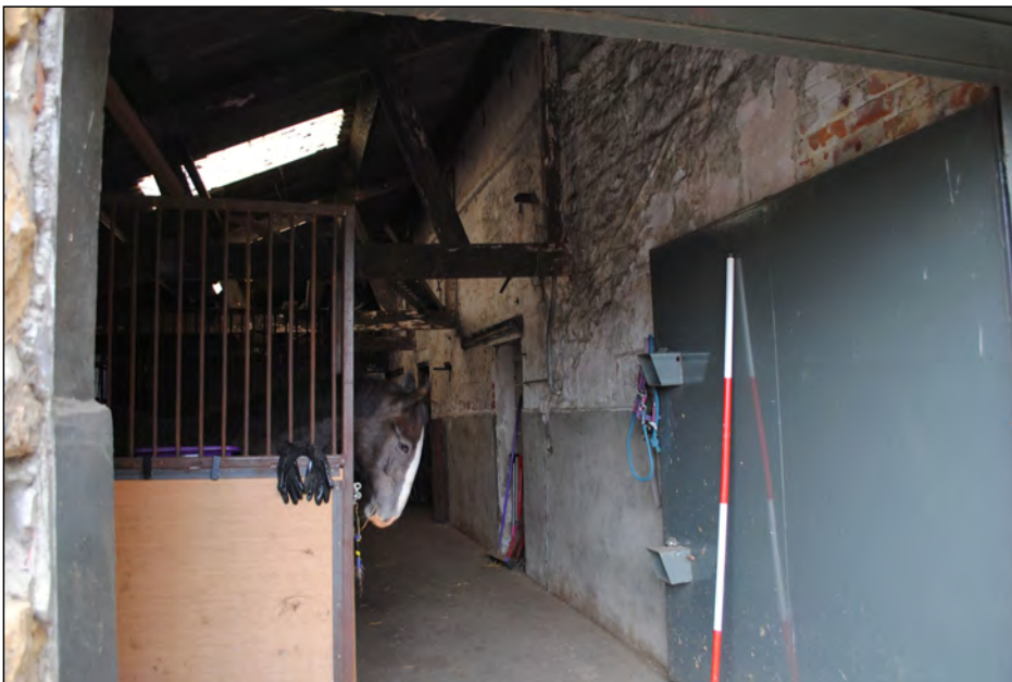
Photo 55. View looking east at the NW facing central wall (now a partition) in stable block interior.
