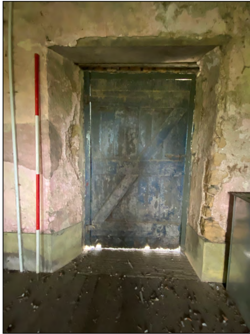
Photo 93. Mill interior (first floor), detail of doorway through the NE wall (NW end).
