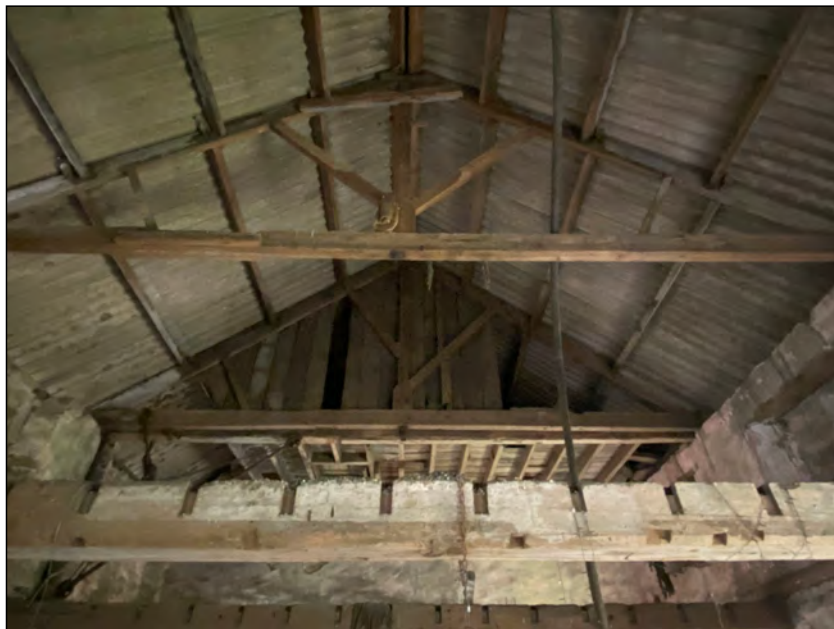
Photo 95. Mill interior, view looking south-east at roof-space and across beams to support former second floor.
