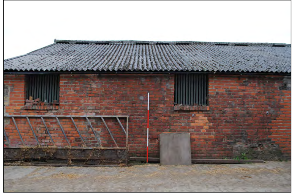
Photo 50. North-west facing elevation of stable-block, towards centre.
