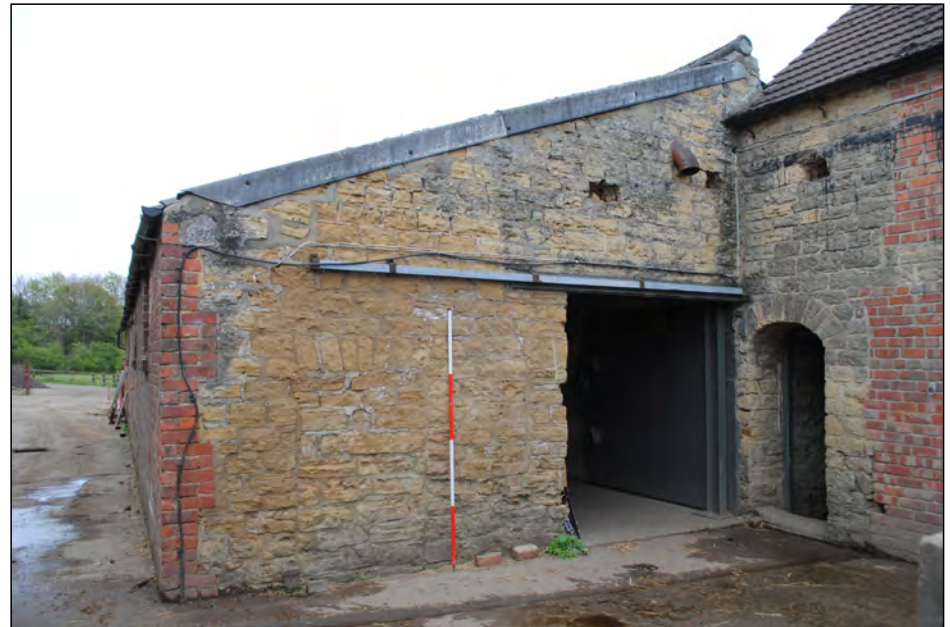
Photo 52. View looking east towards the SW gable of the stable block, partially abutting the NE wall of the cottage.
