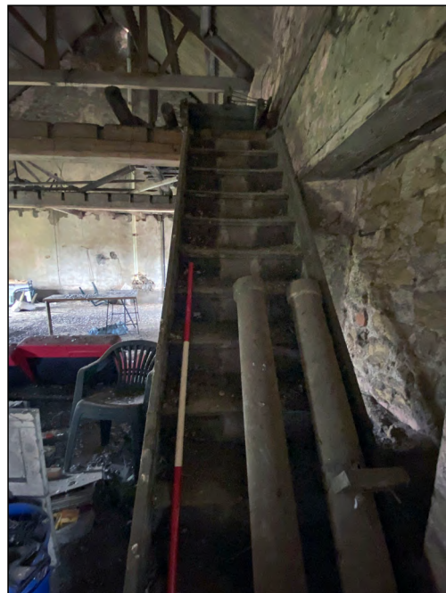
Photo 91. Mill interior (first floor), view looking north-west up stairway leading to former second floor.
