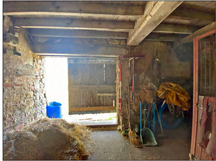
Photo 70. Mill interior view (ground floor), looking north-east towards northernmost entrance through the NE wall.
