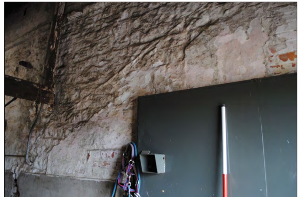
Photo 56. Detail of scar from former roof-line of structure abutting the SW end of the NW facing central (now a partition) wall within the stable block interior.
