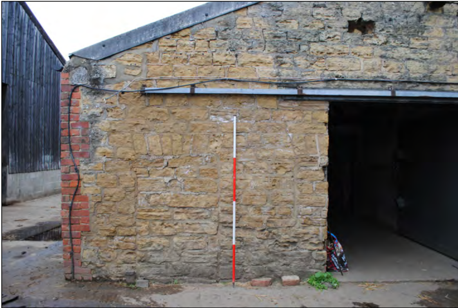
Photo 53. South-west facing elevation of stable block, left side, with detail of blocked doorway.
