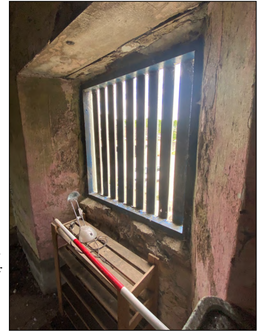
Photo 94. Mill interior (first floor), detail of slatted window through the NE wall (NW end - left of door).
