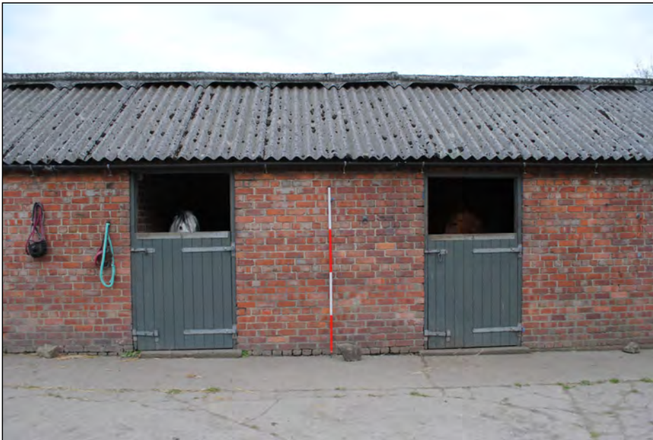
Photo 67. WNW facing elevation of modern stable block (centre area) located at the SE side of the farm complex.
