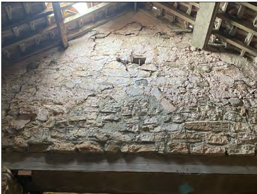
Photo 37. View looking west at detail of former window towards the apex of the west gable (internal view) in the former medieval chapel.
