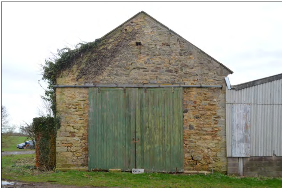
Photo 19. View of the west elevation (gable end) of the former medieval chapel.
