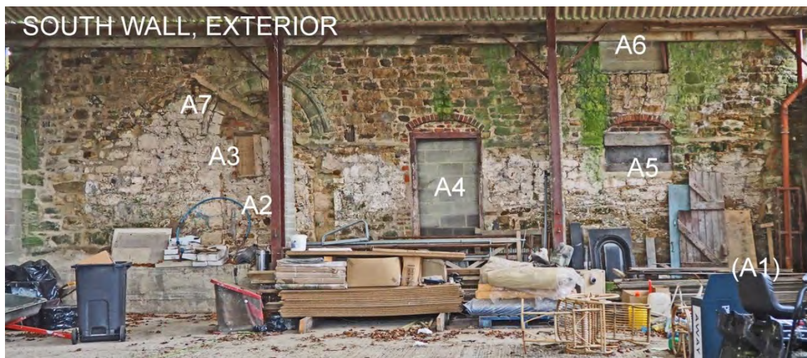
Illus. 27: Annotated photograph of the Chapel Exterior South Wall, keyed to structural inventory.
