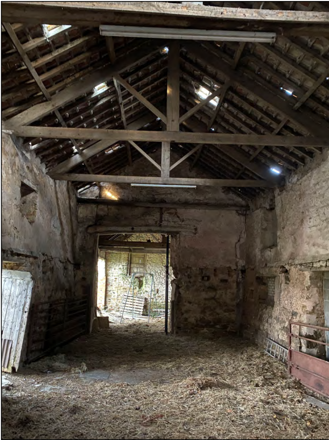
Photo 35. View looking east along the internal space of the former medieval chapel.
