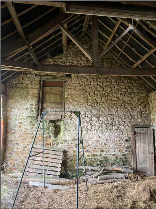
Photo 31. West facing (internal) elevation of the east wall from the Eastern Building of the North Range.
