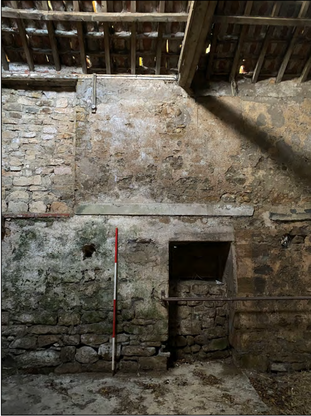
Photo 33. View looking north at blocked door & window in the north wall (internal) of the Central Building.
