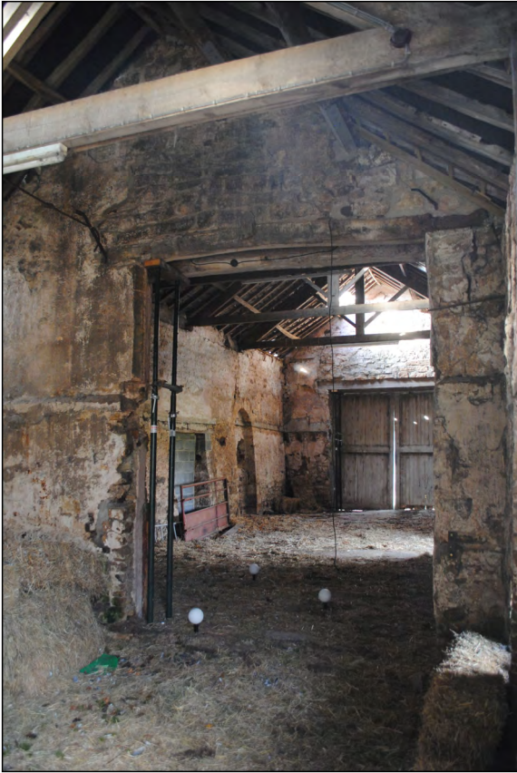
Photo 29. View looking west through the entrance in the east gable wall of the former medieval chapel.
