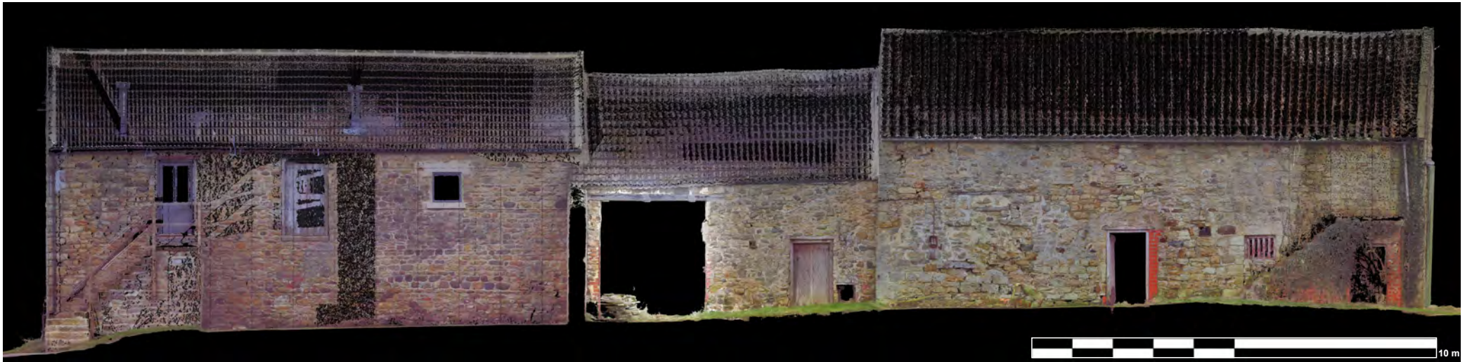
Illus. 10: Digital Scan of the north elevation of the North Range, Walworth North Farm, by Gianluca Foschi, April 2022.
