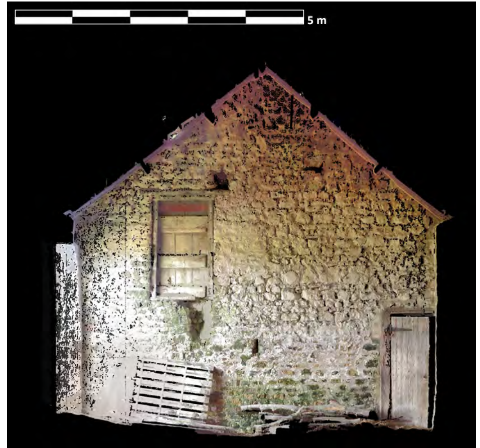
Illus. 20: Digital Scan of the internal east elevation of the Central Barn forming the intersection with the East Barn in the North Range, Walworth North Farm, by Gianluca Foschi, April 2022.
