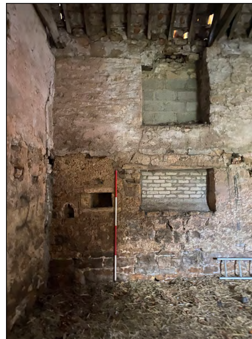
Photo 38. View looking south towards the SE corner of the former medieval chapel.
