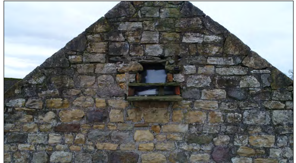
Photo 24. Detail of small window photographed in March 2022, towards the apex of the east gable of the Eastern Building, following renovation work.
