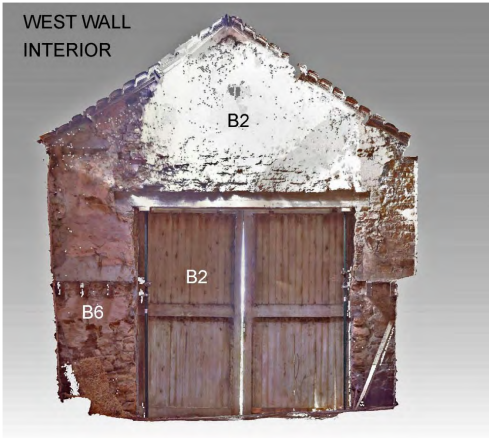
Illus. 30: Annotated photograph of the Chapel Interior West Wall, keyed to structural inventory.
