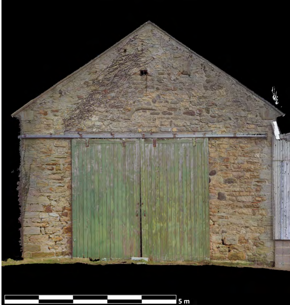
Illus. 12: Digital Scan of the west elevation of the Medieval Chapel forming the west side of the North Range, Walworth North Farm, by Gianluca Foschi, April 2022.
