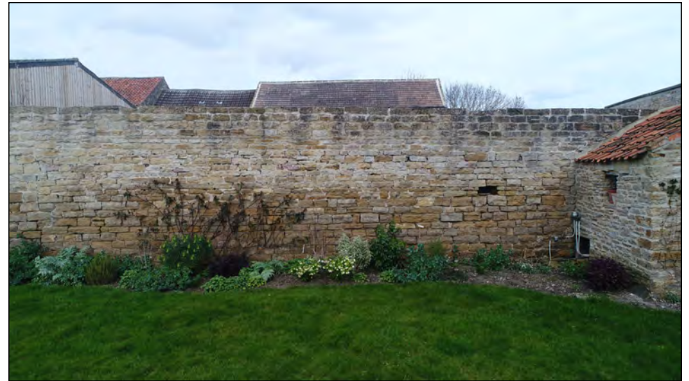
Photo 48. South wall of the outbuilding range, forming the north boundary wall of the farmhouse garden.
