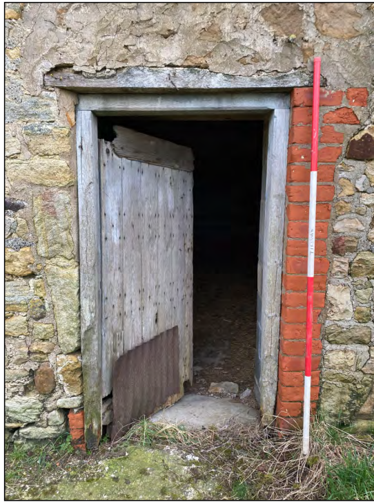
Photo 17. View looking south at doorway through the north wall in the former medieval chapel.
