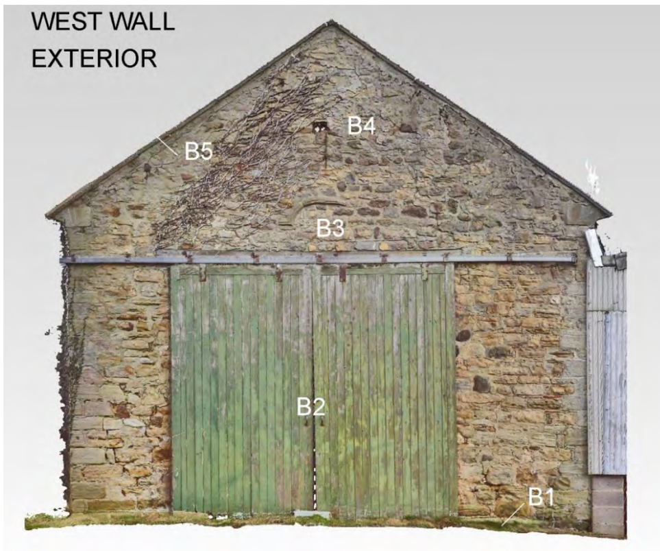
Illus. 29: Annotated photograph of the Chapel Exterior West Wall, keyed to structural inventory.
