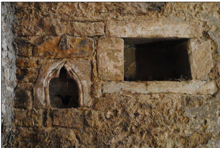
Photo 39. View looking south at detail of Piscina and Niche located at the east end of the south wall in the former medieval chapel.
