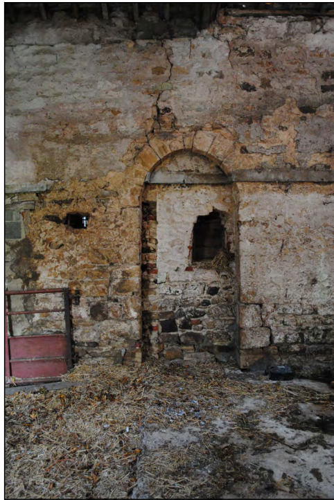
Photo 41. View looking south at original doorway (blocked) in the south wall of the former medieval chapel (internal view).
