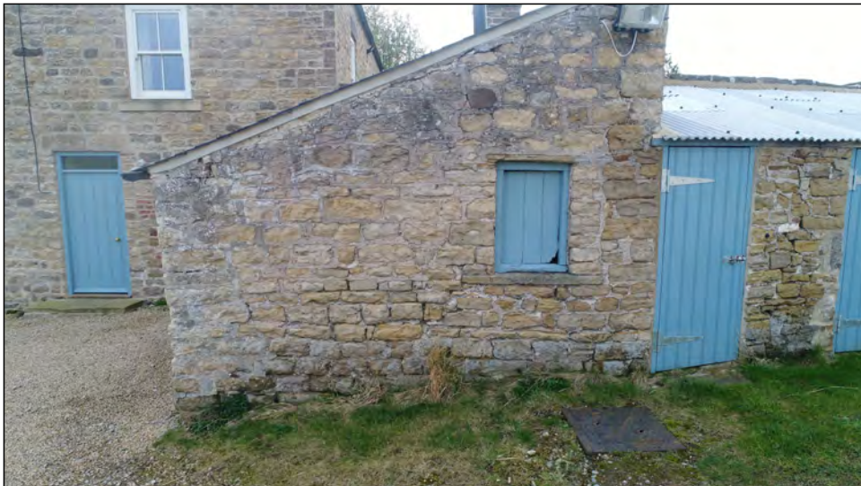
Photo 43. North facing elevation of stone building at east end of outbuilding range.
