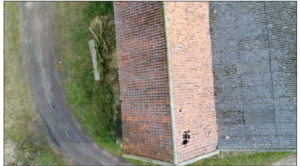
Photo 08. Vertical aerial view, looking east along the pantile roof of the former medieval chapel at North Farm.
