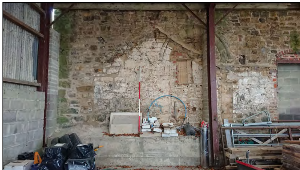
Photo 26. The west part of the south elevation in the former medieval chapel, showing original (blocked) doorway and outline scar of former adjoining structure.
