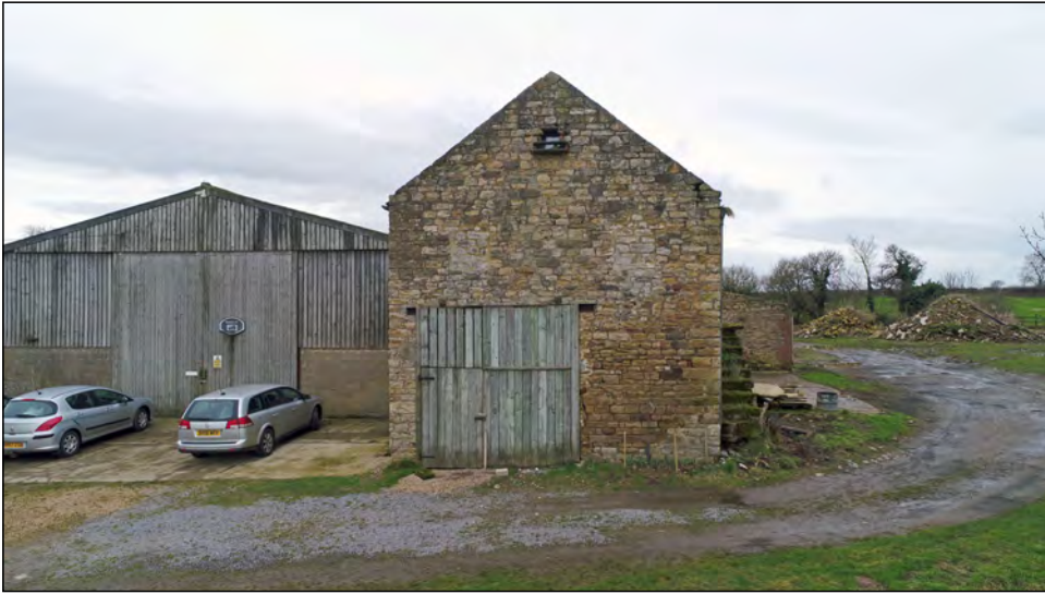
Photo 21. Wide view looking west in February 2020, at the east gable of the Eastern Building in the north range, prior to renovation work.
