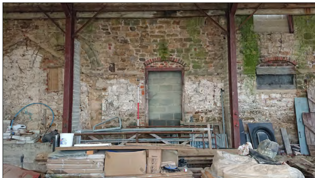
Photo 28. View looking north at central portion of the former chapel south wall, with original door (blocked) to the left, relatively modern door (blocked) in the centre, and relatively modern window (blocked) to the right.
