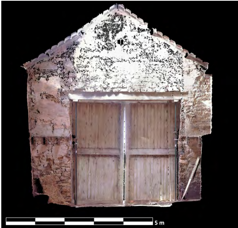
Illus. 17: Digital Scan of the internal west elevation of the Medieval Chapel forming the west side of the North Range, Walworth North Farm, by Gianluca Foschi, April 2022.
