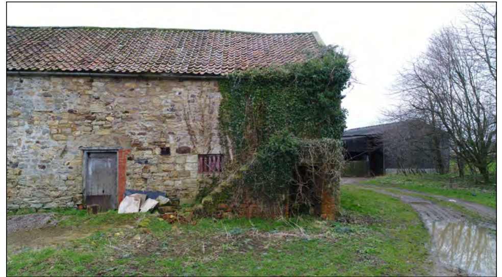
Photo 16. View looking south towards the west end of the north elevation of the former medieval chapel in the north range.
